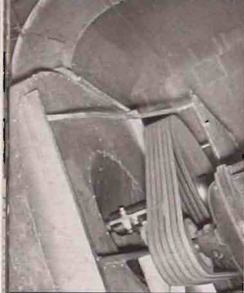
WHIRLING WHEELS BEHIND THE SCENES. SUB-BASEMENT CROWDED WITH MACHINERY FOR AIR CONDITIONING, ELEVATORS, ESCALATORS, REFRIGERATION, LIGHT, POWER, HEAT
