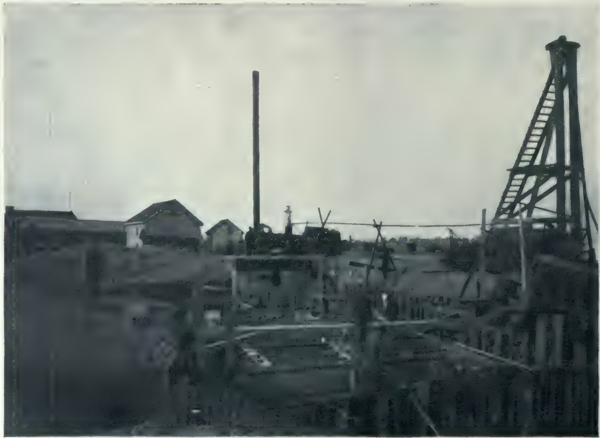
View showing construction of foundation for Low-lifting Pumping Station of Filtration Plant, now in process of installation at Centre Island, Toronto.
