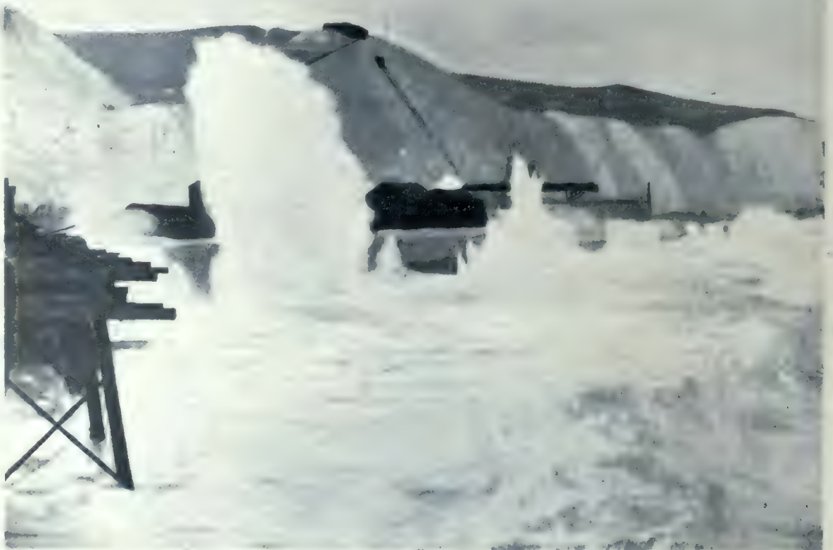
One of the many difficulties contended with in building Dover Naval Harbor. The point at which the work was carried out is one of the roughest spots of water between England and France, being exposed to all seas from east to west. In order to place the massive concrete blocks, it was necessary to erect for temporary use a ponderous wooden staging, on huge piles of a special wood brought a distance of 13,000 miles.
