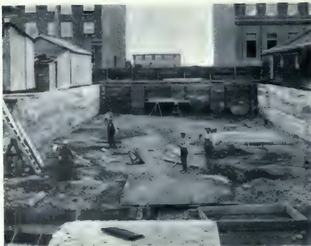
Putting in the foundation work on Eighth avenue west, Calgary, for Alderman J. S. Mackie's new five story, brick and stone, store and office building. Dowler & Michie, Architects.
