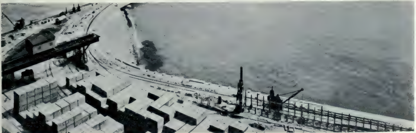
High concrete monoliths, as they were assembled prior to being placed in the walls forming the arms of the great Dover Harbor. Sixty-five thousand blocks in all were used, averaging in weight 35 tons apiece. If placed end to end, they would extend 150 miles in length, and their total weight, together with the 200,000 tons of granite used, is equal to nearly one-half of the estimated weight of the great Pyramid of Cheops.
