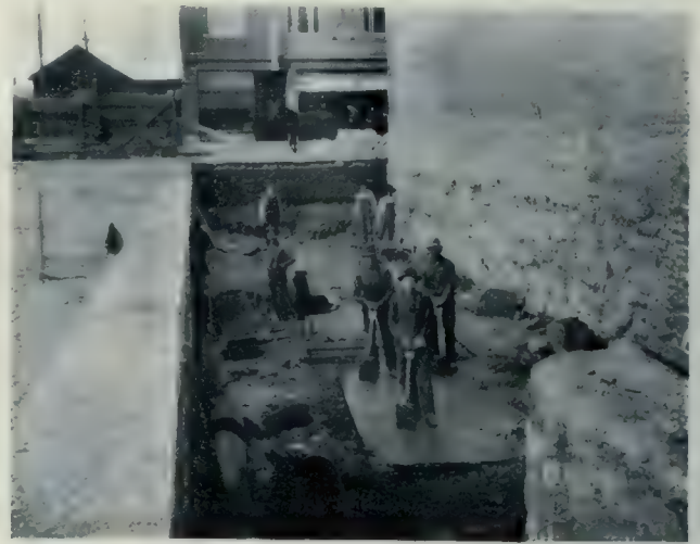
Preliminary stage in the erection of a four story brick and stone store and office building on Eighth avenue west, Calgary, for the Hon. F. A. McNaughton. Dowler & Michie, Architects.
