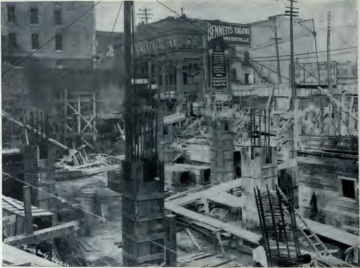
Foundation work on the new Jacobs Building, St. Catherine and St. Alexander streets, Montreal, showing the caissons and reinforcing for the concrete supporting piers. The site of the structure covers an area of 30,000 square feet and 85 piers in all were required. This view was taken on August 5th, 1909, thirteen days before the superstructure was started, and while excavation was still in progress. Mitchell and Creighton, Architects.
