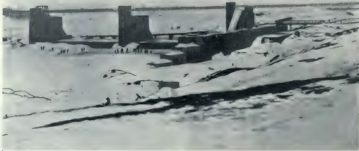
Progress view, St. Andrew's Rapids Dam, showing the stage to which the work had advanced in April, 1909. H. E. Vautelet, Consulting Engineer.
