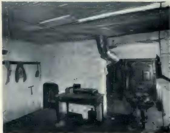
One of the "fireproof" basements in Toronto schools. It will be noted that it has not even metallic ceilings, and the furnace pipe runs directly under a wood beam above the doorway. The only protection being afforded is a piece of tin between the pipe and the beam. There is a can of oil under the table, which would contribute toward the "fireproofing" of this room.
