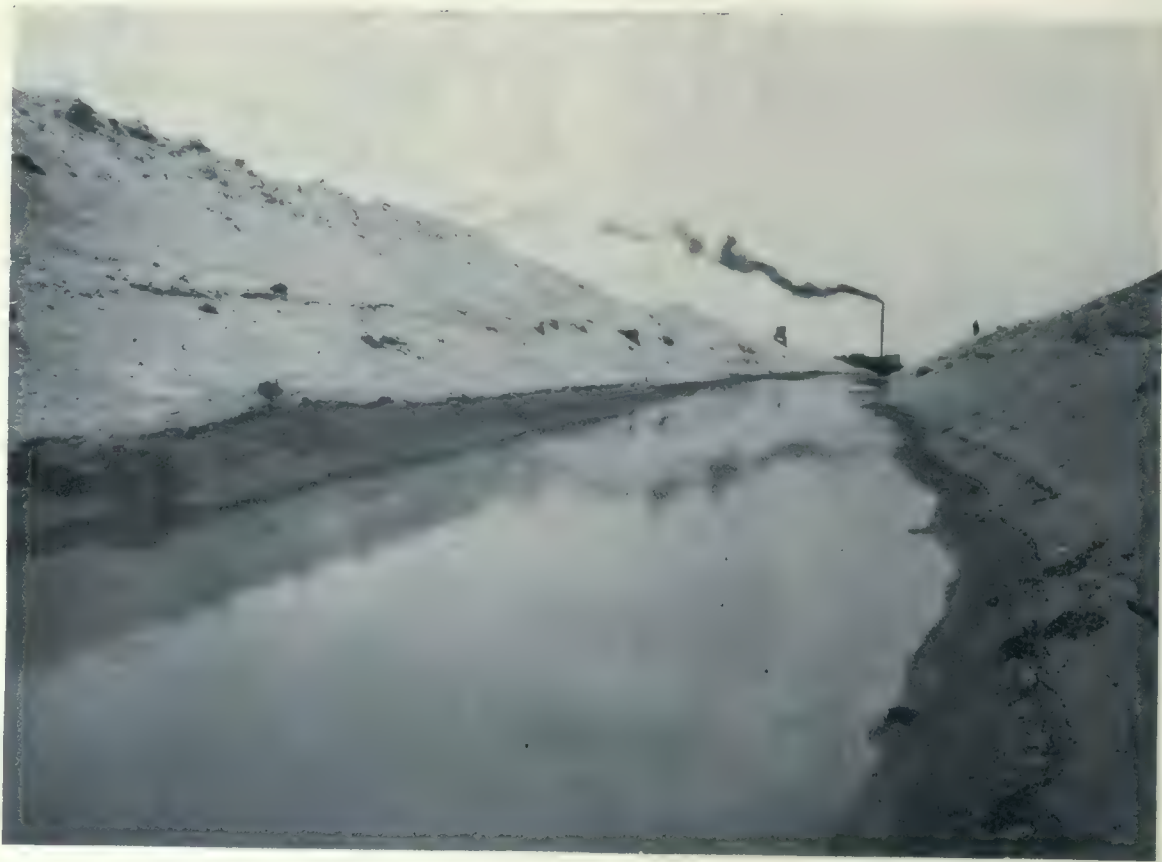
View looking along the canal with which it was necessary to surround the site of the Filtration Works so as to lower the ground water level to a point which would not interfere with the putting in of the concrete. At the head of the canal is to be seen the building housing the centrifugal pumps, which discharge 4,000 gallons of water per minute into the bay.
