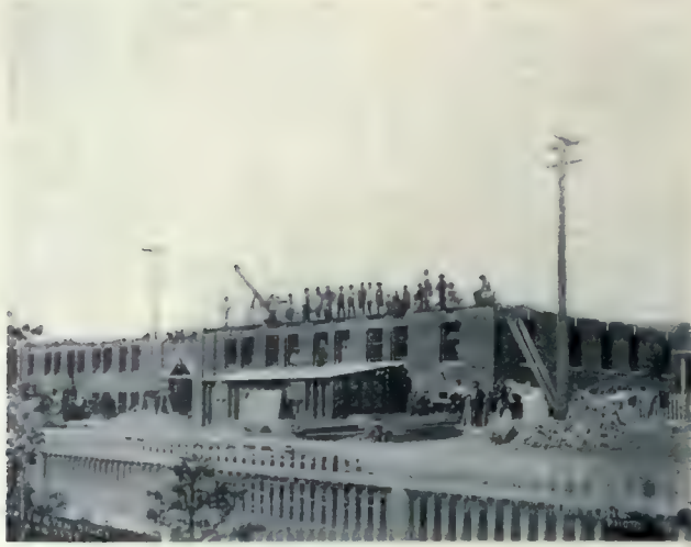
The ability of Western contractors to carry out construction work in a thorough and expeditious manner is convincingly demonstrated in the erection of the Arlington Apartments, Edmonton. This view, which gives an excellent idea of the ground dimensions of the building, shows the stage to which the work had advanced on August 25, 1909, just thirty-five days from the date the contractors undertook the removal of a cottage which originally occupied the site. R. Percy Barnes, Architect.
