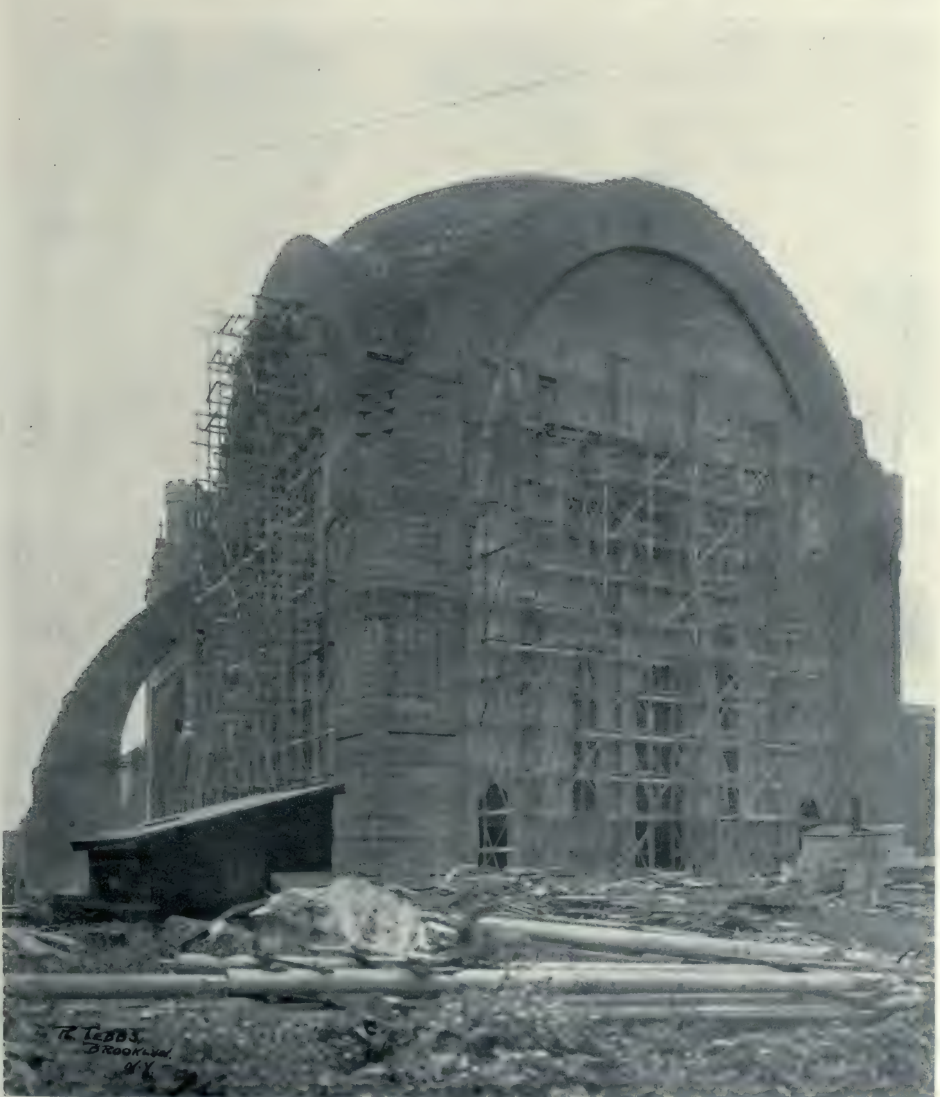
Cathedral of St. John the Divine, New York City. View showing one of the huge buttresses, the massive arches, and the great dome which rises above the centre of the structure at a distance of 200 feet from the Cathedral floor.
