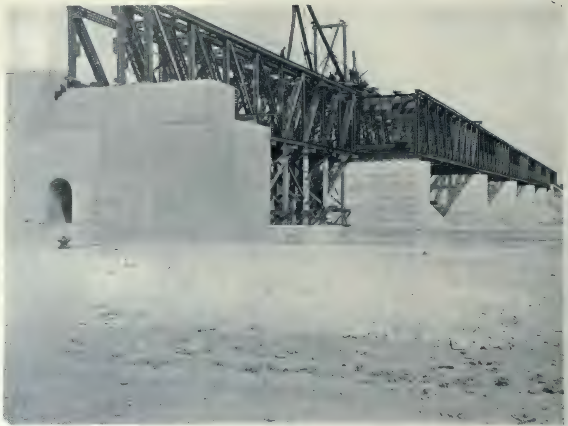
St. Andrew's Rapids Dam. View showing methods of erection, the trusses being assembled on narrow falsework, and then moved laterally into proper position on the piers. H. E. Vautelet, Consulting Engineer.
