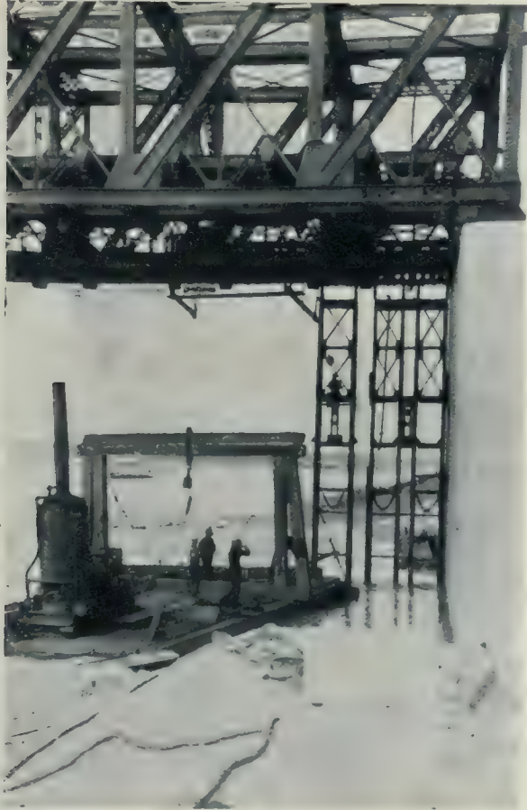
St. Andrew's Rapids Dam. View showing method of erecting girder frames. H. E. Vautelet, Consulting Engineer.
