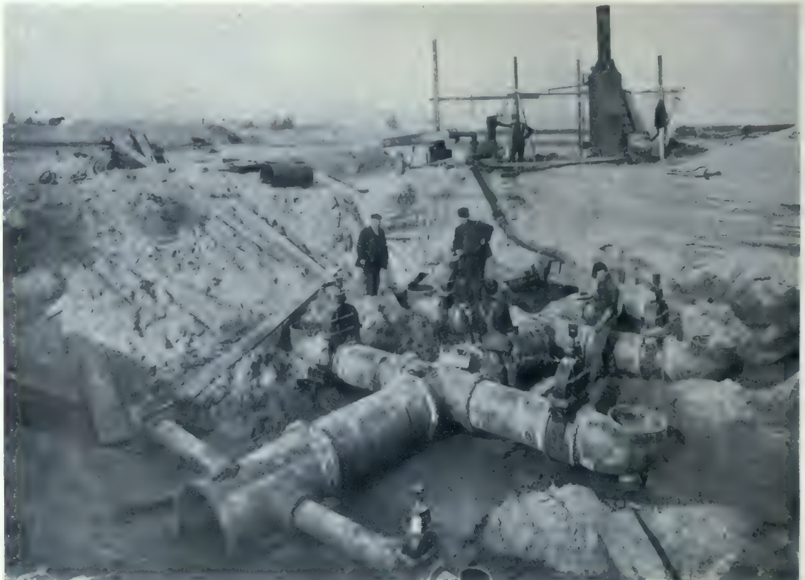
Laying the 24-inch cast iron for the Regulator Houses of Filtration Plant at Centre Island, Toronto, on either side of which are to be aligned six filter beds.
