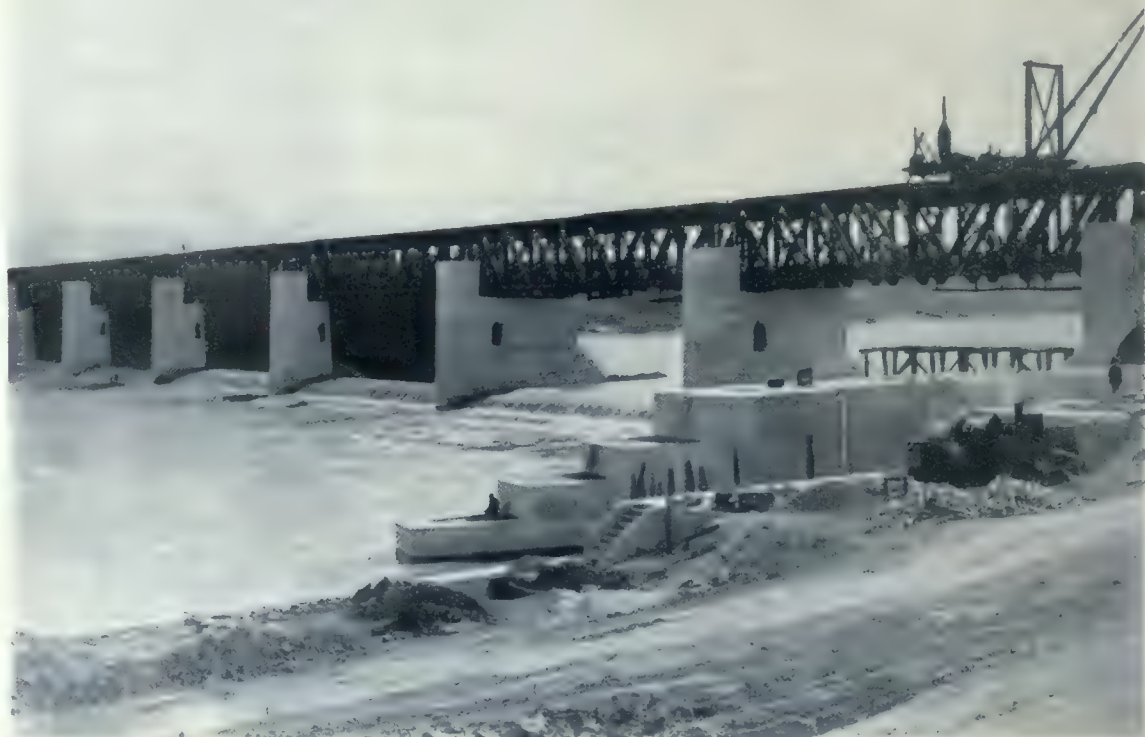
General view of St. Andrew's Rapids Dam, showing four sections of the curtain frames in place. H. E. Vautelet, Consulting Engineer.
