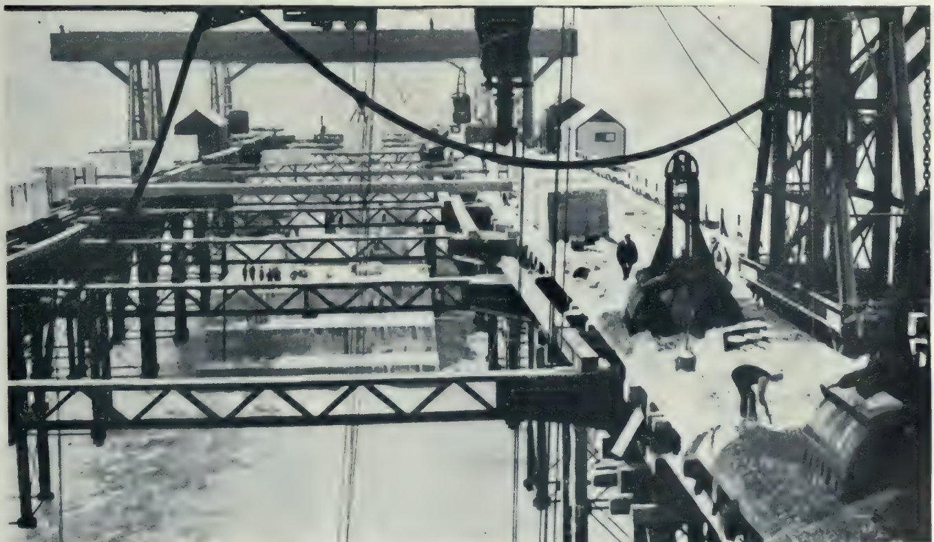
Construction work on walls of the Admiralty Pier Extension of Dover Harbor, showing the masonry through frame work, as it rises above the surface. So accurately were the blocks set below the water that when the walls appeared above the surface, they were even and regularly laid. Below the water, the blocks were not cemented, but "joggled," that is, the cylindrical cavities left between them were filled in with concrete in bags, so as to prevent the possibility of any slight lateral movement under the shock of heavy storm waves. Above the surface, the blocks were joined together in the ordinary way.
