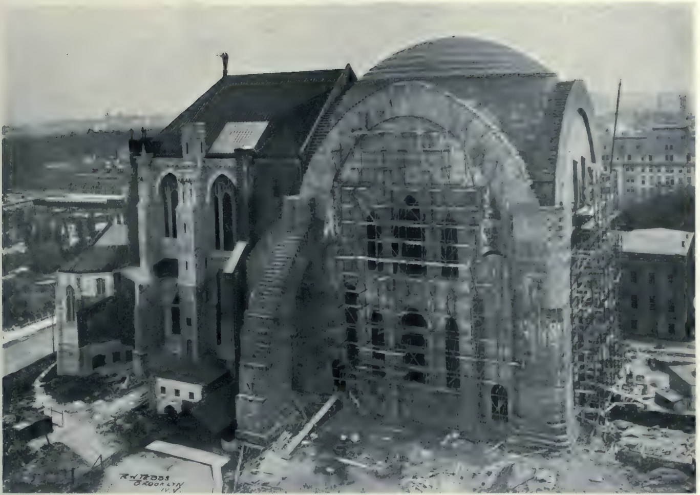
Cathedral of St. John the Divine, now in course of construction, on Morningside Heights, New York City. An idea of its great size may be obtained by comparing it with the buildings in the immediate background. Work on the Cathedral was started fifteen years ago, and, when completed, it will accommodate ten thousand worshippers.
