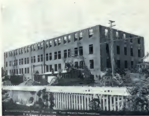
Process view of Arlington Apartments, Edmonton, taken on September 4th, 1909, showing the work five weeks after the concrete foundation was installed. R. Percy Barnes, Architect.
