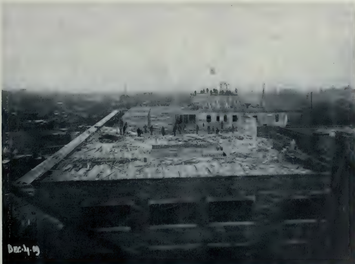
View of new Jacobs Building, Montreal, taken on December 4th, showing the building practically enclosed, and also the superstructure or seventh floor, which will eventually cover the entire area of the building and form a portion of the future extension of four floors provided for in the design and construction of the building. Mitchell and Creighton, Architects.
