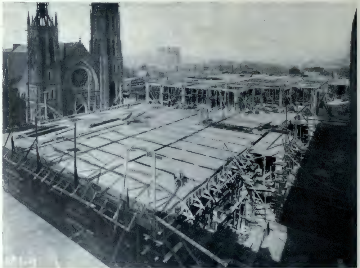
View of the new Jacobs Building, Montreal, taken on October 9th, showing the construction of superstructure. The foreground shows the finished centering ready for concreting, and the background the form work in course of erection for the next floor. The large building under course of erection in the distance, is another modern business structure which is being built according to the same system of construction. Mitchell and Creighton, Architects.
