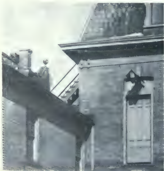
The only fire escape on a Toronto school building; a wooden affair that runs down from the third story of the York Street School to the roof of another building. This was erected about the time of the Collinwood disaster.
