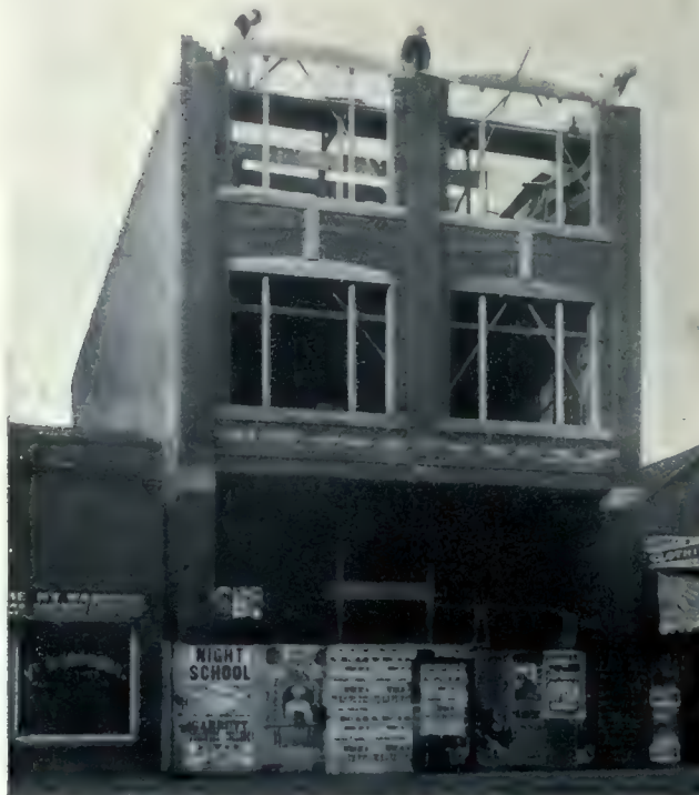
Business building for Bailey Bros., now being built on Eighth avenue east, Calgary, at a cost of $16,000. Dowler & Michie, Architects.
