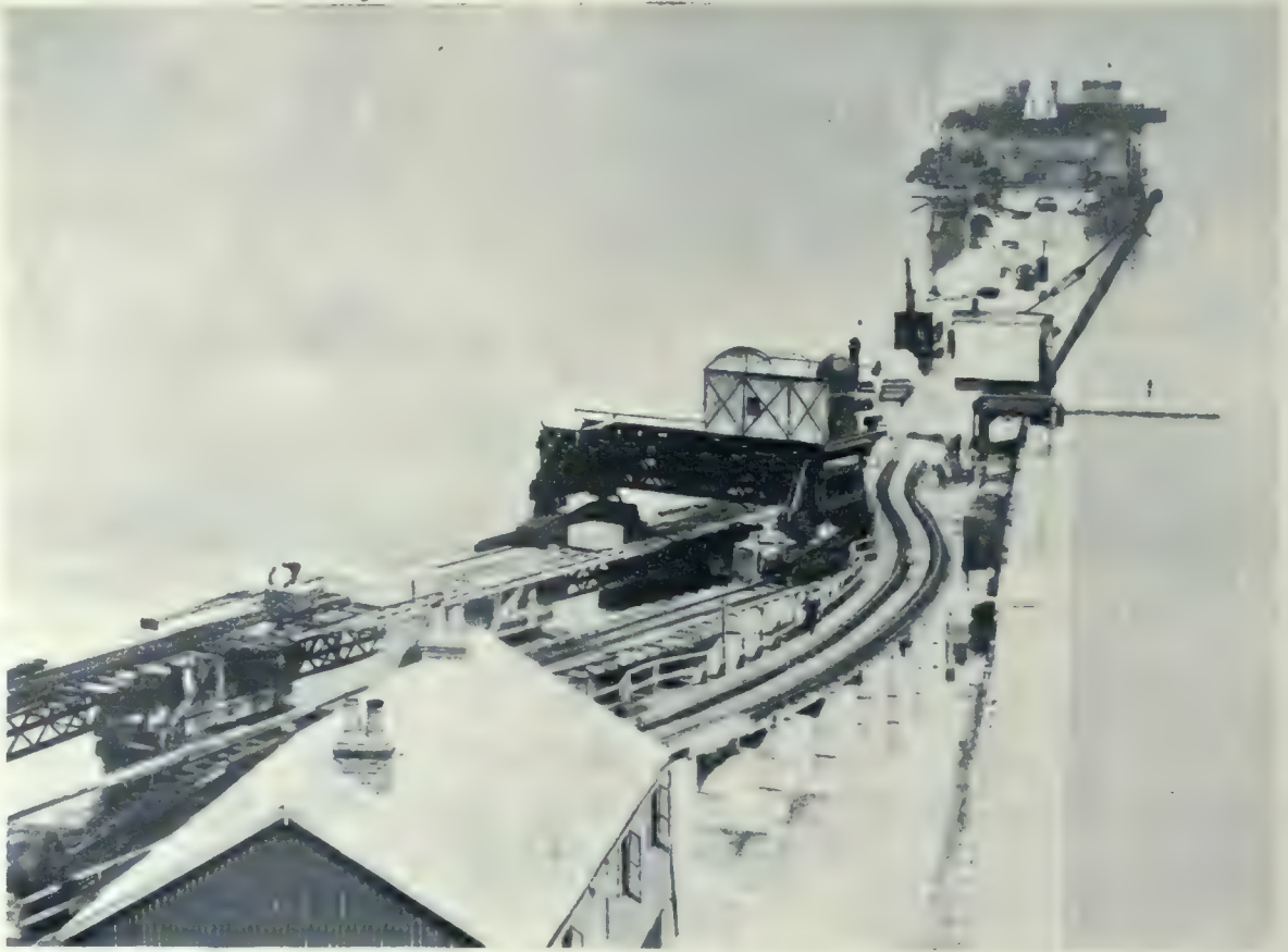
Admiralty Pier Extension of Dover Harbor, as it appeared in course of construction. The work on this extension consisted in carrying the old Admiralty Pier, which was 1,000 feet long, some 2,000 feet further out into the sea. It is the shortest of the three outer walls, the south breakwater, or centre wall, being 4,200 feet, and the east arm 3,320 feet.
