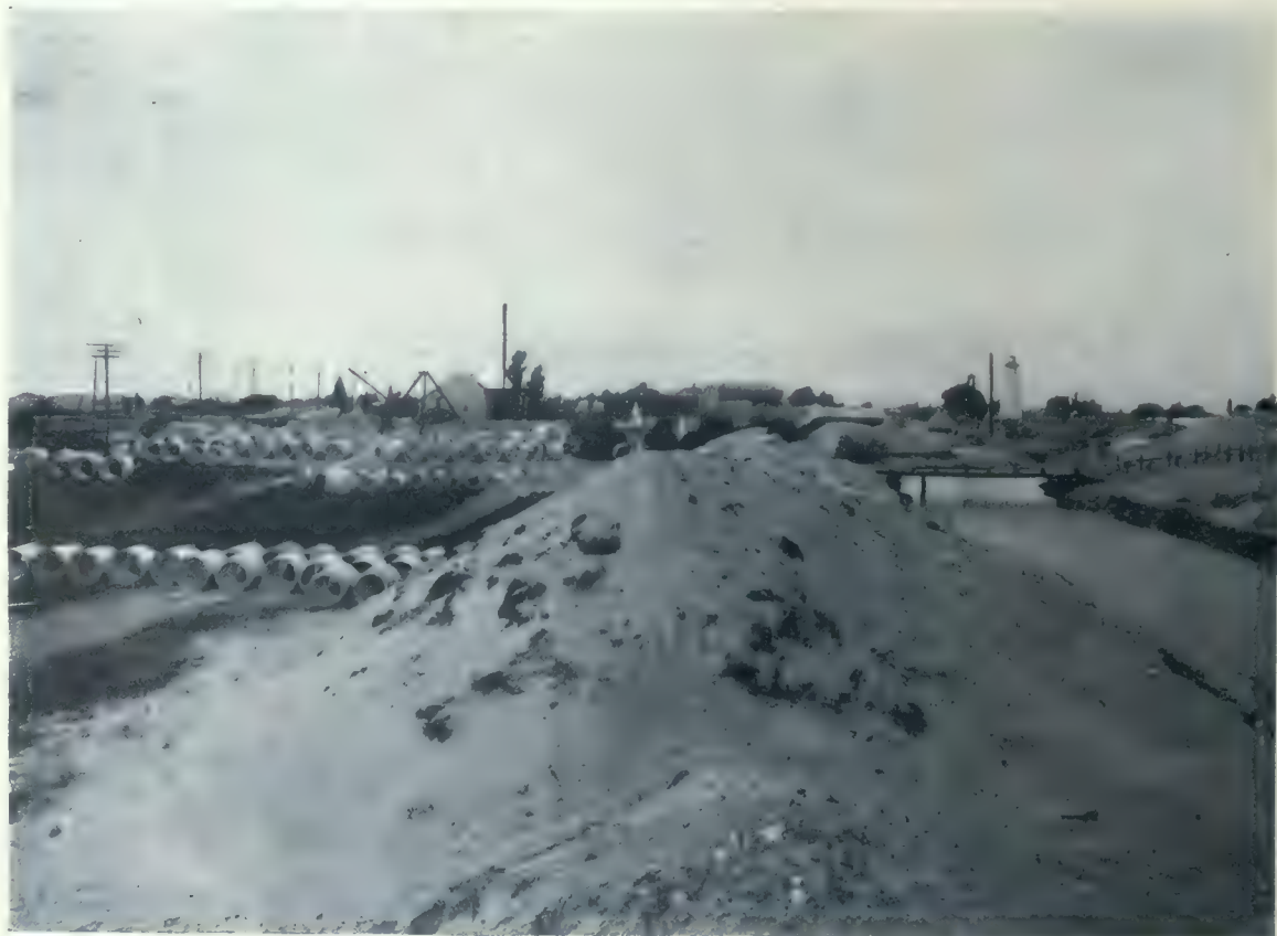
View showing sections of the huge concrete pipes which will form the conduits through which the raw and filtered water will flow. The manner of laying and locking the joints of these pipes will be one of the most interesting processes of the work.
