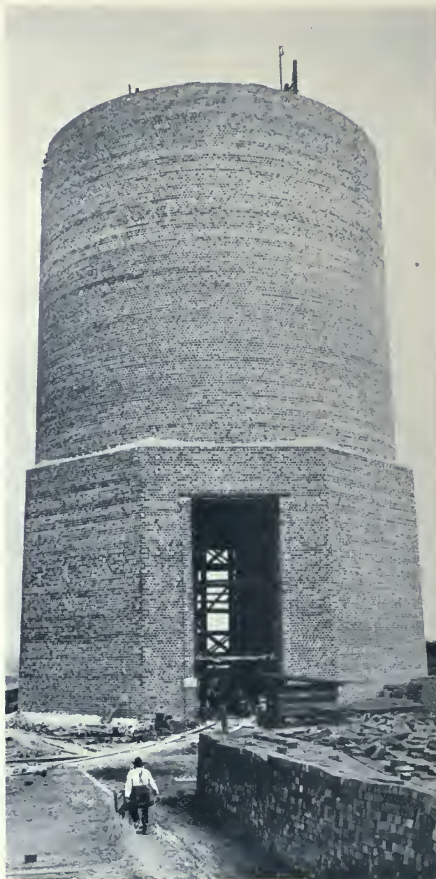
VIEW OF CHIMNEY IN PROCESS OF ERECTION, SHOWING THE LARGE FLUE OPENINGS IN ITS BASE. THE EXTERIOR AND ACID-PROOF LINING BRICKS USED IN ITS CONSTRUCTION, WERE MADE ON THE GROUNDS BY THE CONTRACTING ENGINEER.
