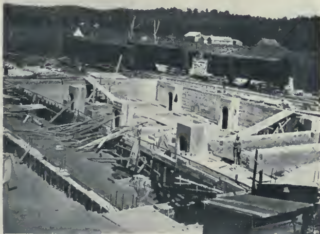
PLANT OF WOOD PRODUCTS COMPANY—VIEW SHOWING FOUNDATION OF OVEN HOUSE WITH DIVIDED FOOTING FOR THE SIX CENTRE COLUMNS. THE DIVIDED FOOTING WERE MADE NECESSARY TO PROVIDE A PASSAGE FROM ONE SIDE OF THE OVEN HOUSE TO THE OTHER. E. D. PITT, DESIGNING AND CONSTRUCTING ENGINEER.
