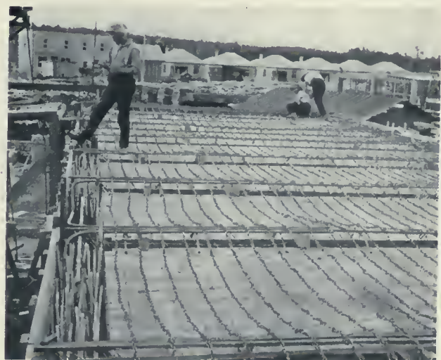
PLANT OF WOOD PRODUCTS COMPANY—VIEW SHOWING STEEL CHAIN FABRIC ON THE TANK FLOOR OF STILL HOUSE, USED IN CONNECTION WITH THE NIAGARA BAR FOR BEAMS. THIS FLOOR WAS FIGURED FOR 400 LBS. UNIFORM LIVE LOAD; IT IS NOW LOADED TO OVER 50 TONS CONCENTRATED LOAD, AND THERE IS NO APPARENT DEFLECTION AND IT IS IN PERFECT CONDITION. E. D. PITT, DESIGNING AND CONSTRUCTING ENGINEER.
