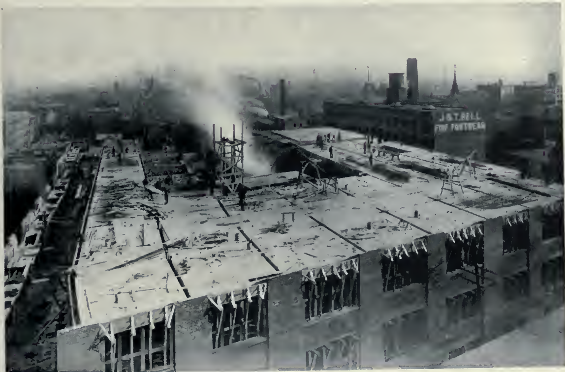
AMES-HOLDEN BUILDING, MONTREAL, SHOWING REINFORCED CONCRETE FLOOR WORK IN PROCESS OF CONSTRUCTION. IT WILL BE NOTED THAT THE FLOOR SUSTAINING EXTERIOR WALLS ARE CONSTRUCTED SIMULTANEOUSLY WITH THE CONCRETE FRAMEWORK OF THE BUILDING. ROSS & MACFARLANE, ARCHITECTS.
