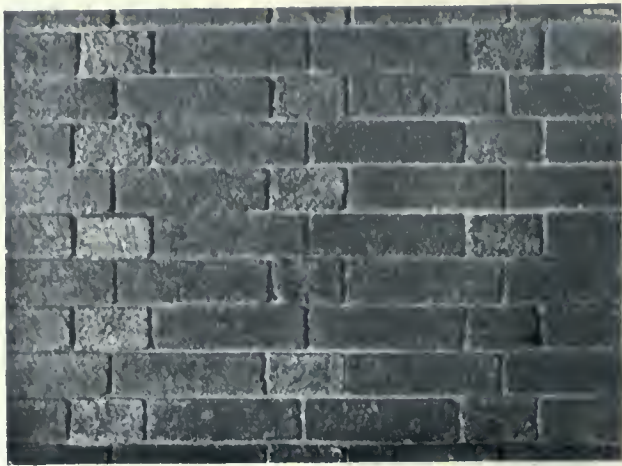
Fig. 7.—Another example of the double stretcher Flemish bond, only here the mortar joints are much thinner, being but one-eighth of an inch in thickness and slightly raked-out. The bricks used are 8 x 2½ x 3¾ inches in size, and of a rough texture; the stretchers being of dark clear red, and the headers of a brown blue color.
