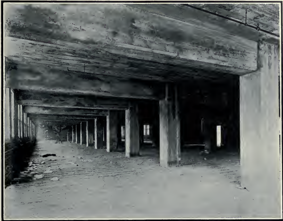
View of one of the floors, new Southam Building, Toronto, prior to applying the finishing coat or laying the hardwood super-floor. Messrs. Sproatt & Rolph, Architects.
