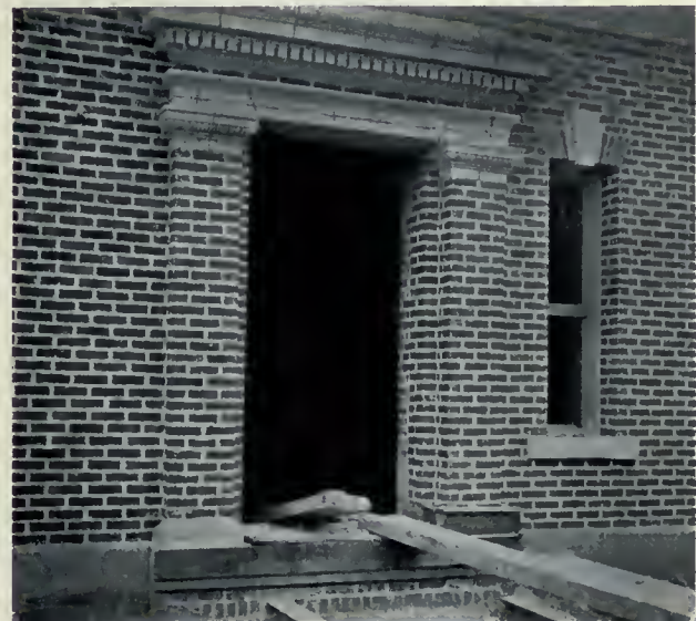
Fig. 5.—Detail of doorway of boiler house, illustrating the running or plumb bond, a bond common in a large number of buildings throughout the country. The bricks used in the structure are of varying shades, and the joints are half an inch thick, of gray color, cut rough and flush.
