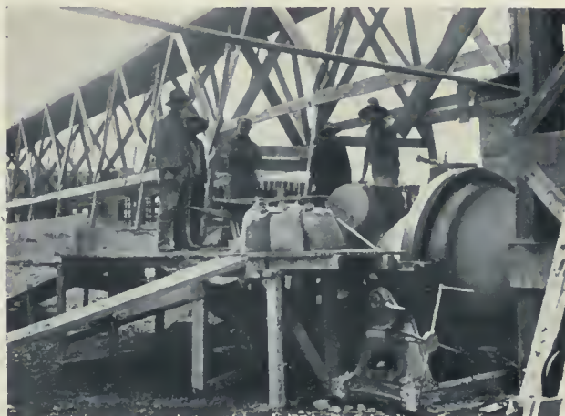
PLANT OF WOOD PRODUCTS COMPANY—SHOWING THE NO. 21-2 SMITH MIXER THAT WAS USED ON THE JOB, ALSO THE 125-FOOT RUNWAY FROM HOIST PLATFORM TO CHARCOAL HOUSE. E. D. PITT, DESIGNING AND CONSTRUCTING ENGINEER.
