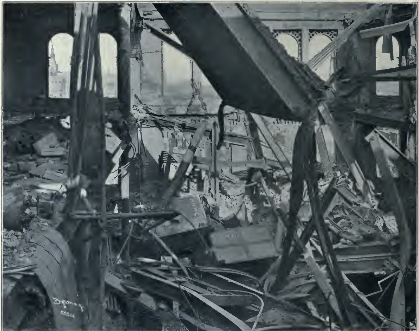
ANOTHER VIEW OF DESTROYED BUILDING, SHOWING HOW COMPLETELY THE STRUCTURE WAS WRECKED. THE TWO SAFES WHICH ARE SEEN FELL FROM THE UPPER STORIES.
