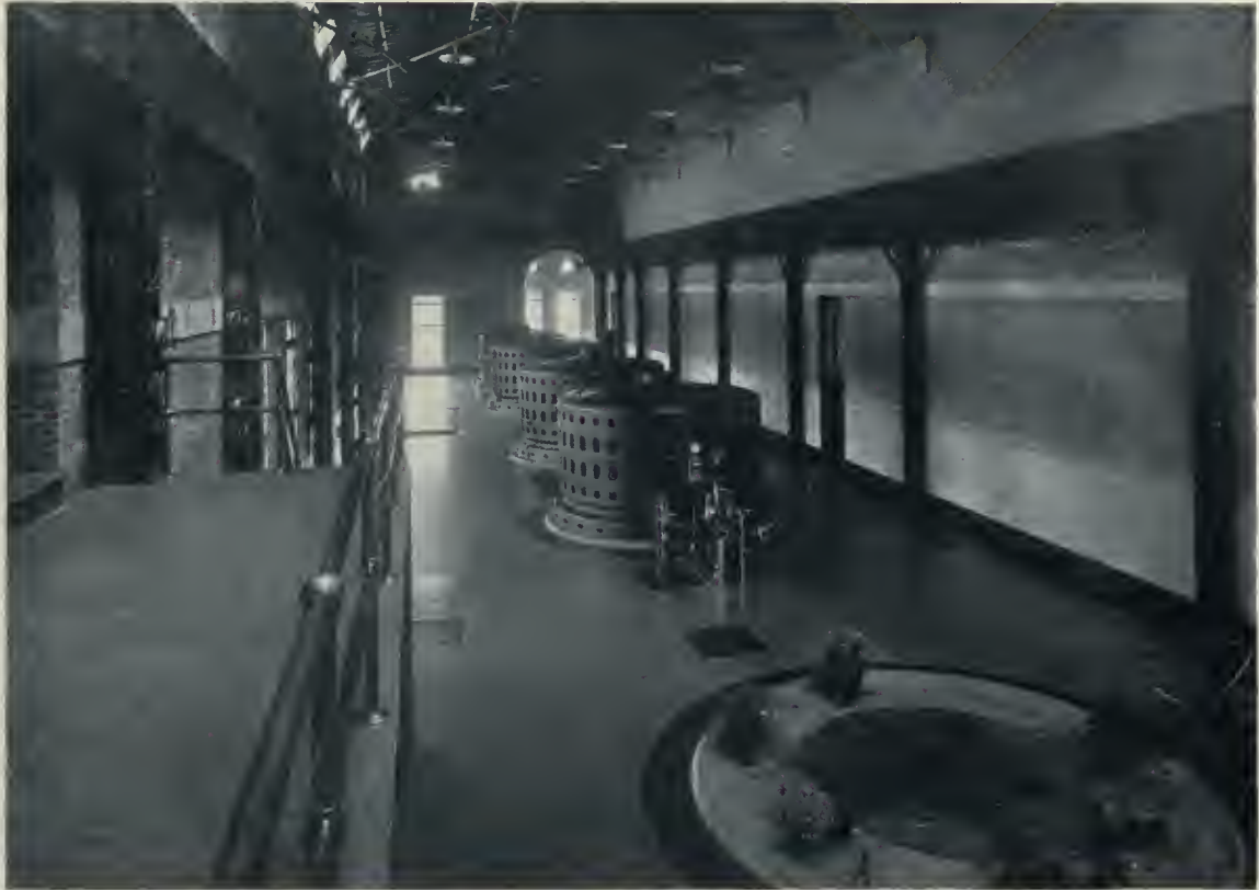
View of Generating Room, power plant of the Electrical Development Company, Niagara Falls, Ont., showing four 8,000 kilowatt generators. E. J. Lennox, Architect.
