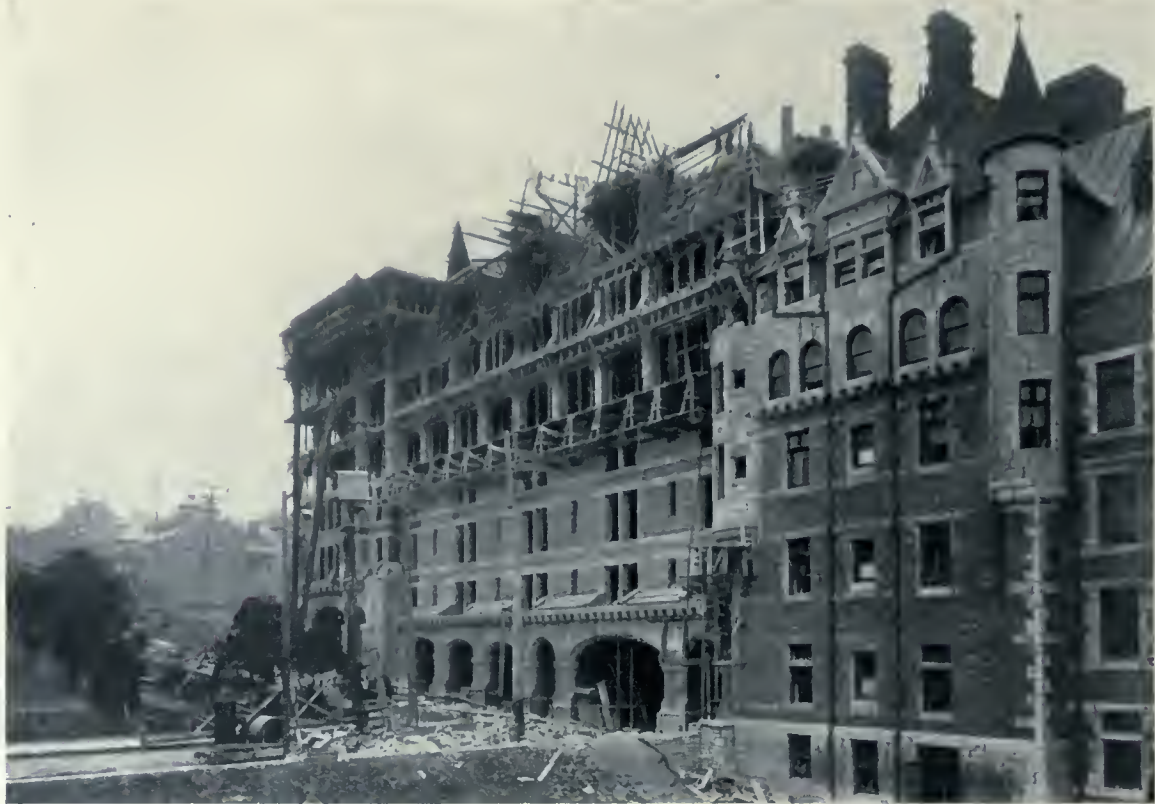
NEW ADDITION TO CHATEAU FRONTENAC, QUEBEC CITY. VIEW TAKEN OCTOBER 1ST, SHOWING THE EXTERIOR OF THE LOWER PORTION OF THE BUILDING FINISHED, AND THE FORM WORK OF THE ROOF IN COURSE OF PREPARATION. NOTE THE MANNER OF MAKING THE CONNECTION BETWEEN THE OLD AND NEW PART, THE GENERAL TREATMENT EFFECTING A PERFECT ASSIMILATION. W. S. PAINTER, ARCHITECT.
