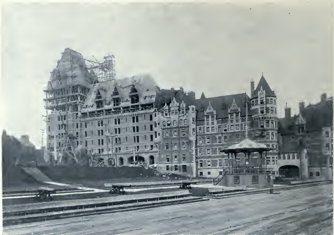
NEW ADDITION TO CHATEAU FRONTENAC, QUEBEC CITY. VIEW TAKEN OCTOBER 31ST, AT WHICH TIME THE CONCRETE PORTION OF THE BUILDING HAD BEEN FINISHED. THE ONLY EXTERIOR WORK WHICH REMAINED TO BE DONE BEING THE CURTAIN WALL OF THE UPPER PORTION. W. S. PAINTER, ARCHITECT.
