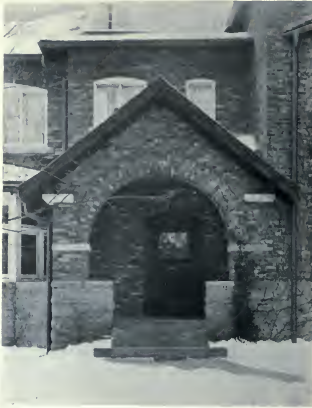
Entrance porch, clinker brick residence, Toronto, showing detail of arch and brick work. Mr. Eden Smith, Architect.
