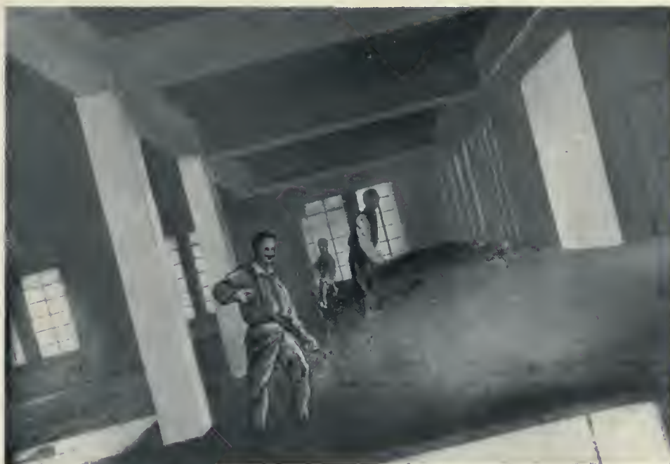
INTERIOR VIEW OF WAREHOUSE, TUNIS, AFRICA, SHOWING WORKMEN EXCAVATING UNDER HIGH SIDE SO AS TO PERMIT THE BUILDING TO SETTLE TO A VERTICAL POSITION.
