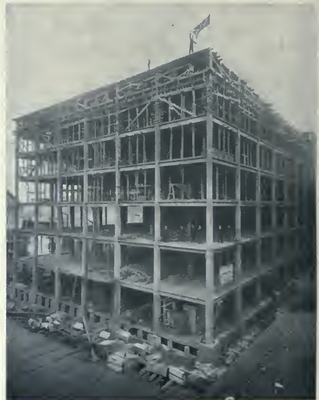
VIEW SHOWING STRUCTURE TWO MONTHS AND A HALF AFTER EXCAVATION WAS MADE, FLOORS, ROOF AND STRUCTURAL WORK COMPLETED, LYMAN SONS AND COMPANY'S BUILDING, MONTREAL. MITCHELL AND CREIGHTON, ARCHITECTS.
