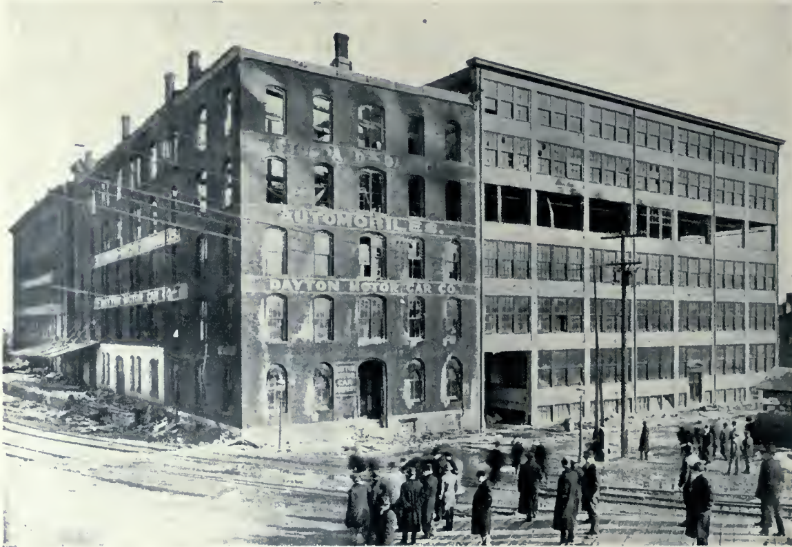
DAMAGED WAREHOUSE OF THE DAYTON MOTOR CAR COMPANY, DAYTON, OHIO, WHICH IS DEMONSTRATIVE OF THE FIRE-RESISTING PROPERTIES OF CONCRETE. THE FIRE STARTED ON THE FOURTH FLOOR OF THE CONCRETE STRUCTURE ON THE RIGHT, WHERE IT BURNED ITSELF OUT. THE ADJOINING BUILDING TO WHICH THE FIRE WAS COMMUNICATED WAS COMPLETELY GUTTED.
