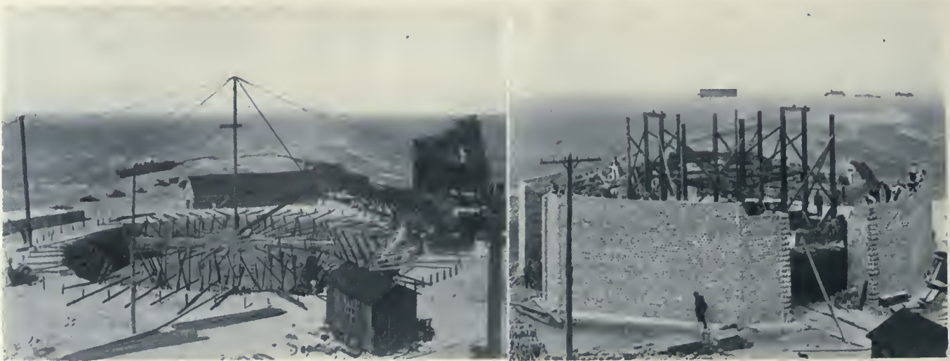
VIEWS SHOWING FALSE WORK OF FOUNDATION AND CONSTRUCTION OF OCTAGONAL BASE OF 506-FOOT CHIMNEY, RECENTLY ERECTED AT THE SMELTING WORKS OF THE BOSTON AND MONTANA CONSOLIDATED COPPER AND SILVER MINING COMPANY, GREAT FALLS, MONTANA.
