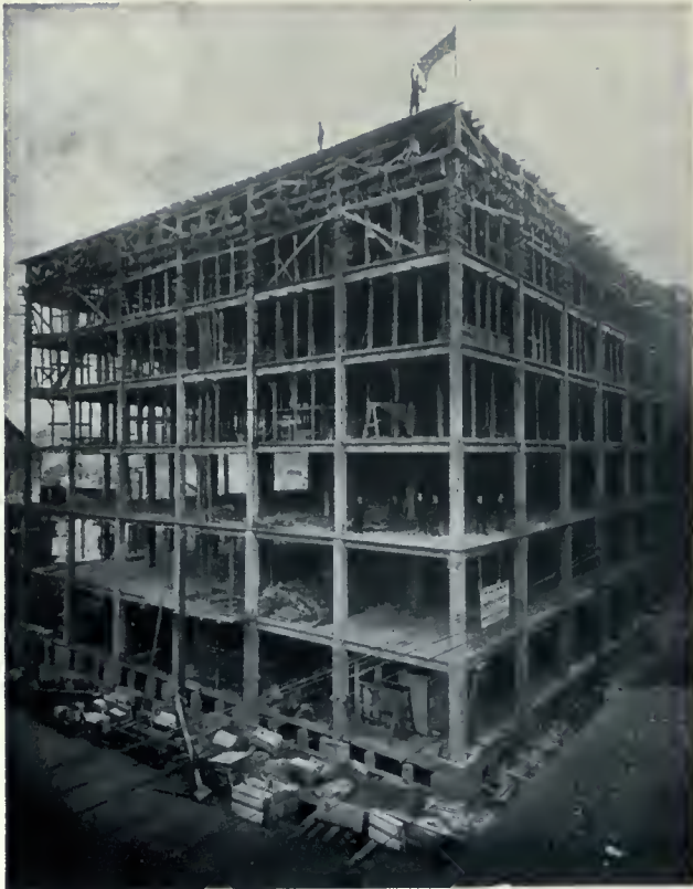
LYMAN SONS & COMPANY'S NEW BUILDING, MONTREAL. THIS BUILDING DEMONSTRATES THE POSSIBILITIES OF QUICK CONSTRUCTION IN REINFORCED CONCRETE, THE FRAME WORK, INCLUDING ALL FLOORS AND THE ROOF, WAS COMPLETE TWO AND A HALF MONTHS AFTER EXCAVATION. MITCHELL & CREIGHTON, ARCHITECTS.
