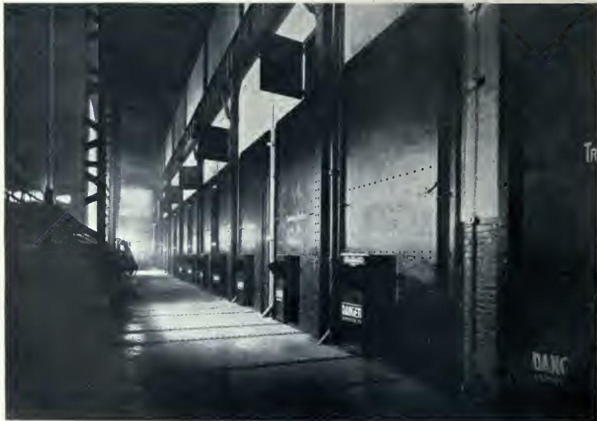
View showing Transformer Banks, power plant of Electrical Development Company, Niagara Falls, Ont. E. J. Lennox, Architect.
