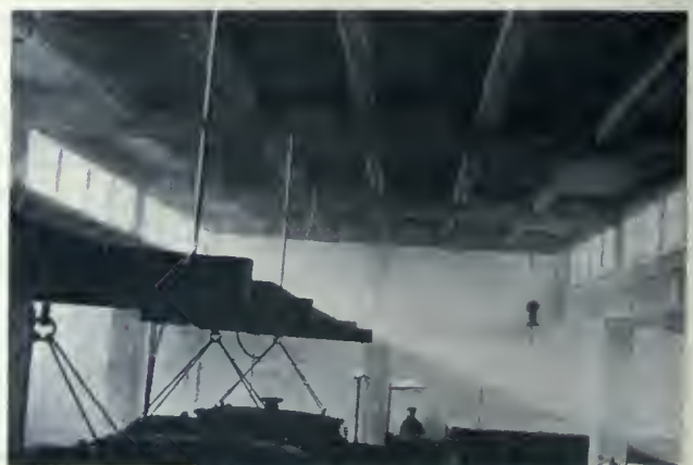
PLANT OF WOOD PRODUCTS COMPANY—THIS VIEW SHOWS THE WIDE SPAN ROOF CONSTRUCTION OF THE MAIN DISTILLERY ROOM OF THE STILL HOUSE. THE SPAN HERE SHOWN IS 32 FEET IN THE CLEAR FOR THE GIRDERS, WITH 18-FOOT LONGITUDINAL SPAN FOR THE BEAMS. E. D. PITT, DESIGNING AND CONSTRUCTING ENGINEER.
