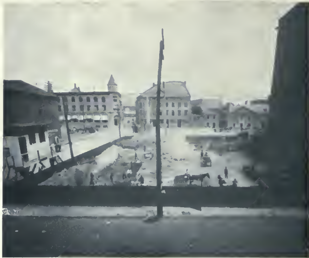
VIEW TAKEN JUNE 1ST, 1908, SHOWING EXCAVATION ALMOST COMPLETED FOR LYMAN SONS AND COMPANY'S NEW REINFORCED CONCRETE BUILDING, MONTREAL. MITCHELL AND CREIGHTON, ARCHITECTS.
