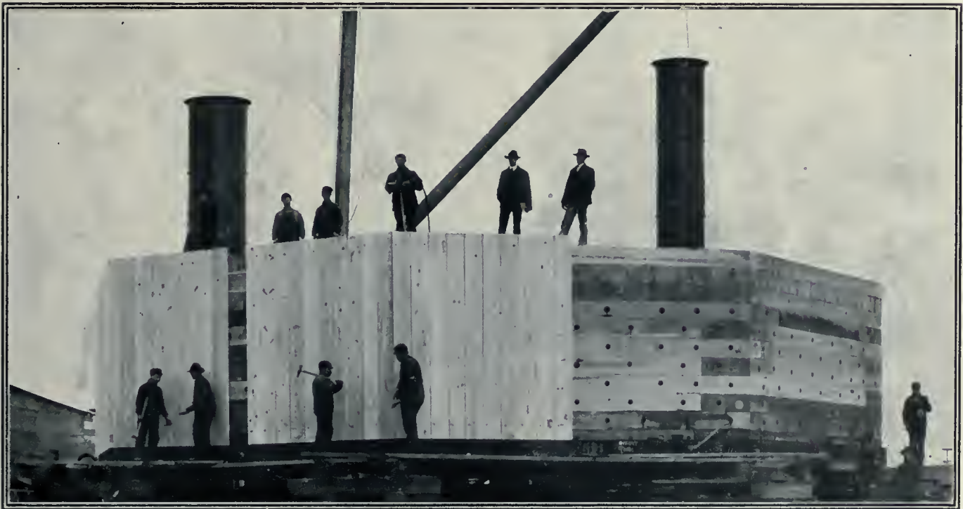
BUILDING CAISSON FOR PIVOT PIER, FORDHAM HEIGHTS, HARLEM RIVER BRIDGE, NEW YORK.
