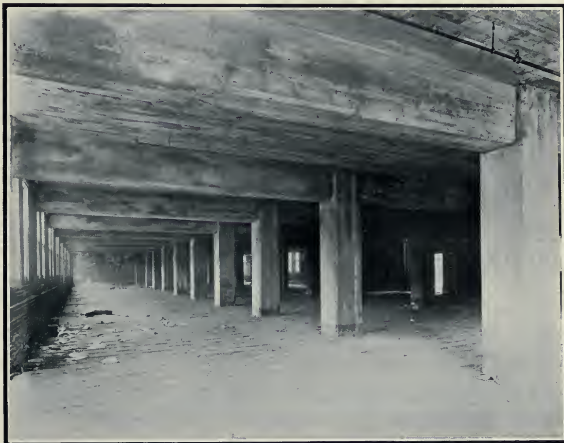
View of one of the floors, new Southam Building, Toronto, prior to applying the finishing coat or laying the hardwood super-floor. Messrs. Spratt & Rolph, Architects.
