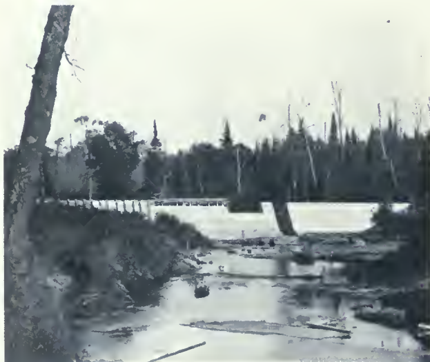
PLANT OF WOOD PRODUCTS COMPANY—VIEW OF DAM IN PROCESS OF CONSTRUCTION, SHOWING WASTE-WAY FOR THE NORMAL FALL OF THE BURNT RIVER, IN THE RECENT DRY SEASON. E. D. PITT, DESIGNING AND CONSTRUCTING ENGINEER.
