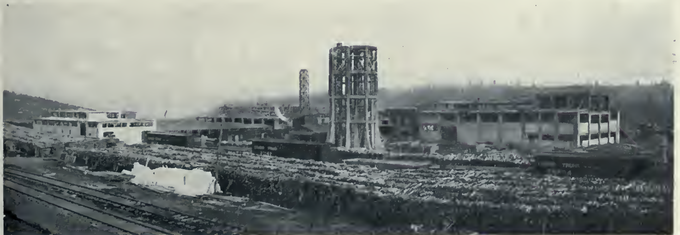
NEW PLANT OF WOOD PRODUCTS COMPANY—PANORAMIC VIEW TAKEN FROM THE WEST, SHOWING THE ENTIRE PLANT DURING PROCESS OF CONSTRUCTION. E. D. PITT, DESIGNING AND CONSTRUCTING ENGINEER.
