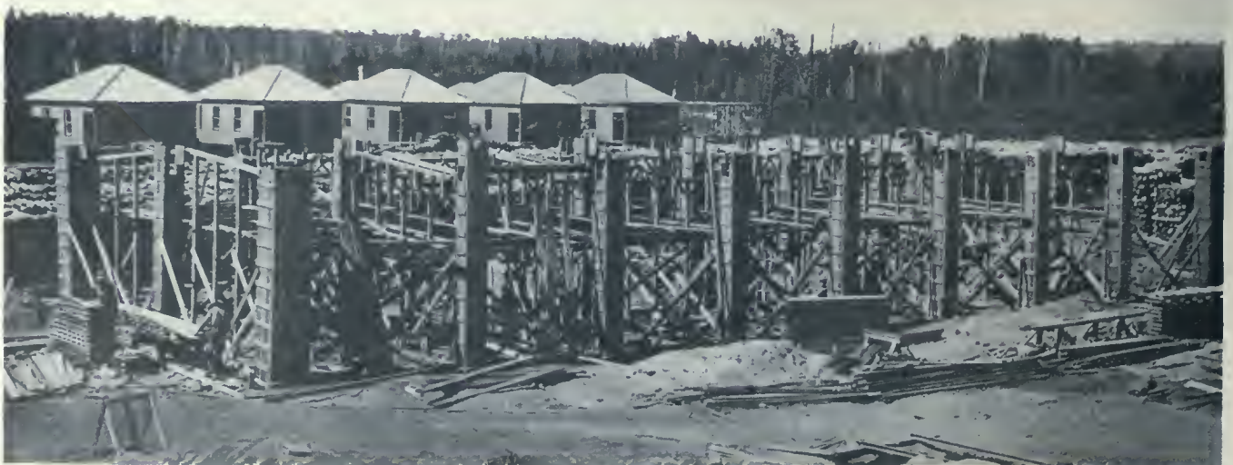
PLANT OF WOOD PRODUCTS COMPANY—FORM WORK PARTIALLY ERECTED AND COMPLETED FOR THE FIRST TOWER OF THE CHARCOAL HOUSE. THIS FORM WORK WAS PRACTICALLY ERECTED COMPLETE IN A DAY AND A HALF. E. D. PITT, DESIGNING AND CONSTRUCTING ENGINEER.
