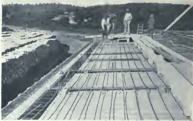
PLANT OF WOOD PRODUCTS COMPANY—ROOF OF CHARCOAL HOUSE, WITH REINFORCEMENT READY FOR THE POURING OF THE CONCRETE. ALL ROOFS ARE FIGURED FOR 125 LBS. LIVE AND DEAD LOAD. E. D. PITT, DESIGNING AND CONSTRUCTING ENGINEER.
