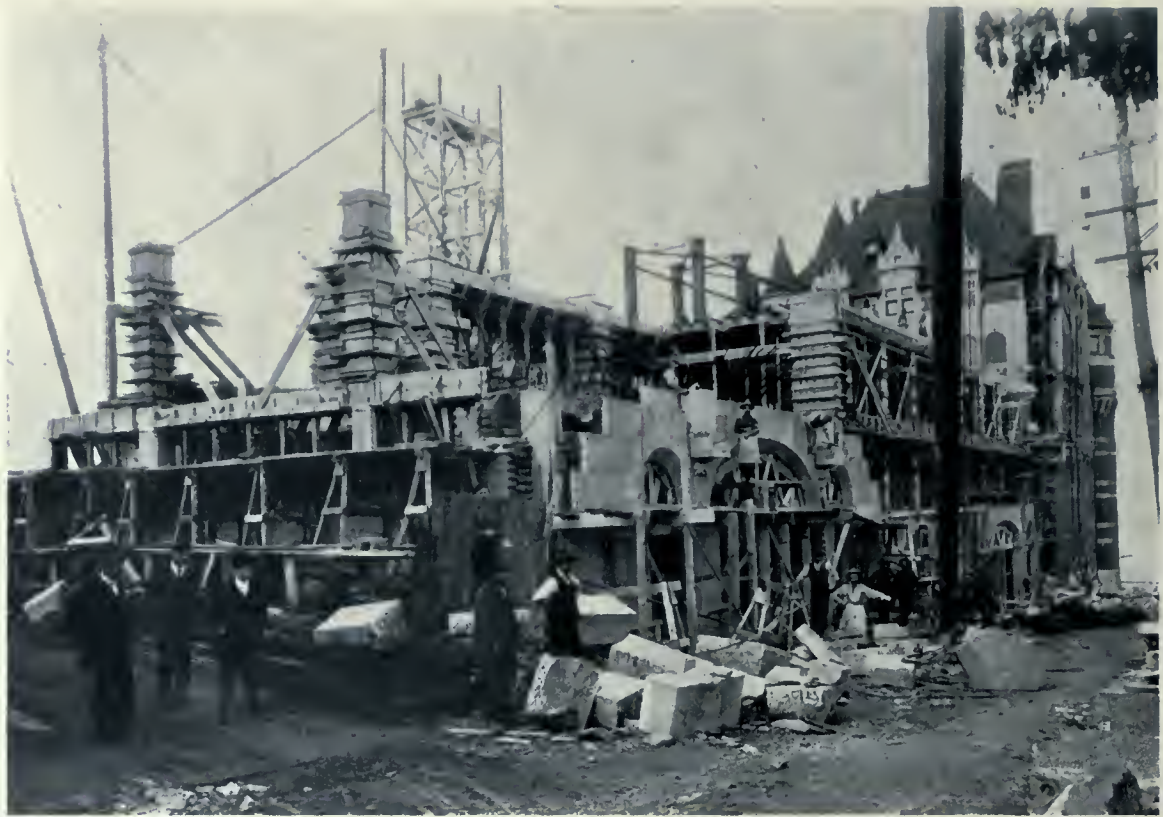
NEW ADDITION TO CHATEAU FRONTENAC, QUEBEC CITY. VIEW TAKEN AUGUST 20TH SHOWING THE MANNER IN WHICH THE CONCRETE SKELETON WAS WALLED IN WITH BRICK AND STONE, AND HOW SOON THIS WORK FOLLOWED THE CONSTRUCTION OF THE CONCRETE FRAME. W. S. PAINTER, ARCHITECT.
