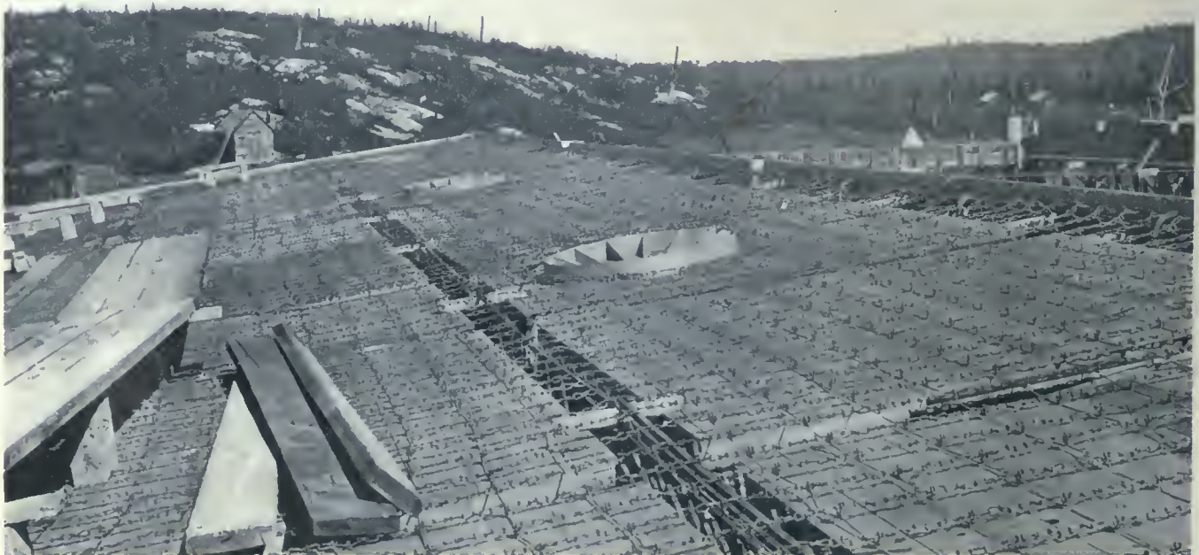
PLANT OF WOOD PRODUCTS COMPANY—ROOM OF OVEN HOUSE SHOWING CHAIN FABRIC REINFORCEMENT READY FOR THE POURING OF THE CONCRETE. NOTE THE OPENINGS FOR VENTILATING STACKS OVER OVEN. E. D. PITT, DESIGNING AND CONTRACTING ENGINEER.
