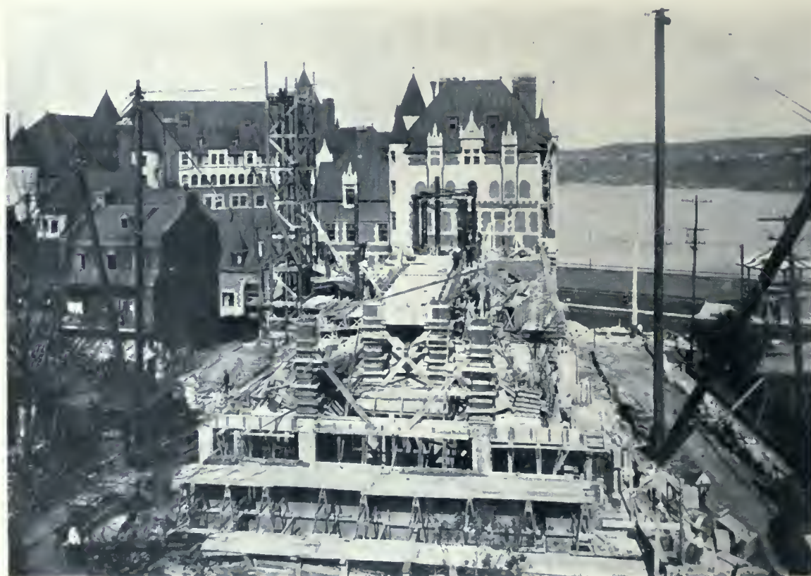
NEW ADDITION TO CHATEAU FRONTENAC, QUEBEC CITY. VIEW TAKEN AUG. 14TH, SHOWING THE GENERAL FLOOR CONSTRUCTION, TOGETHER WITH THE CONCRETE COLUMNS IN THE FOREGROUND WHICH ARE DESIGNED TO CARRY THE TOWER PORTION OF THE BUILDING. W. S. PAINTER, ARCHITECT.
