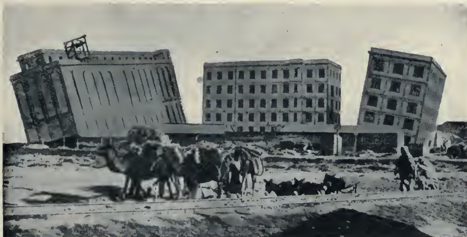
GRAIN WAREHOUSES IN TUNIS, AFRICA. A REMARKABLE PICTURE SHOWING TWO LARGE CONCRETE STRUCTURES THROWN 25 DEGREES OUT OF PLUMB, OWING TO ESCAPE OF QUICK SAND ON WHICH THEY WERE BUILT. BOTH WERE BROUGHT BACK TO A VERTICAL POSITION WITHOUT DEVELOPING A CRACK IN EITHER STRUCTURE. THIS WAS DONE BY LOADING SAND ON THEIR HIGH SIDE AND EXCAVATING UNDERNEATH.
