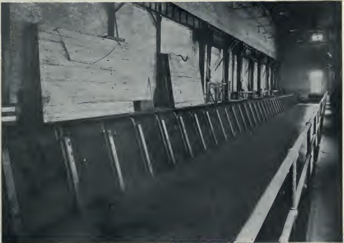
Screen Room, Generating Station, Electrical Development Company's Power Plant, Niagara Falls, Ont., showing the immense steel gratings through which the water passes to the turbines. E. J. Lennox, Architect.
