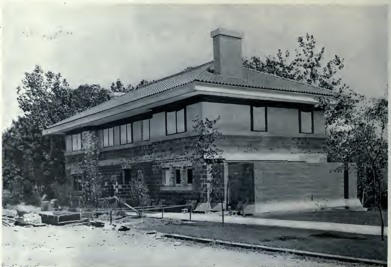
View of residence of Dr. George E. Harter, Elkhart, Ind., in process of construction, showing the concrete block walls before the cement stucco was applied.
