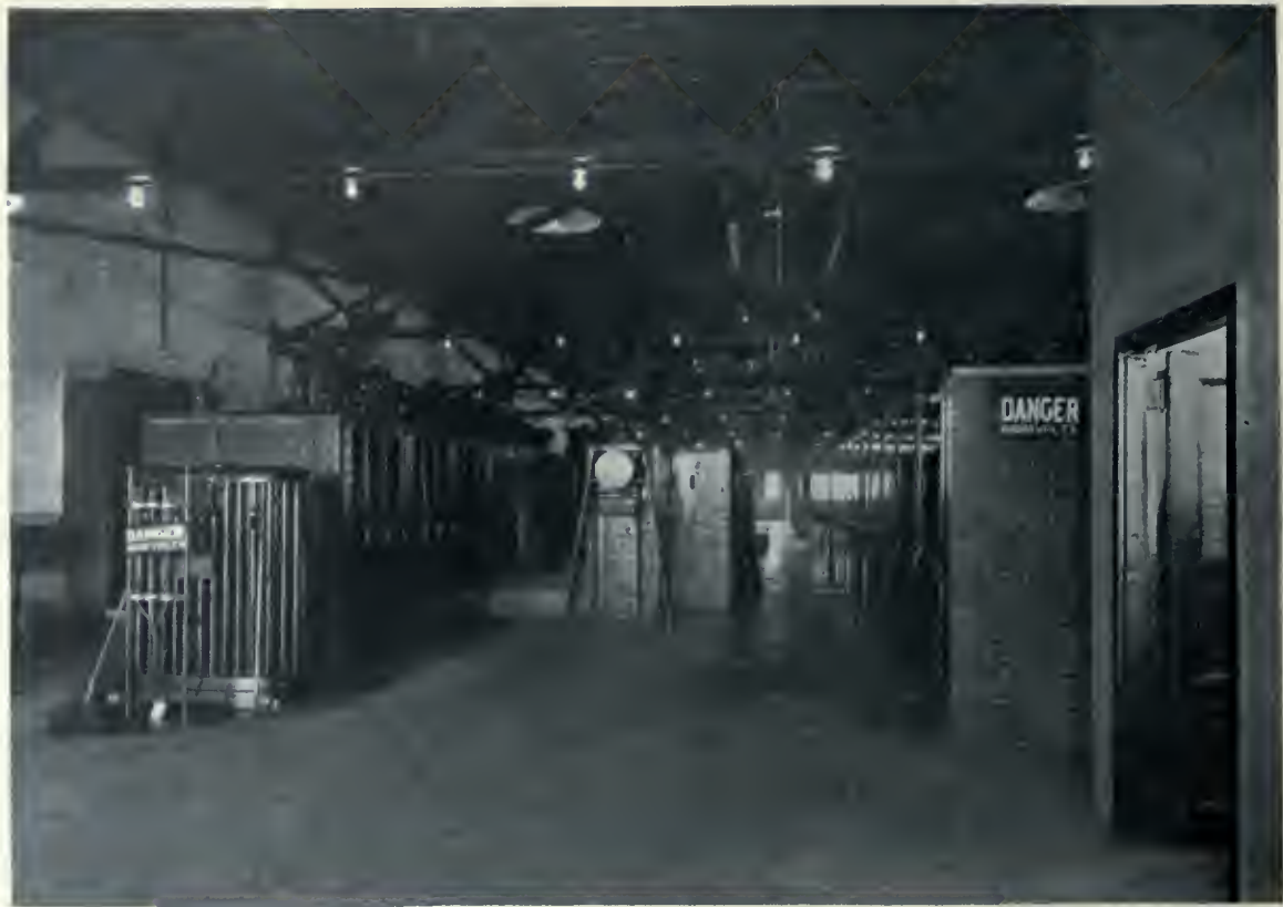
Interior of Transformer Station, power plant of the Electrical Development Company, Niagara Falls, Ont., showing the terra cotta ceiling with its structural steel supporting members. E. J. Lennox, Architect.
