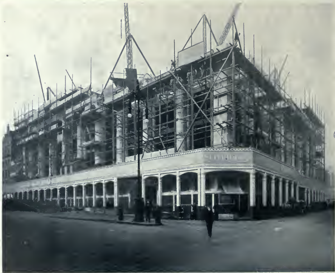
VIEWS OF SELFRIDGE & COMPANY'S BUILDING, SHOWING PROGRESS OF CONSTRUCTION ON SEPTEMBER 17 AND OCTOBER 2. AN IDEA AS TO THE RAPIDITY WITH WHICH THE WORK IS BEING CARRIED OUT CAN BE SEEN FROM WHAT HAS BEEN ACCOMPLISHED IN THE SPACE INTERVENING THESE DATES.
