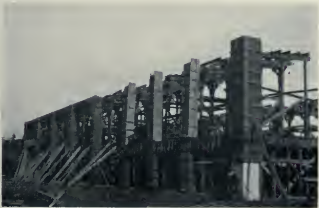
PLANT OF WOOD PRODUCTS COMPANY—FIRST STORY AND ROOF FORM WORK FOR THE STILL HOUSE. IT IS WORTHY OF NOTE THAT THE LUMBER FOR THE FORM WORK WAS USED ONLY ONCE. E. D. PITT, DESIGNING AND CONSTRUCTING ENGINEER.
