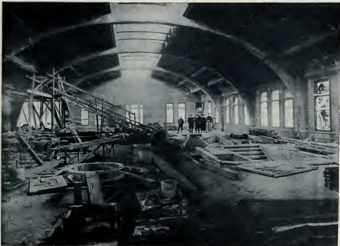
INTERIOR OF TELEPHONE BUILDING, SHANGHAI, CHINA, SHOWING ARCHED TRUSSES OF THE REINFORCED CONCRETE ROOF.
