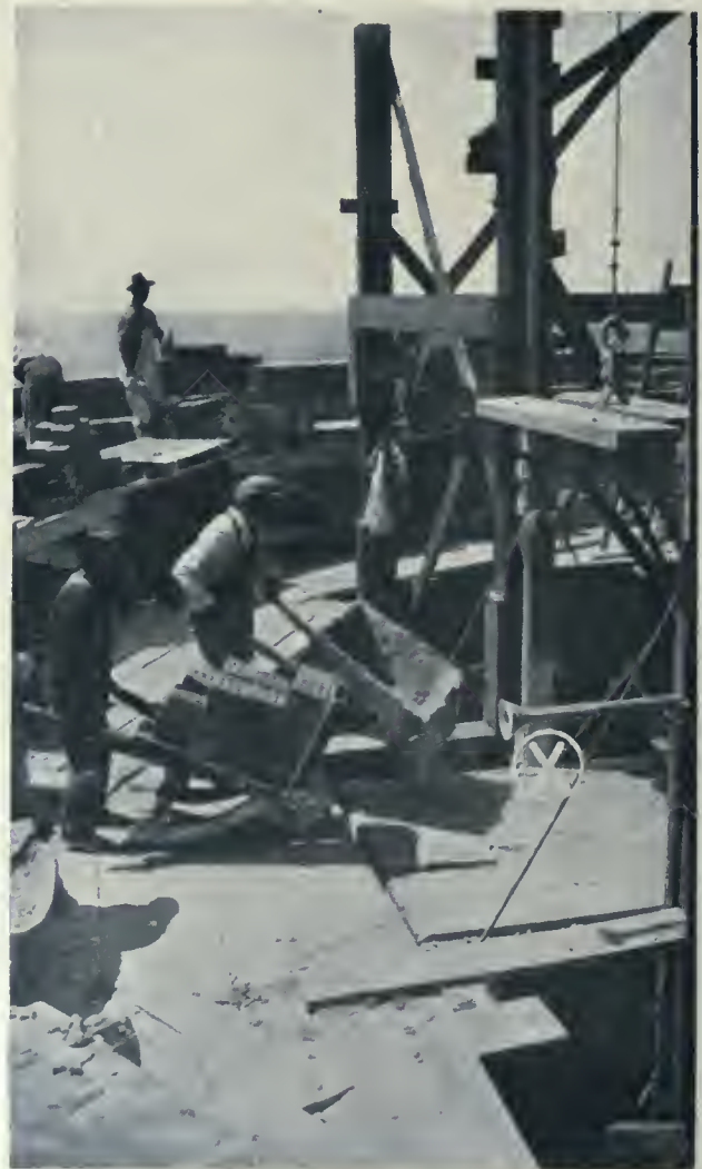
VIEW OF WORKMEN'S SCAFFOLD INSIDE OF STACK. THE SPEAKING TUBE SHOWN AT X IS PART OF A COMPLETE SYSTEM OF COMMUNICATION WHICH CONNECTED WITH EACH ELEVATOR.
