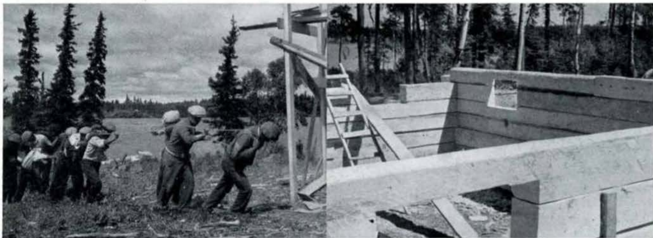
Hauling logs from the shore for the basement of the house. Huge trees were cut this spring within five miles of the post and floated to the site.
