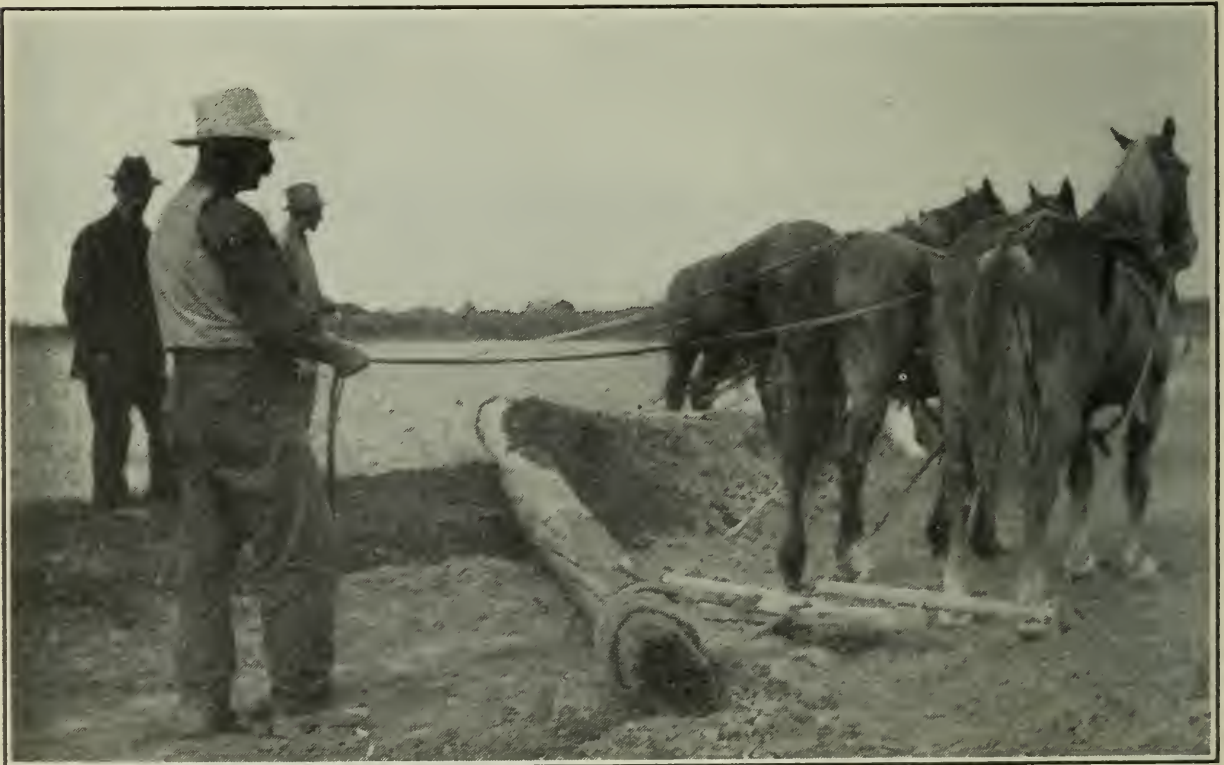
Fig. 10.—Using a log for backfilling. A stick of square timber is better. When drawn on an angle, the trench can be easily filled.
