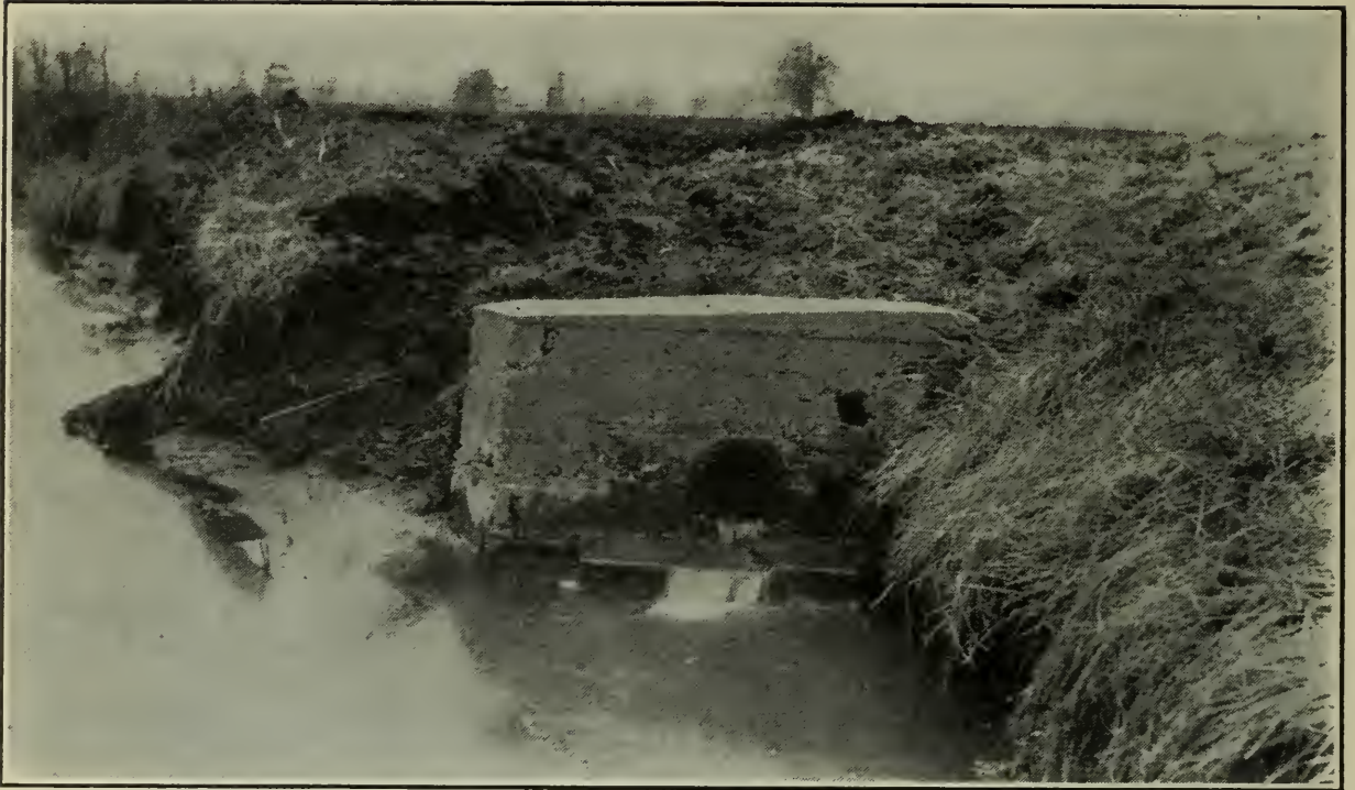
Fig. 14.—A well protected outlet—the concrete wall prevents caving, the screen the entrance of animals and the cement floor undermining of the wall.
