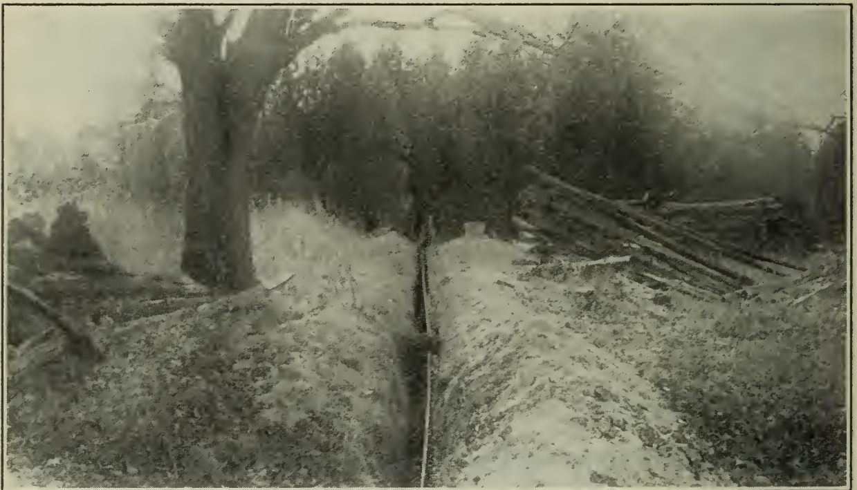
Fig. 27.—A Farm Spring being piped to the Farm Buildings. The actual Spring is shown in Fig. 9.
