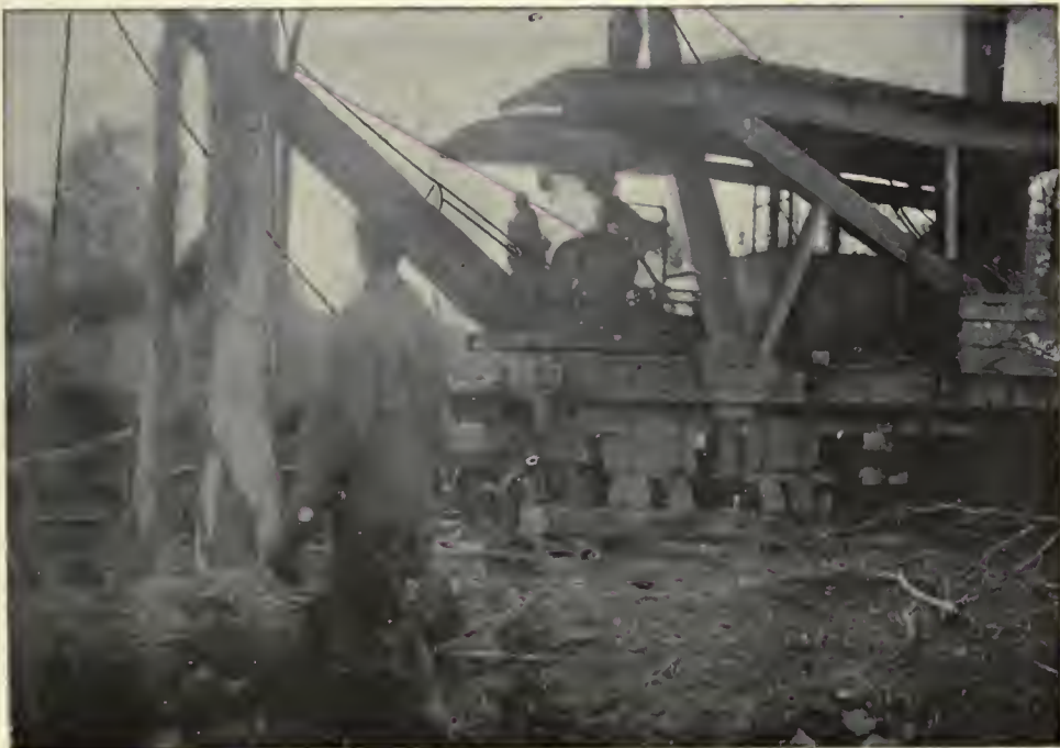
(2). Same as above, showing near view of wood blocks supporting the platform ;—Sardis, Mississippi.
