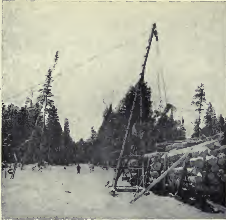
(1). PORTABLE GIN POLE ON SNOW SLED Sleigh on right being loaded from pile of logs (not shown) ; rope being pulled by horse.—River Marnie, Quebec.
