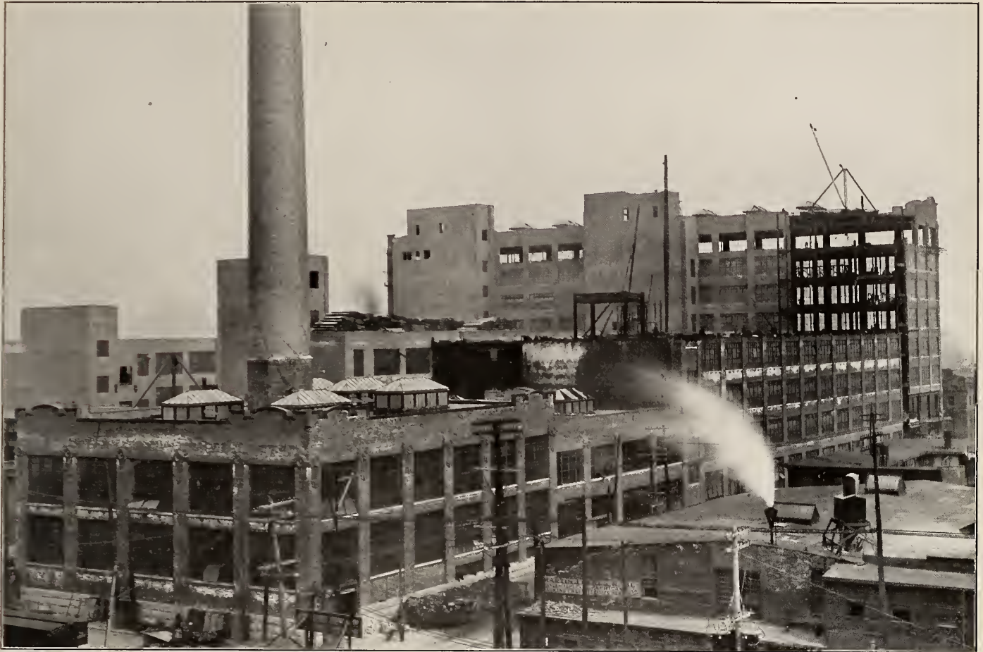
New Factory of the Northern Electric Company, Limited, Montreal, now under construction
