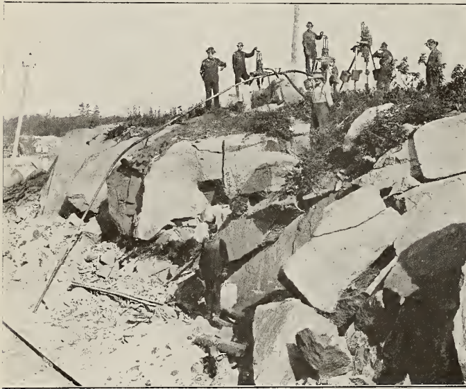
Drilling and Blasting the Last Section of Rock in the Rainy River Causeway
