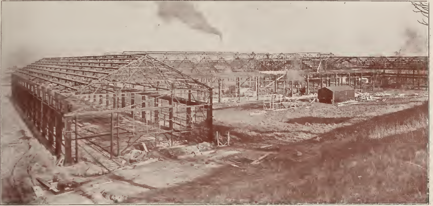
The Steel Work of the New Plant of the Canadian Rolling Mills, Montreal
