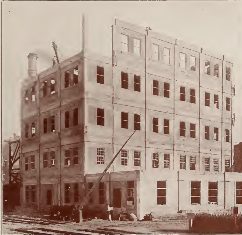
Example of Unit Construction. The above is one of Five Factory Units. (Courtesy of Factory).
