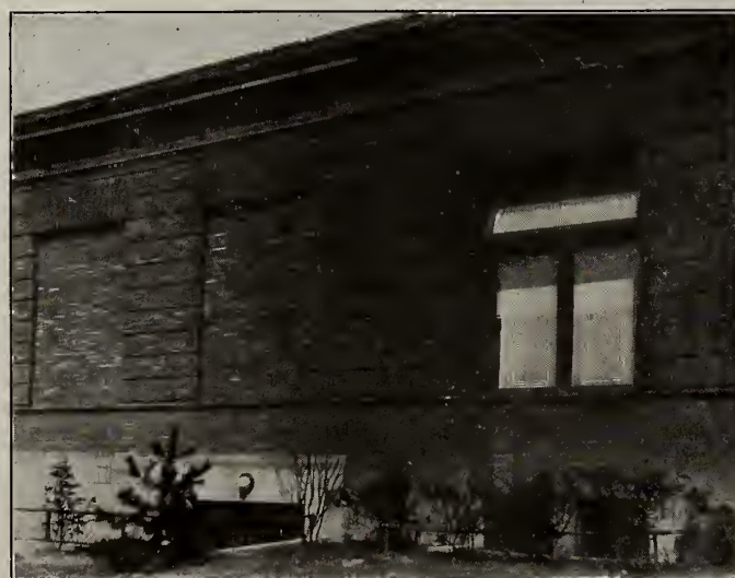
How Smoke Disfigures a Building
