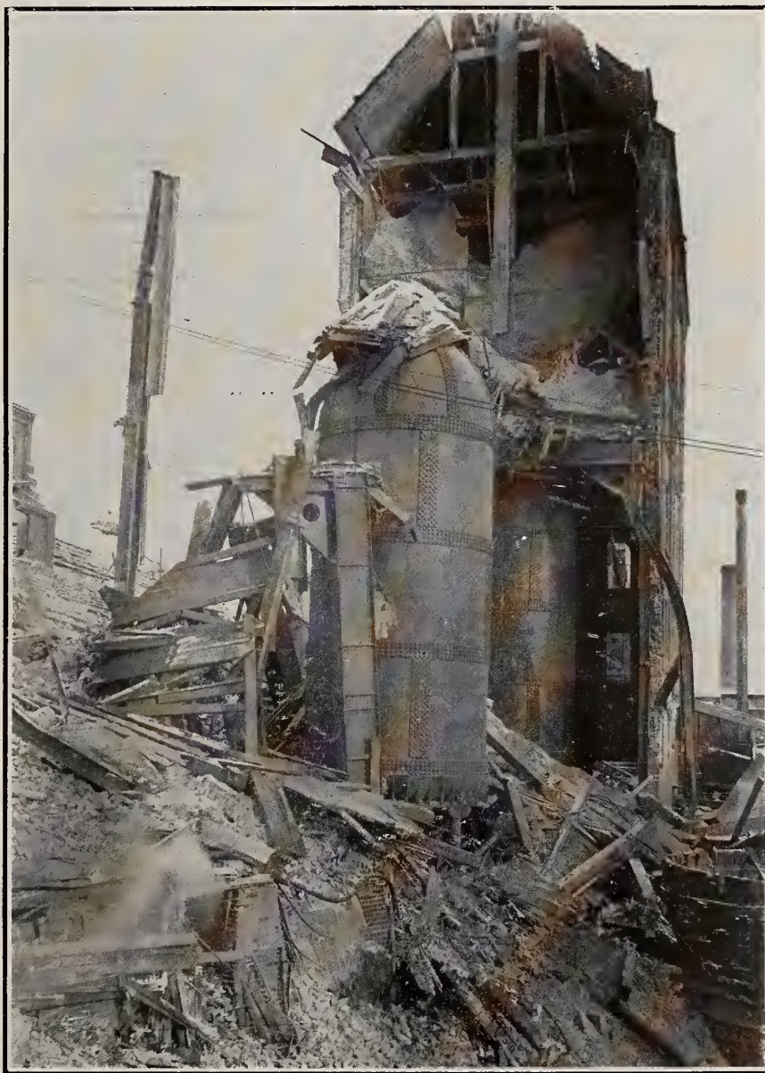
The Wrecked Digester House
