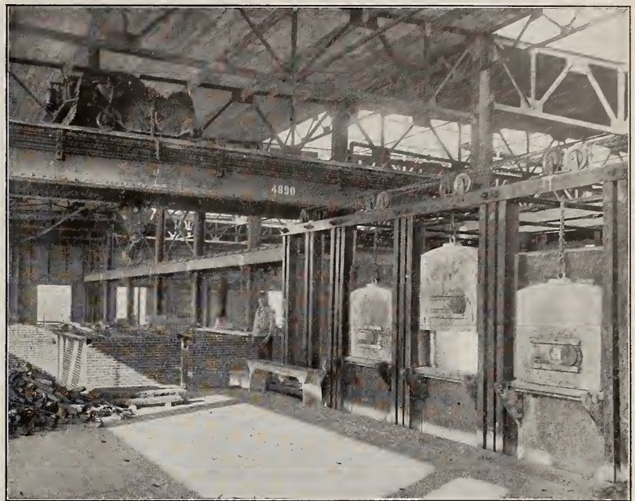
Interior of Dominion Steel Castings Company's Plant under Construction in Hamilton, Ont.
