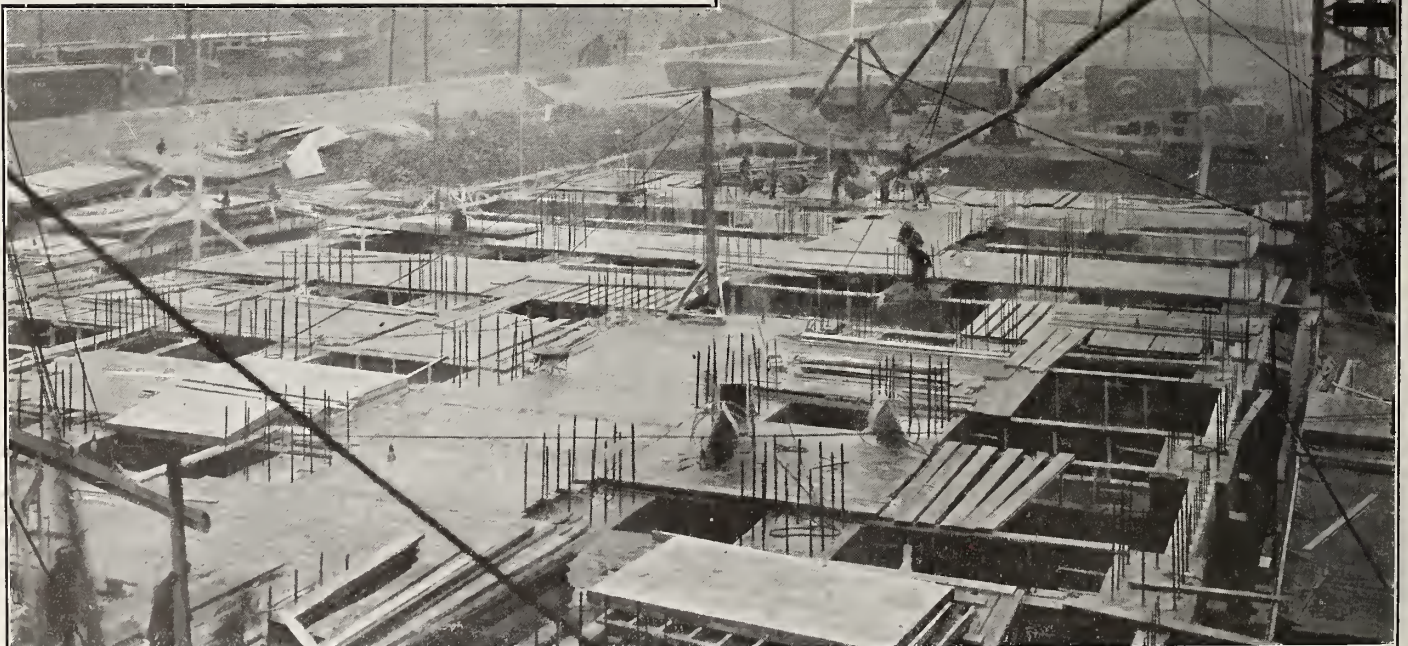
Elevator No. 2 of Harbor Commissioners of Montreal. Foundations Nearing Completion up to Wharf Level. Elevator When Completed Will Have Capacity of 2,000,000 Bushels.
