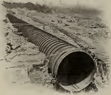
Section of Steel Penstock 18 ft. diam. and over 6000 ft. long built by us for the Ontario Power Company, Niagara Falls.
