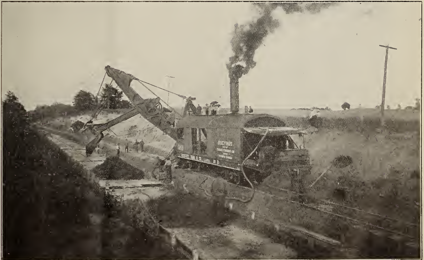
A construction gang at work on the Canadian Northern Railway. The steam shovel built by the Canada Foundry Co., is depositing earth on flat cars for distribution elsewhere.
