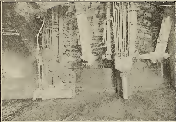
Blast Furnace Bosh
