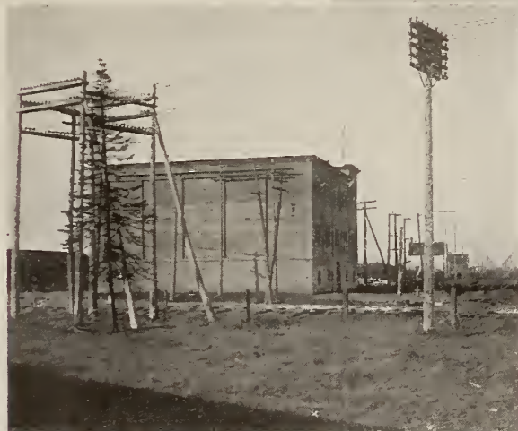
FORT WILLIAM sub-station showing transmission lines in duplicate from power house and distributing lines through the city.
