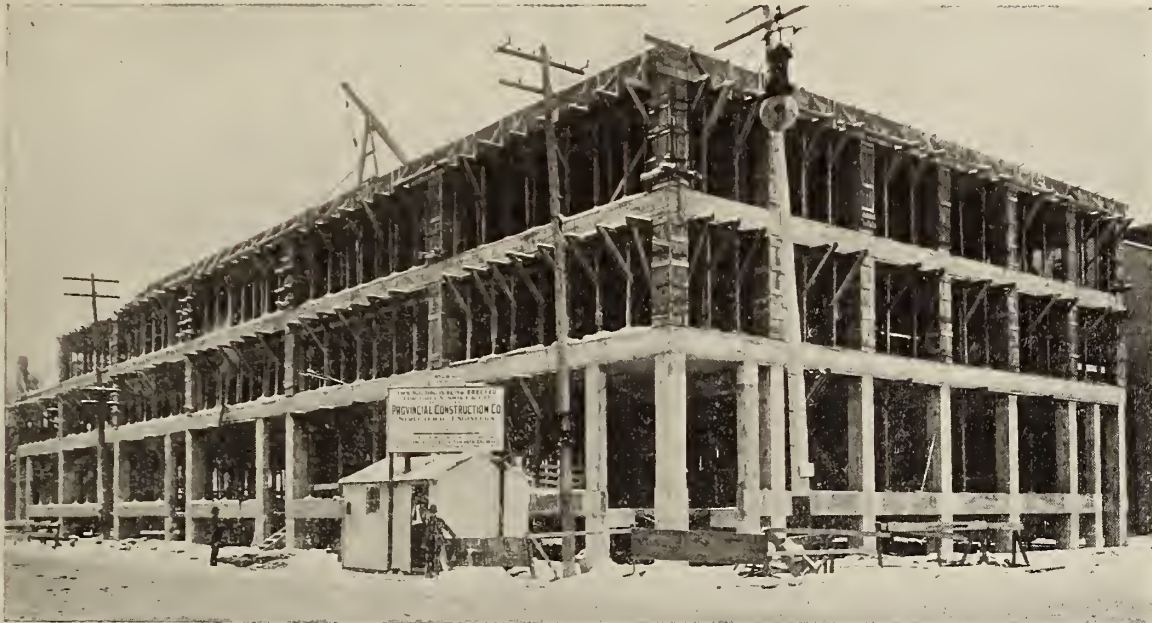
Factory Under Construction, with Re-inforced Concrete, Showing the Immense Possibilities for Lighting Under this System.
