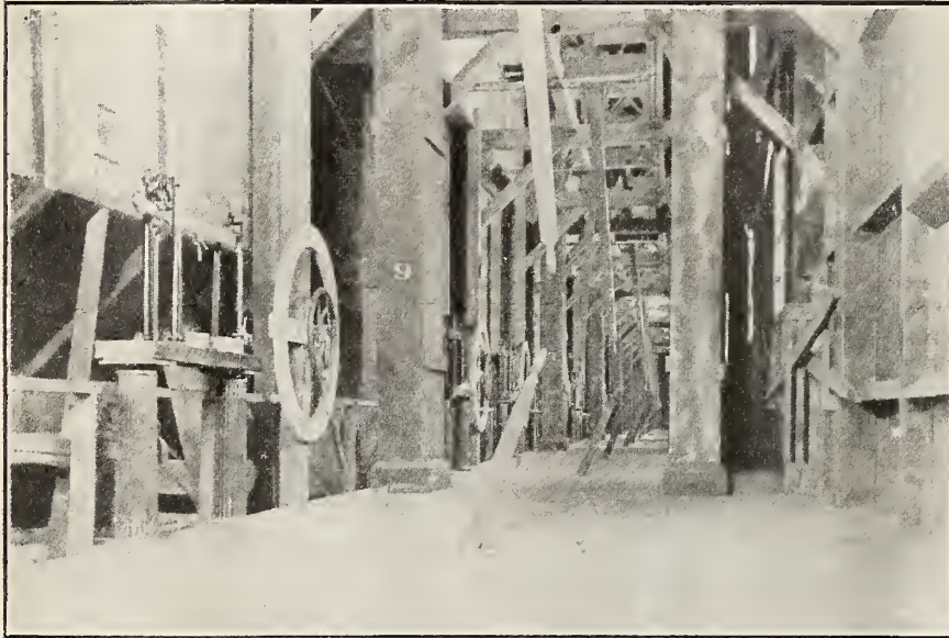
"Scale" Floor in Elevator A, showing ten 40 ton Scales, with dials for Setting Spouts.
