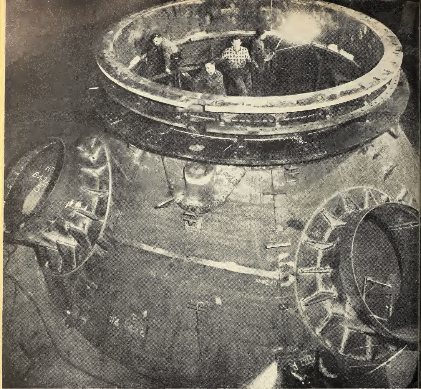
Fitting a ring casting to top cone section of blast furnace. Furnace shell is 76 ft. high ranging in diameter from 32 ft. at the bottom to 14 ft. 9 ins. at the top. It was made in Montreal.
