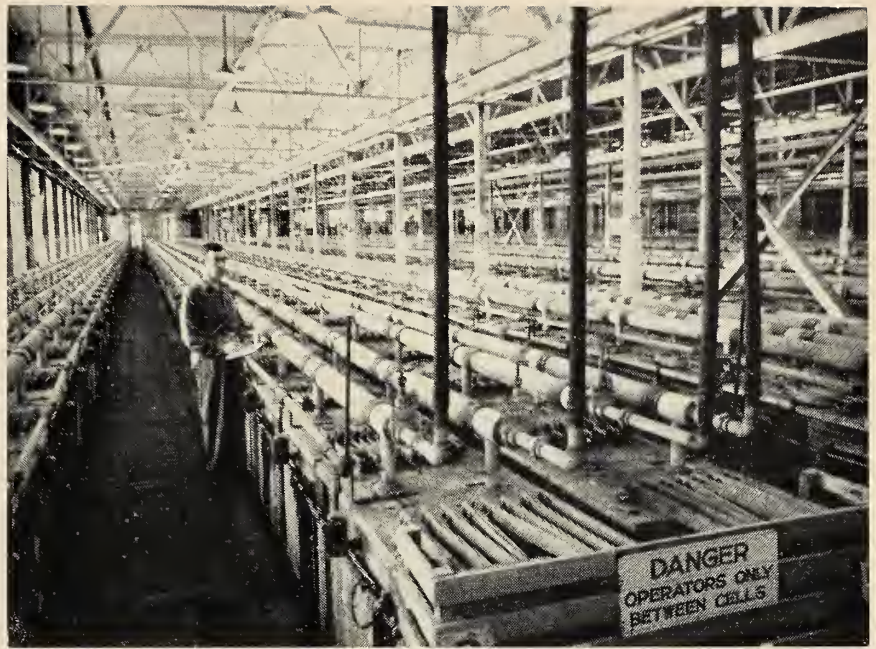
Fig. 2. Electrolytic Gas Cell Room. Shows typical arrangement of cells with oxygen and hydrogen row mains leading gases to coolers at the far end of the batteries. Hose connections in foreground are nitrogen supply lines for purging purposes.
