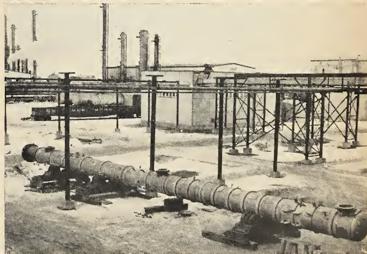
This 80-ft. long 36-inch diameter, stainless steel tower was fabricated in Edmonton for an Alberta petrochemical plant. Weight of the vessel is 22,000 pounds.
