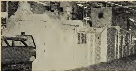
Interior 120 foot spray booth
