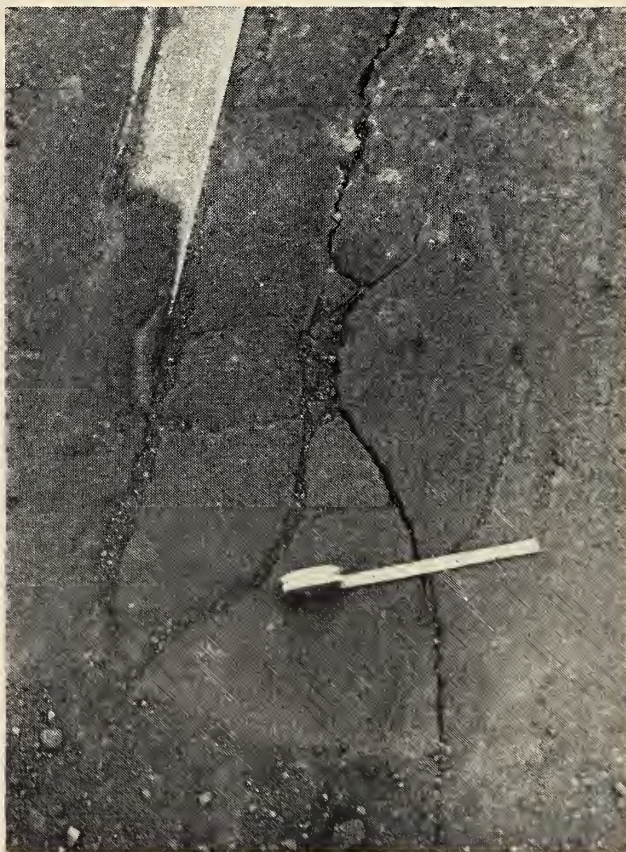
Fig. 6. Crack behind Richmond St. Bridge Abutment after 30 deg. temperature drop.
