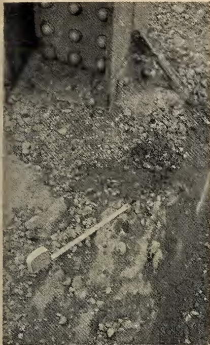
Fig. 9. (a) Crumbling Curb Concrete
