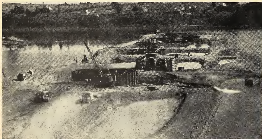
Fig. 10. Construction of Substructure, July 1958. From foreground to rear, cofferdams of piers 1, 2 and 3. The piles protruding from the cofferdam of pier 2 were later incorporated in the shaft of this pier.
