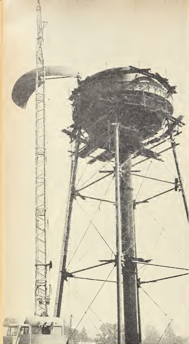
Dominion Bridge construction crews at our Vancouver branch hoist last segment of 100,000-gallon water tank. The tower is 102 ft. high and 28 ft. 8 ins. in diameter.
