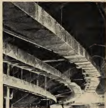
Galvanized Duct Work
