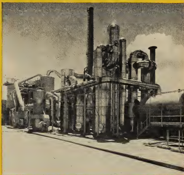
Sulphuric acid plant to produce 100 tons a day of acid from refinery waste gases at Shell Oil refinery, Geelong, Australia.
