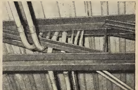
SMALL PIPES FOR OXYGEN, vacuum and electrical services are easily passed through the spaced double angle top chords of the joists directly into partitions without troublesome bends or offsets.
