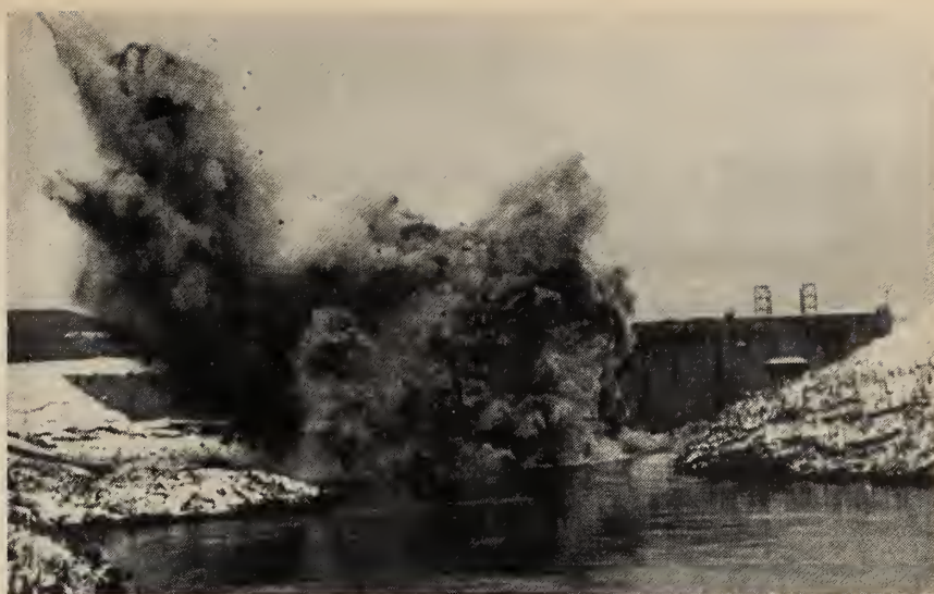
Fig. 9. The blast on 19th April, 1959, removed the rock plug, and water filled the intake tunnel. 60,000 pounds of explosive removed 13,000 cu. yd. of rock (rapid sequence film).
