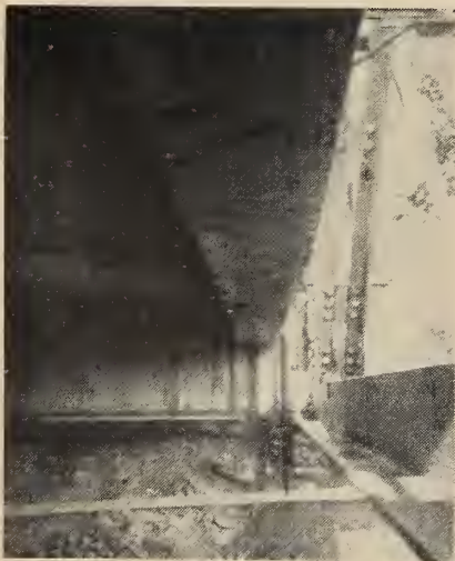
Fig. 12. Edge stringer failure and suggested methods for strengthening the edge panel
