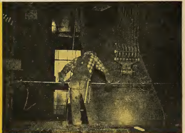
THE DRUM MOVES IN. Here is one of the two B&W steam drums being moved into position for installation. Each B&W Boiler can supply 625,000 lbs. of superheated steam per hour.
