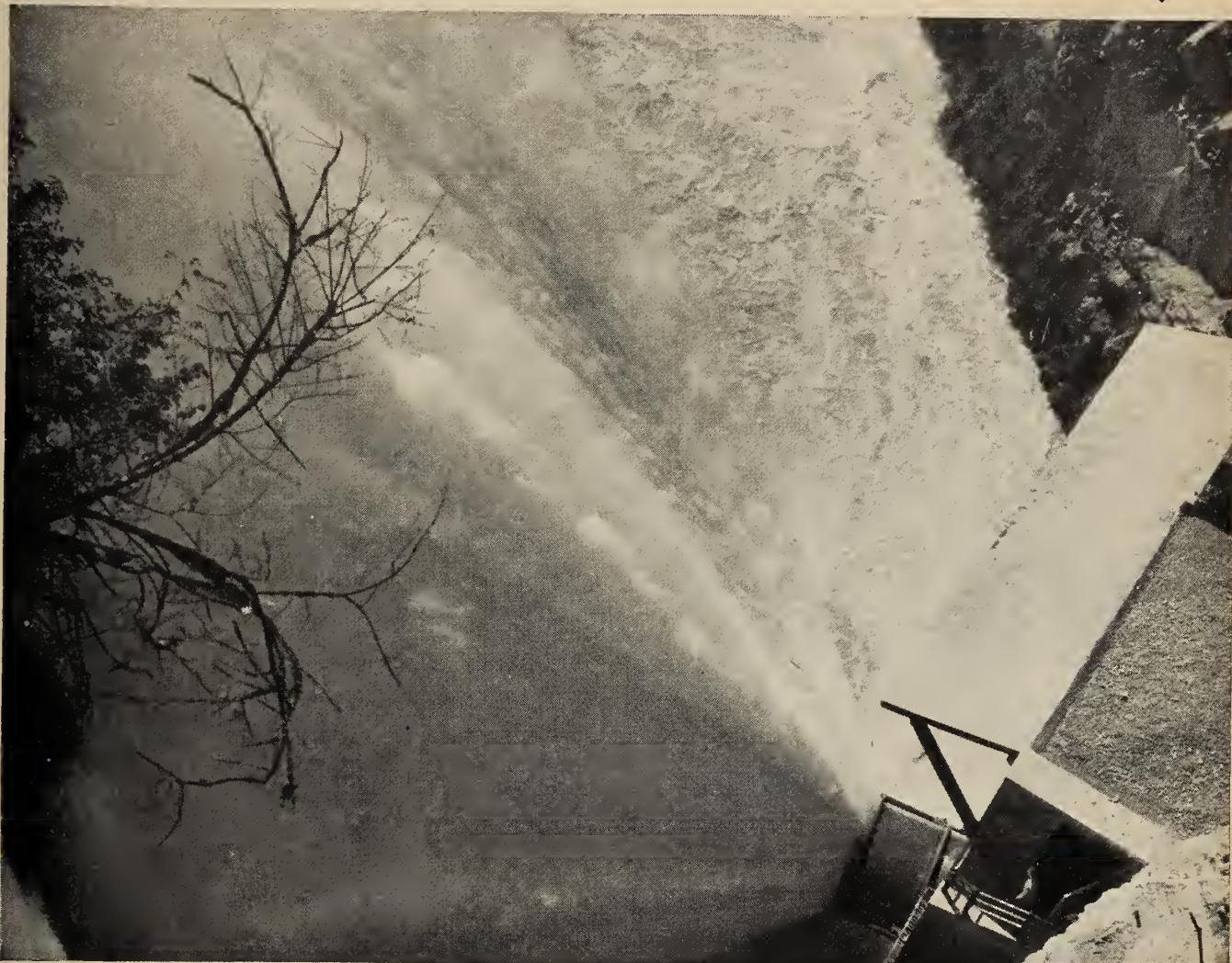
One of three 96-inch Howell-Bunger valves in operation at the U. S. Engineers Mud Mountain Dam, White River, Wash.
