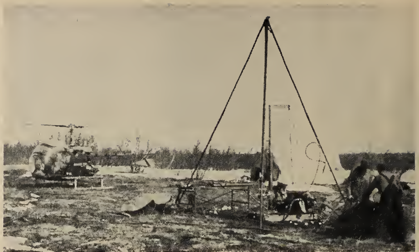
Fig. 5. Drill rig operation before airlift to next drilling location. Tent in background provides shelter for soil sampling and photographing frozen cones.
