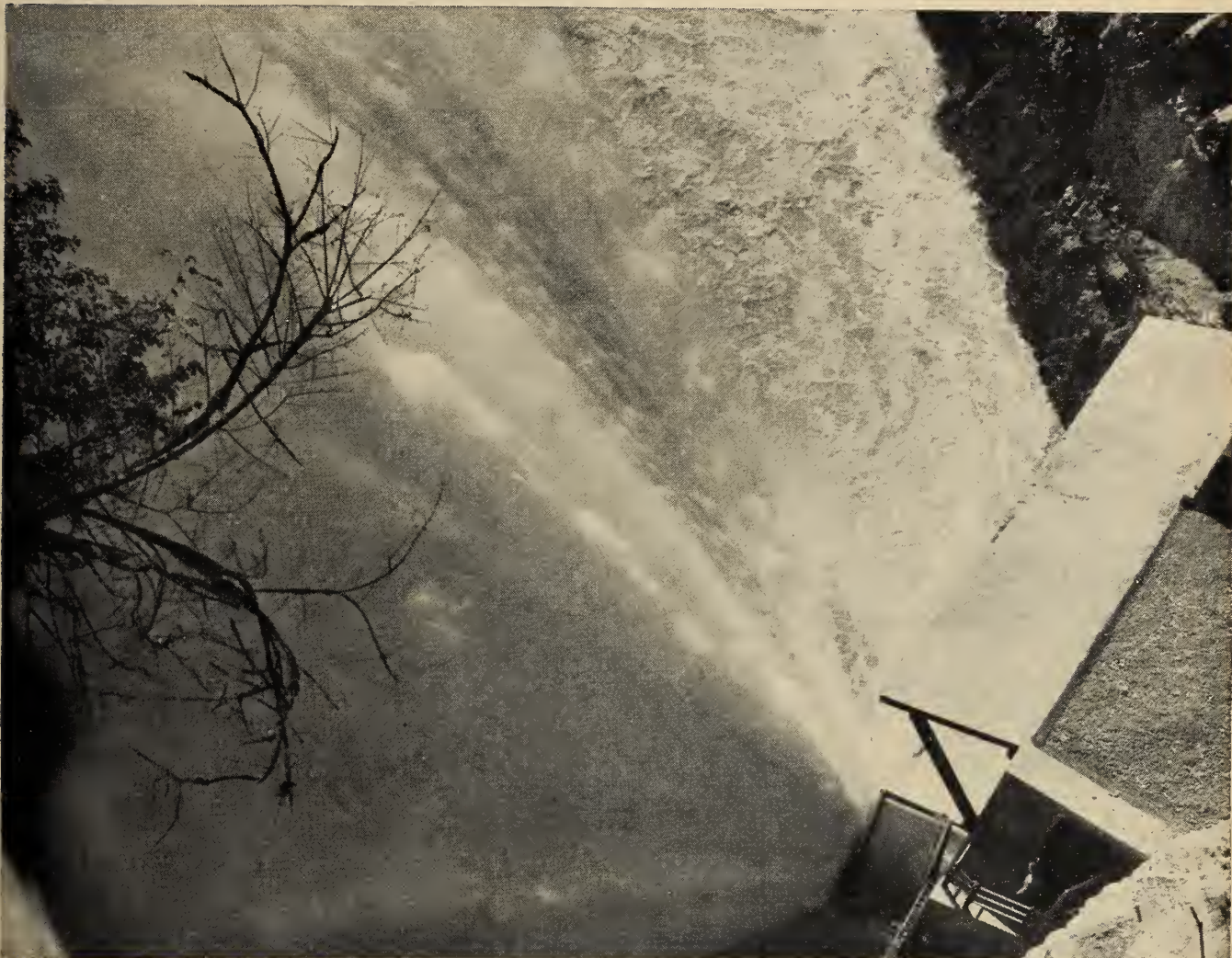
One of three 96-inch Howell-Bunger valves in operation at the U. S. Engineers Mud Mountain Dam, White River, Wash.
