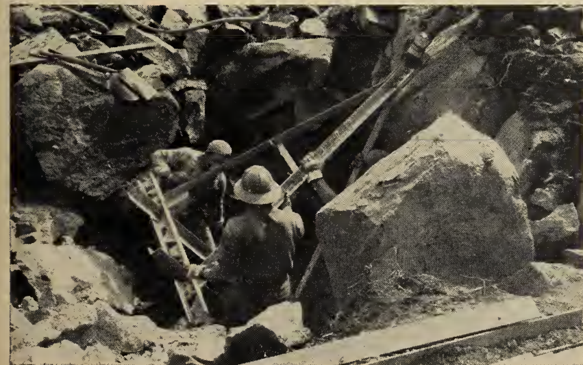
Fig. 6. Quadruped grillage being set. Bearing angles are placed in the triangular slots in channels. Broken rock is typical of conditions encountered at tower sites.
