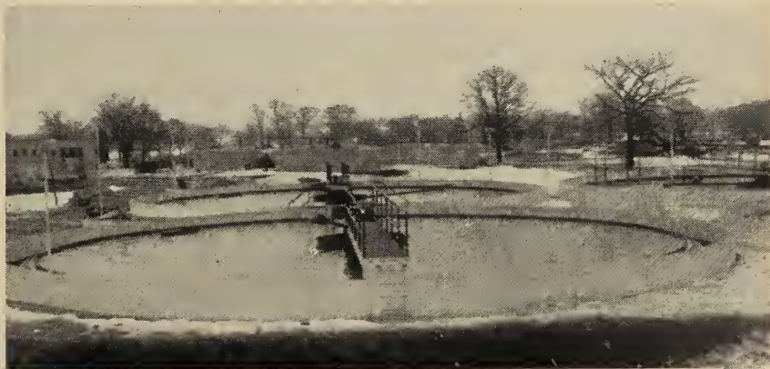
Fig. 1 Primary clarifiers at Brantford's new sewage treatment plant. Sludge digesters are in the background.
