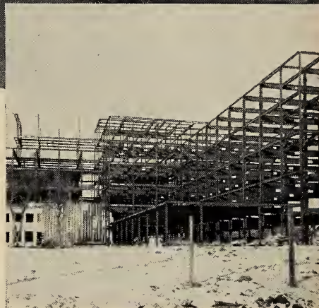
1800 tons of steelwork, fabricated and erected by Dominion Bridge, Winnipeg. Most of this was of "rigid frame" design.
