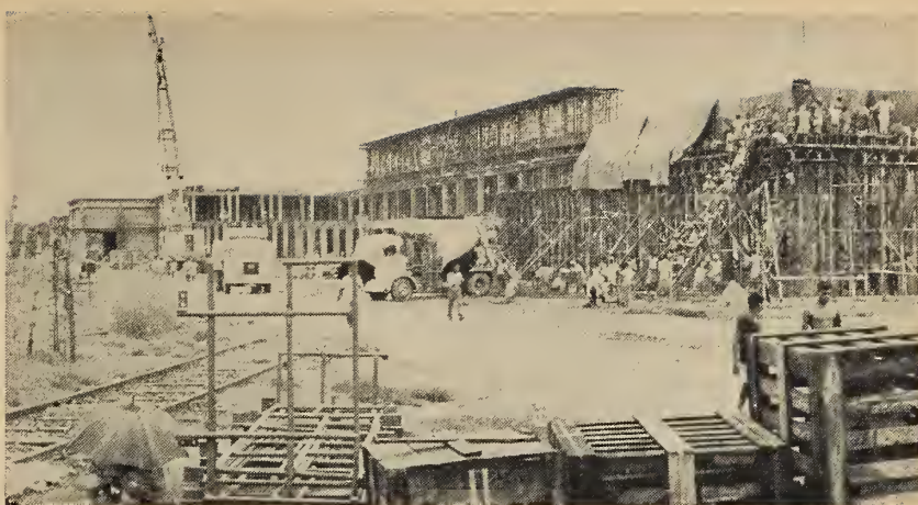
Fig. 2. General view of mill during construction. Note that concrete was delivered by mobile mixer but placed by "human bucket elevator".
