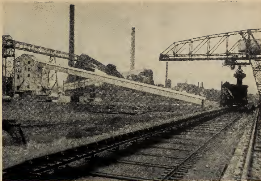
Fig. 3. View of new coal handling system just after completion. The travelling hopper is being loaded at the extreme right. Blending bins at right centre. Storage bin above coke ovens at left centre. Construction of new conveyor system to new oven bin at upper left.
