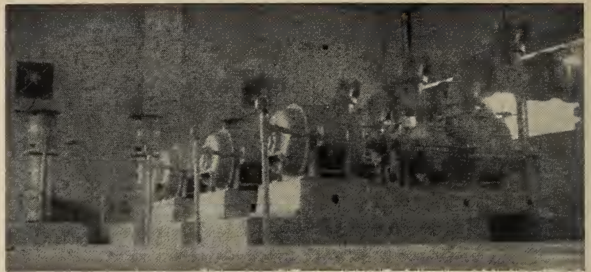
Fig. 2 Air Compressors in the main pumphouse in Stratford's OWRC-built and operated sewage treatment plant which was opened in 1958.
