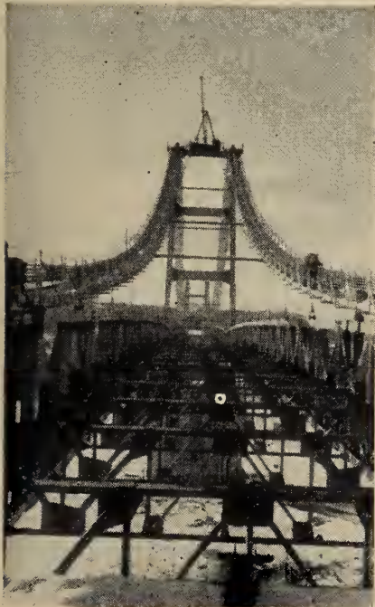
Fig. 7. Floor Trusses together with the stiffening trusses and cables, looking south through the middle of the bridge
