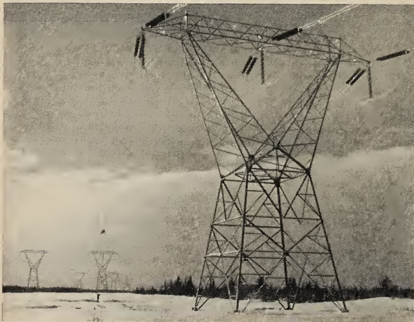
Fig. 2. Deadend assemblies on 20° strain tower. Note mid-span installation of spacers.
