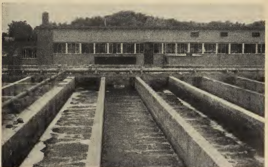
Fig. 1. Aeration tanks at the new activated sludge plant at Stratford designed to protect the Avon River.
