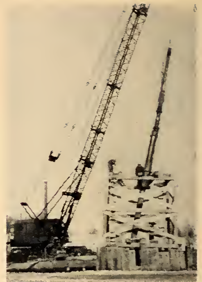
Fig. 2. Driving pipe piles with a diesel pile hammer. Pipe pile positioning and driving frame was 16 ft. square by 16 ft. high and secured to top of sheet pile cofferdam by chains tightened with loggers' load binders.
