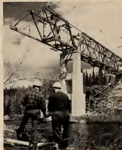
The Crow River Valley Bridge, one of the major building projects on the second half of C.N.R.'s new $35 million Chibougamau branch line.
