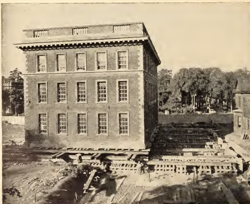
Fig. 3. Here, the building has come to rest over its new foundation after moving 250 ft. from the old site.
