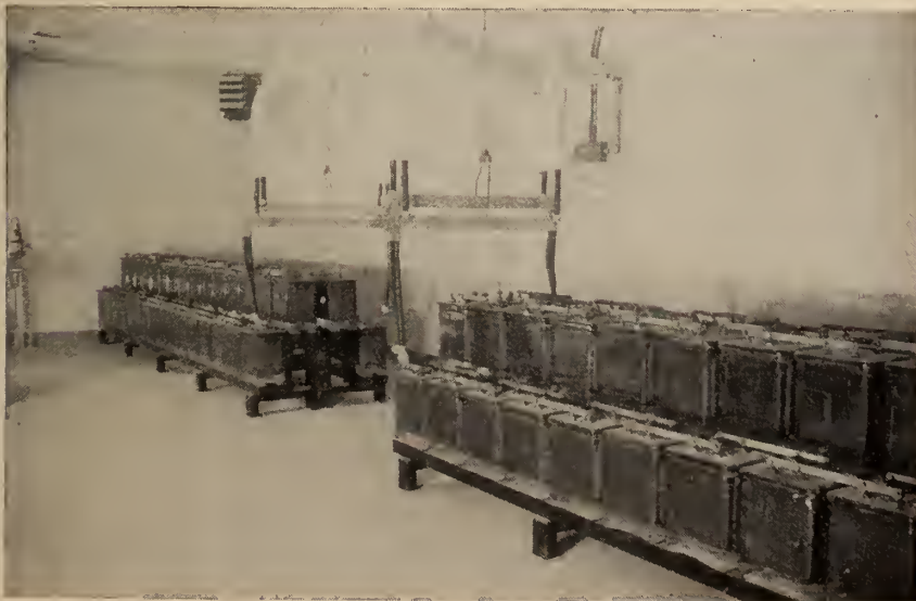
Fig. 5 — The accumulator room.
