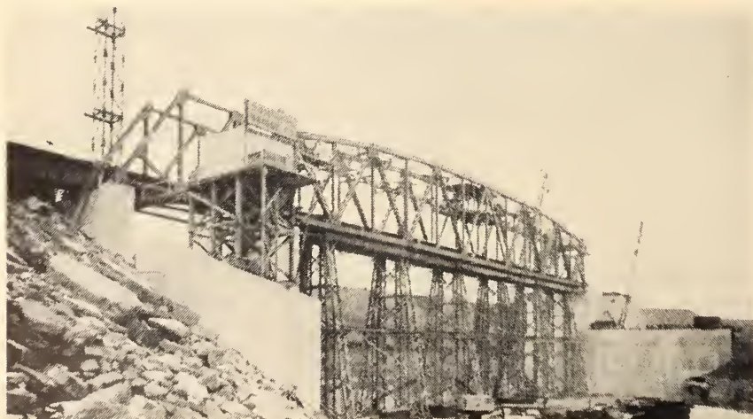
Fig. 13. Falsework upon which both the Caughnawaga spans were constructed, one after the other.
