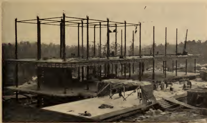
Fig. 3. The lift slab method is an ideal winter construction method because the concrete slabs can be placed with a single enclosure at ground level (Carleton University Arts Building, Ottawa).
