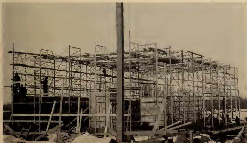
Erection of structural steel for engine test house at T.C.A.'s new turbine maintenance and overhaul base at Montreal's Dorval Airport.
