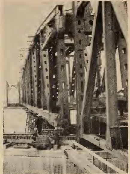
Fig. 14. Translation of span at Caughnawaga on twenty wheel trucks running on rails.
