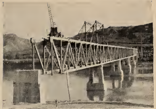
The recently-opened P.G.E. Railway bridge across the Peace River in B.C. — shown here under construction.
