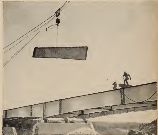
Construction view of plate girder bridge over the Exploits River in Newfoundland.
