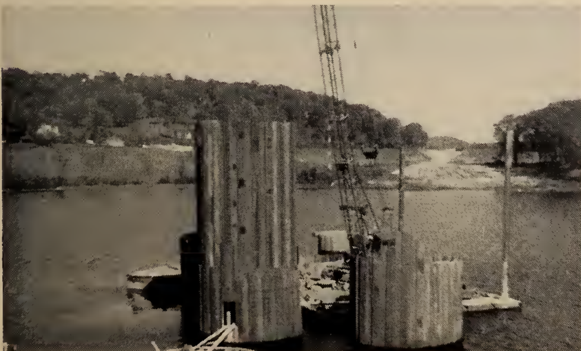
Fig. 1. Set-up for testing pipe pile. Sheet pile cell was placed on top of cofferdam undergoing test and filled with 450 tons of sand and gravel. Jack inside the test cell transmitted load to piling.
