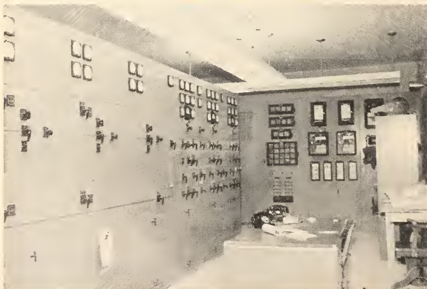
Fig. 11. Whitedog Falls control room.
