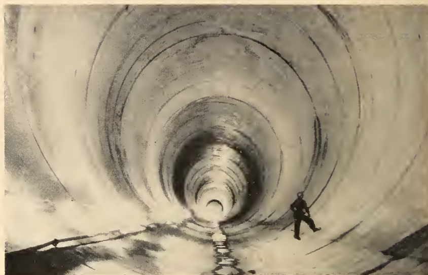
Fig. 3. Interior view of 45 ft. diameter Niagara tunnel No. 2 near downstream end with concrete lining complete.
