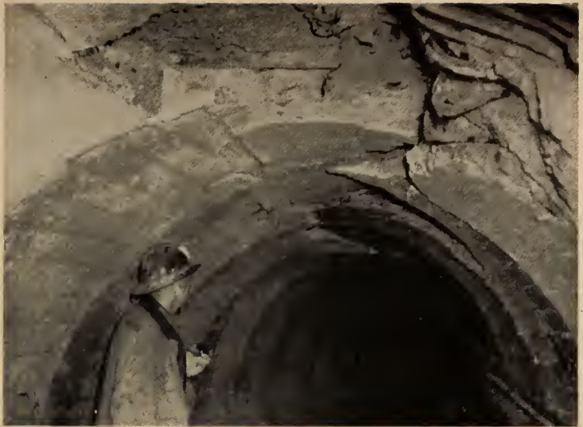
Fig. 4. Result of side pressure against a concrete lining in a small opening.
