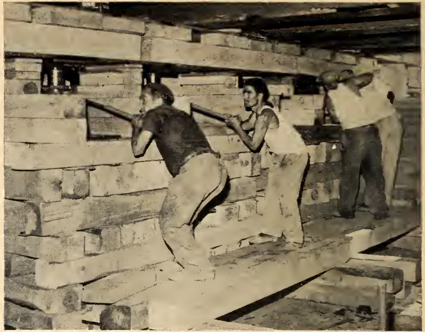
Fig. 2. The jacking crew at work: At this point, the building was being raised a further 18 in. and it was necessary for the men to work from staging.
