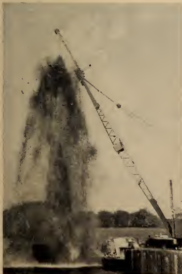
Fig. 4. "Blowing out" pipe pile after driving. An 80-foot-long "blow pipe" connected by hose to air receivers was inserted into the material inside the pipe pile. When pressure in the receivers built up to 110 pounds per square inch, gate valve was opened and sudden release of compressed air hurled rock and other material up to 80 ft. into the air. Cleaning pile to rock took about an hour.
