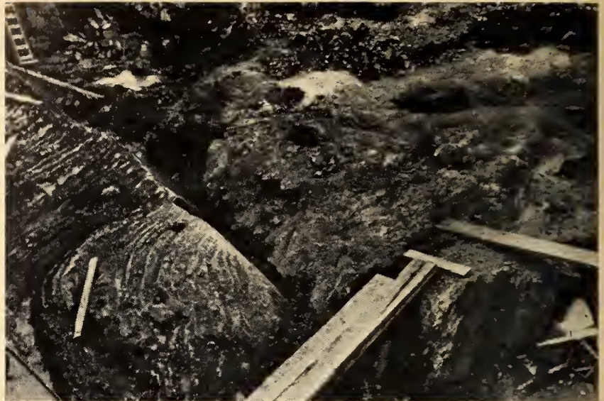
Fig. 5 Fault Zone — West End of Intake
