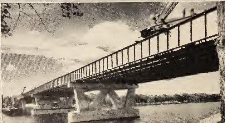
New Rivière des Prairies bridge, near Montreal, incorporates ten 225 ft. girders, each 70 tons; twenty of 212 ft. and many of smaller size.
