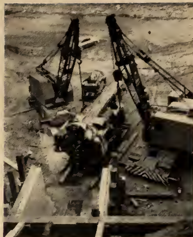
Foundation Co. of Canada develops high-speed tunnelling methods without the use of explosives. Start of operation on 11-ft. diameter 2½ mile long Humber Valley Trunk Sewer for the Municipality of Metropolitan Toronto.
