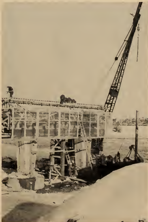
Fig. 5. Form work on one of the eight reinforced concrete piers. Plastic cover was devised to provide protection from freezing temperatures.
