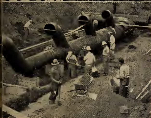
Manitoba Bridge crews erect and place into position 60", 48", 30" and 24" pipe for the cooling water.
