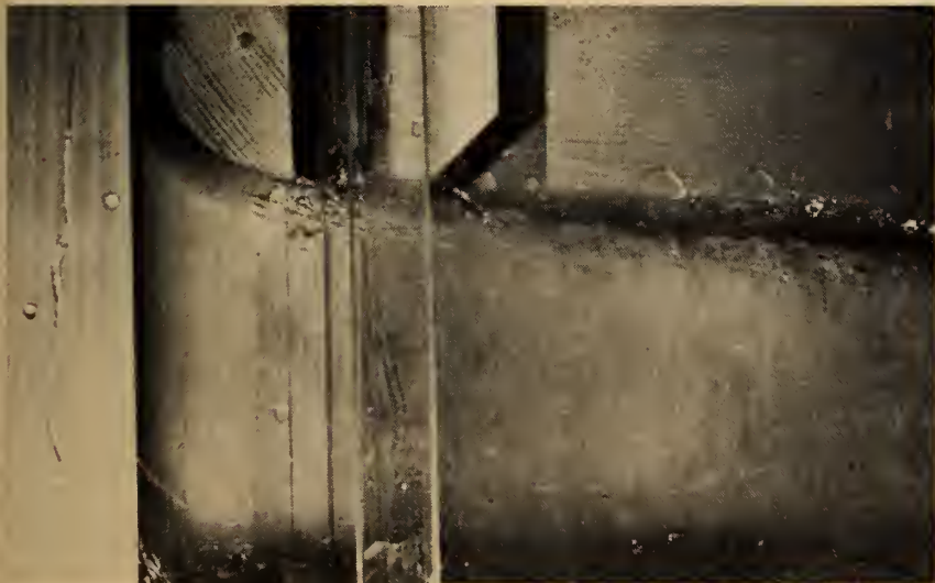
Fig. 1 Unsatisfactory Intake Transition
