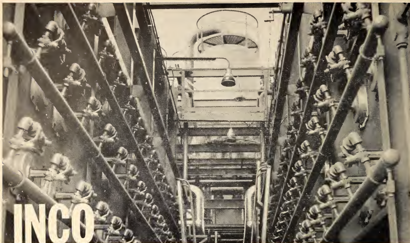
Incoloy tubing installed in a large furnace for converting ethane to ethylene. Very little tube maintenance or downtime required in spite of the 1500°F. temperature of operation. Tube wall temperatures are about 1700°F.
