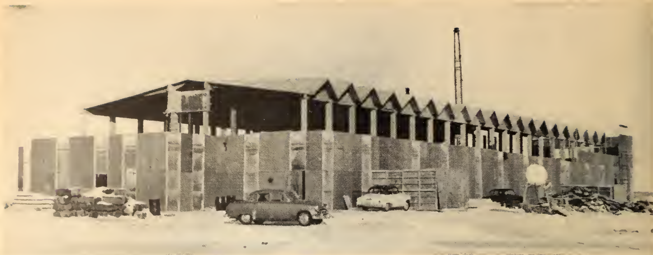
Fig. 2. Precast concrete roof and frame provide the structural portion of a lightweight enclosure (University of Saskatchewan).
