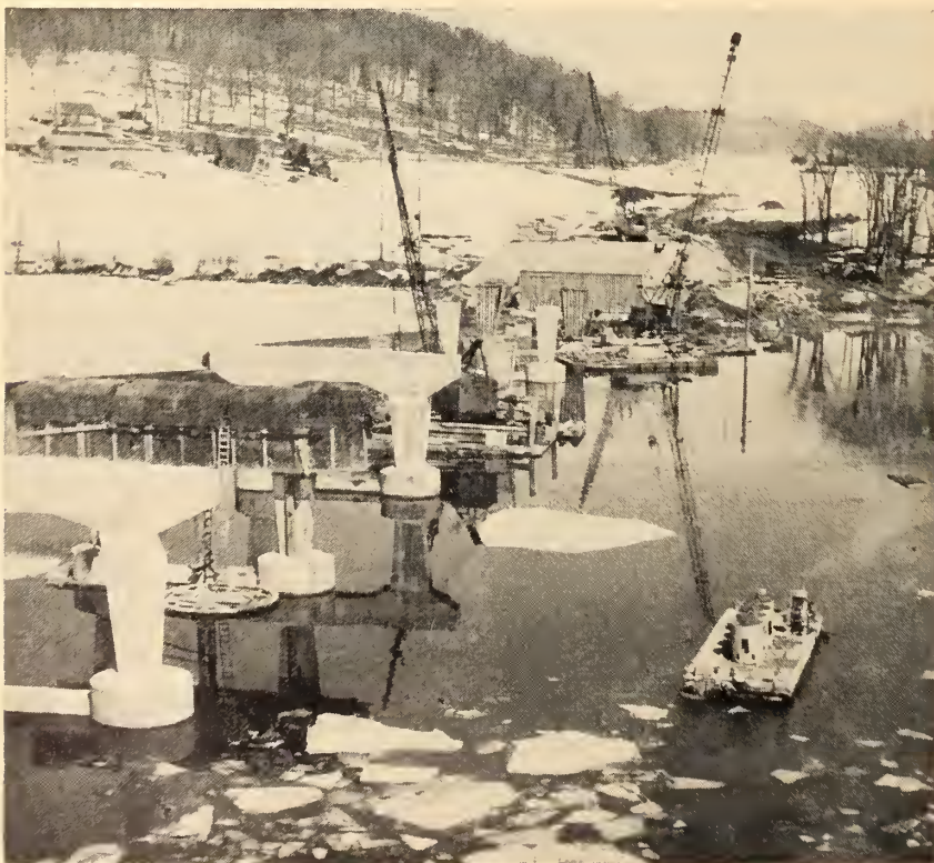
Fig. 3. Ferrying concrete from shore to piers. Concrete was mixed on shore, transferred via shuttle car to four bottom dump concrete buckets on cable-operated ferry.
