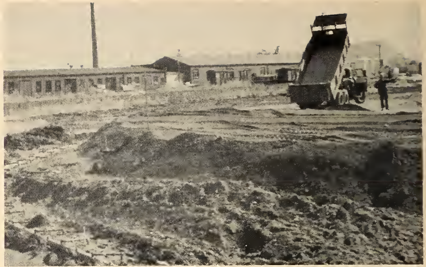
Fig. 5. Filling operations in progress at larger of two tanks. Part of wellpoint installation can be seen in left foreground. Pipe sticking out of fill is one of the settlement points.
