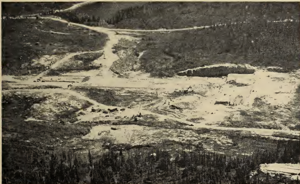
Fig. 2 Site preparation. Excavation in progress for smelter site. Beginning of road to townsite at upper left. June 11, 1956.
