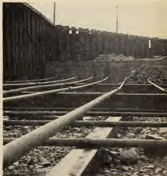
Fig. 4. Left: Arrangement of tie rods at nose of breakwater. Below: Tie rods at nose of dock (before tightening).
