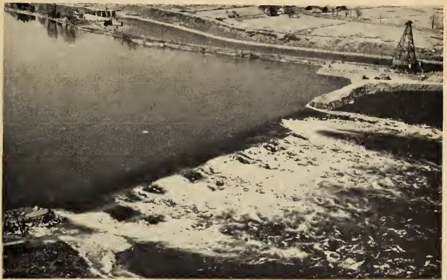
End of second stage construction of cofferdam 'E' by dumping rock from cableway skip; rockfill is built within 10 ft. of water surface. (PASNY)
