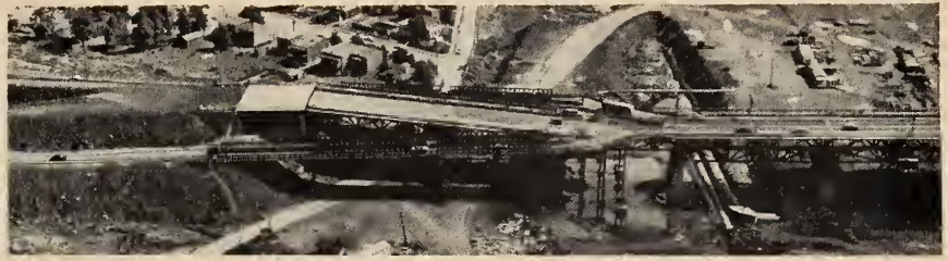
Fig. 4 Aerial view of Bailey bridges, new abutment, 65-ft. span and stage one jacking.
