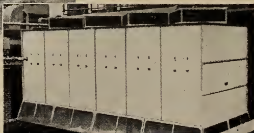
Evaporative condenser handling 330 tons of refrigeration
