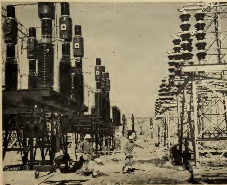
Fig. 2. Close-up view during construction of the 230 kv. switchyard at the St. Lawrence transformer station. The airblast circuit breakers are shown, left, parallel with the disconnecting switches. (Ontario Hydro photos.)
