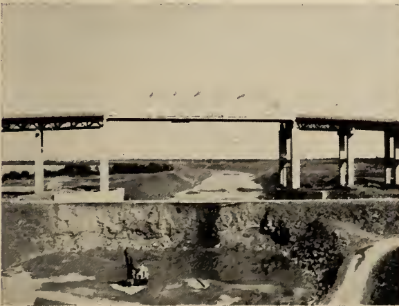
Fig. 18. Honore Mercier bridge crossing of canal. Remainder of temporary rock-fill for highway diversion in foreground.
