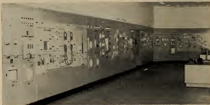
Fig. 4. Central treating plant.
