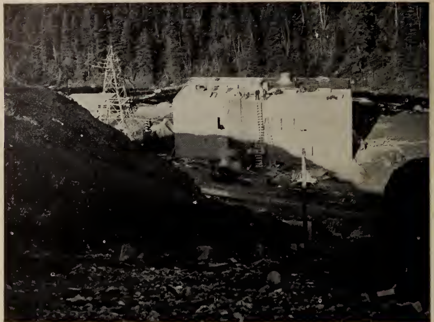
A view during construction of the penstock and powerhouse of the Bowater Paper Company hydro-electric station at Corner Brook, Newfoundland. The installation has a total capacity of 12,000 h.p. from two similar units.
