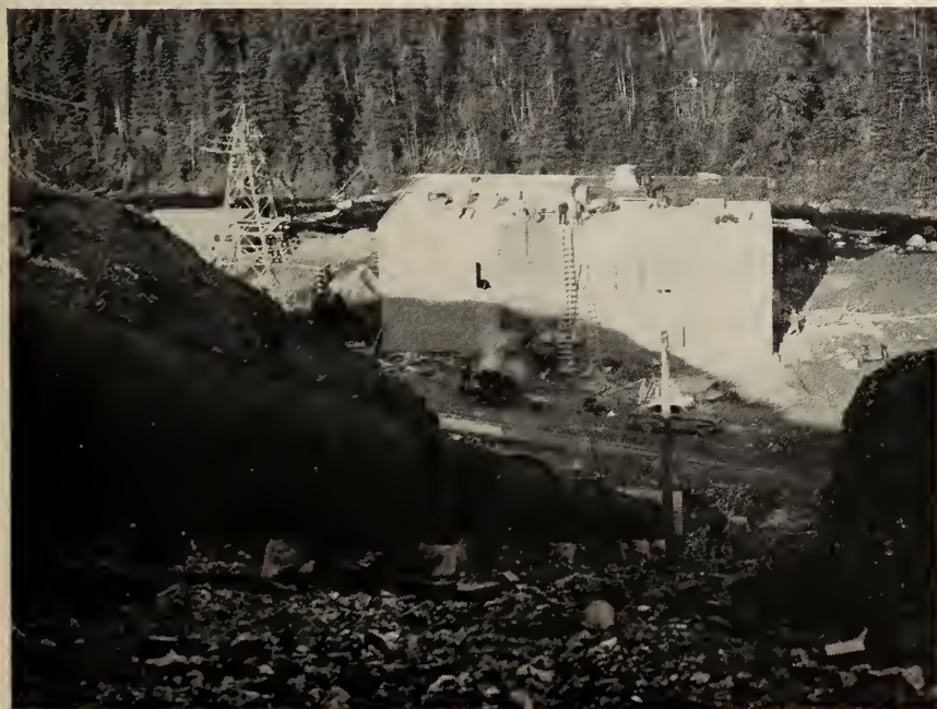
A section of the penstock and powerhouse under construction for Bowater Power Company at Corner Brook, Newfoundland. The two-million dollar project is nearly complete.
