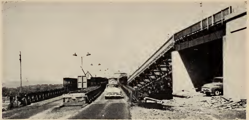
Fig. 6 South bound Bailey bridge route, 65-ft. span and addition to old abutment.
