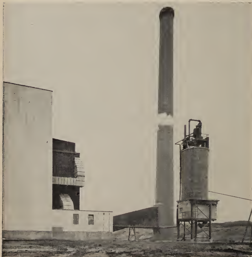
Fig. 9. Ash handling equipment and chimney.
