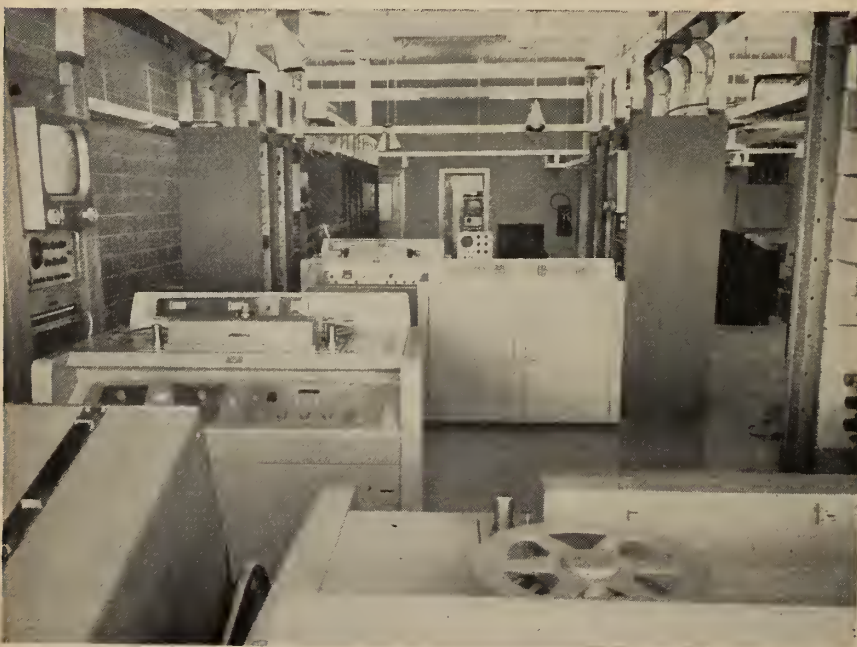
The video tape relay centre at Calgary.
