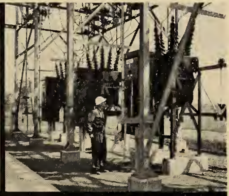
Three of six 46 Kv, 1000 MVA outdoor oil circuit breakers in the transformer station.
