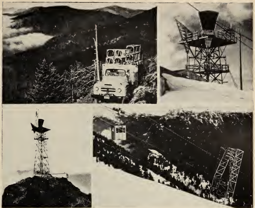
To build mountain-top relay stations for the Trans-Canada Telephone System's microwave network to the West Coast, roads had to be cut through mountains, even above cloud level (upper left). At Hedley, B.C., a mountain top was blasted away to form a site (lower left). So high are many of the sites that buildings are often buried in snow (upper right). Access roads could not be built at two sites, so aerial tramways were constructed. The Dog Mountain tramway (lower right) is one of the biggest in the world—more than two miles—with a lift of 4,400 ft.
