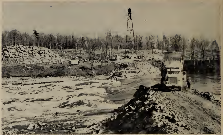
Construction of rockfill section of cofferdam stage 3, by truck dumping of rock. (HEPCO)
