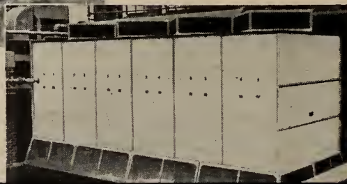
Evaporative condenser handling 330 tons of refrigeration
