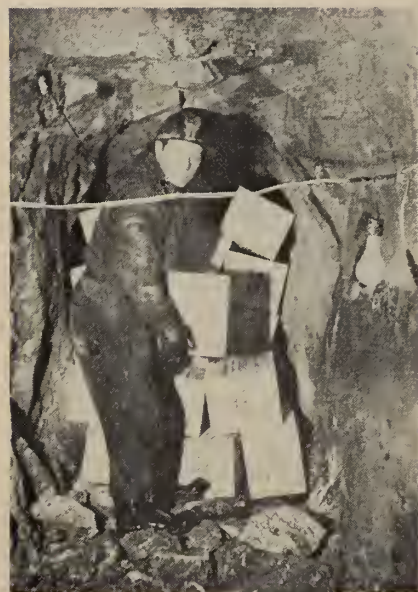
Fig. 12 (left). McCormick Dam. Loading south plug coyotes of unwatering tunnel with explosive.
