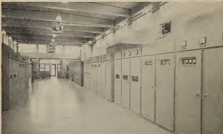
Fig. 17. Transmitter hall at Cloverdale.
