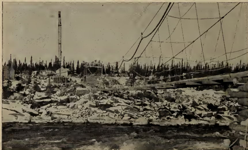
A foot-bridge over the Hamilton River and a 25-ton cable-way, under construction at the left, provide access to the 4-million h.p. Hamilton Falls project.
