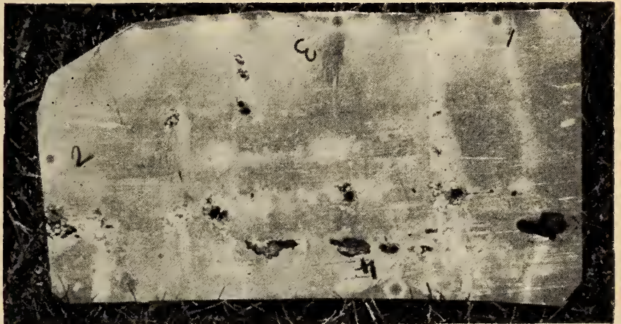
Fig. 12. Close-up view of reverse side of parapet flashing. Note ghosts of tile ribs and mortar joints. Sheet was not back-painted.
