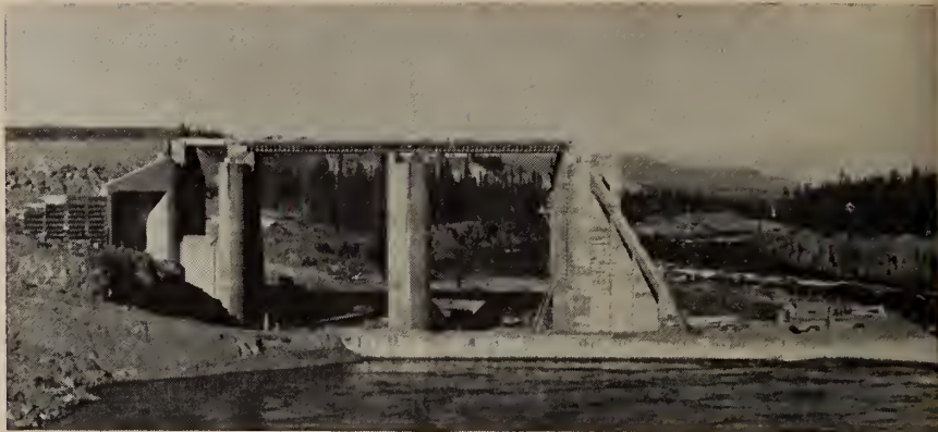
The Whitehorse Rapids project on the Yukon River, shown here during construction, comprises two 7500 h.p. units, with provision for further expansion.
