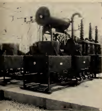
161 KV, 115 MVA main step-down transformer. This is one of a bank of English Electric transformers handling incoming power from the generating station at Manicouagan.
