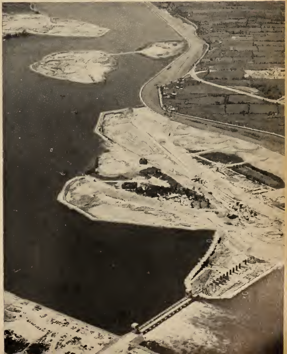
Iroquois dam (right). Looking upstream at the dam in the foreground, Iroquois lock on Iroquois Point; Toussaints Island and Sparrowhawk Point in the distance; showing progress in June.
