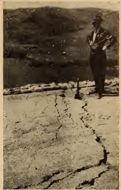
Fig. 6. Cracks in crest of homogeneous earth dam.
