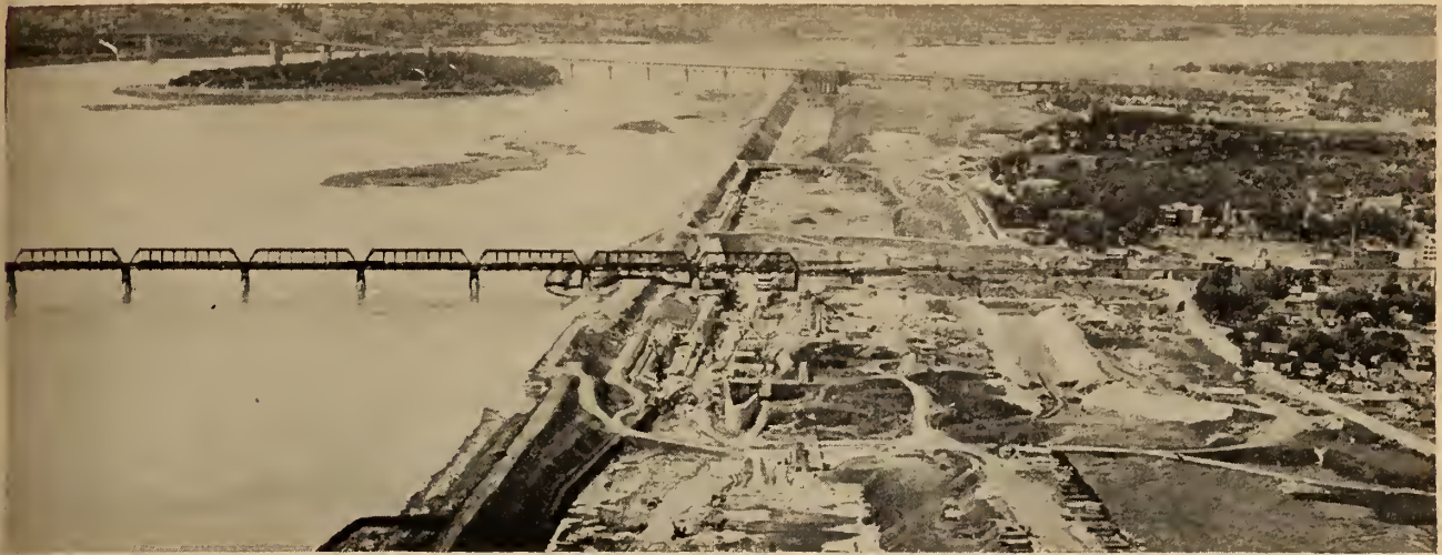
Fig. 3. Victoria Bridge, showing span No. 25 in way of St. Lambert Lock under construction.
