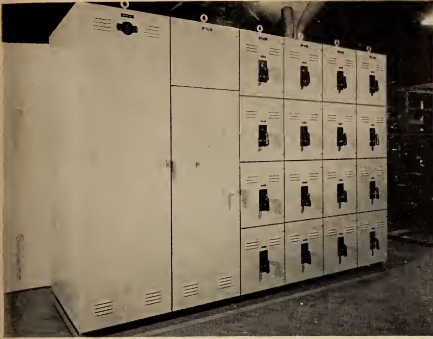
Typical cubicle arrangement; circuit breaker, lighting, and heating cubicles.
