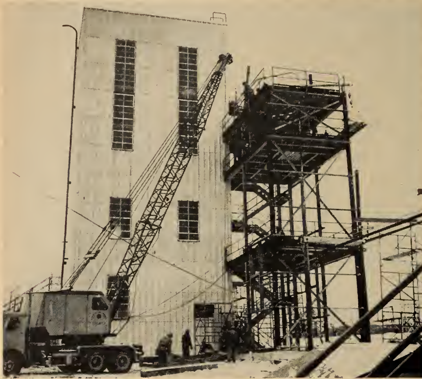
Extensive construction and development programs call for increasing supplies of explosives. Above is the acid building of a commercial explosives plant near North Bay, Ont., under construction in 1956. (Photo: Du Pont of Canada.)
