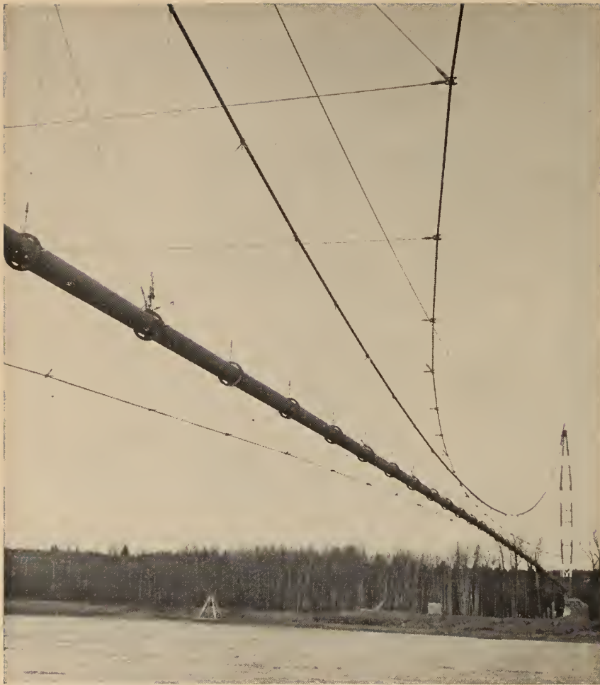
Cobweb of wire rope carries the 30-in. tube of Westcoast Transmission Company's gas pipeline over the Fraser River at Shelley, B.C.
