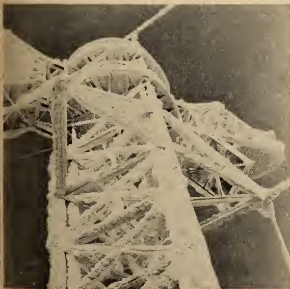
Rime ice on guyed tower late in 1956.
