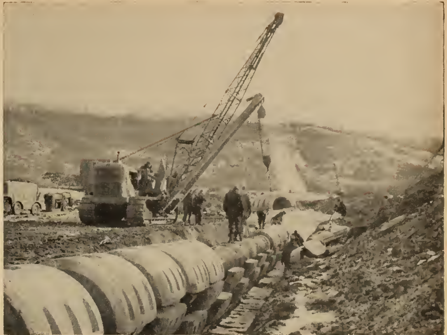
The Trans Canada natural gas line has 6000-lb. concrete weights attached to the 260-ft. section that crosses the Assiniboine river at Miniota, Man. (Photo: Trans-Canada Pipe Lines Limited.)
