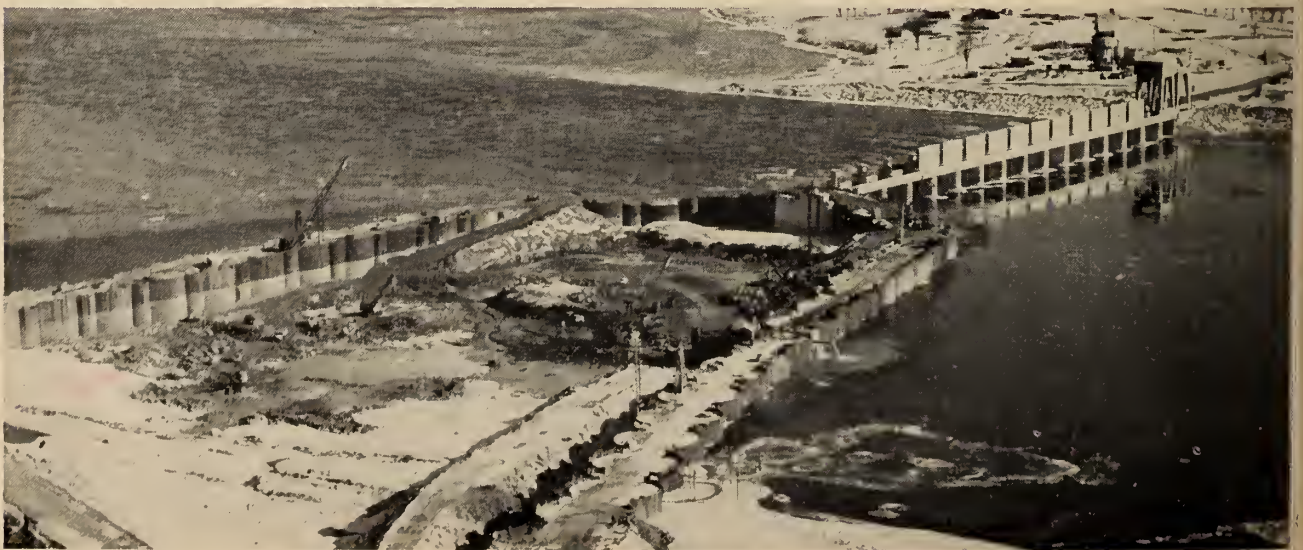
Iroquois dam. Excavation operations are being carried out in the Stage II construction area.
