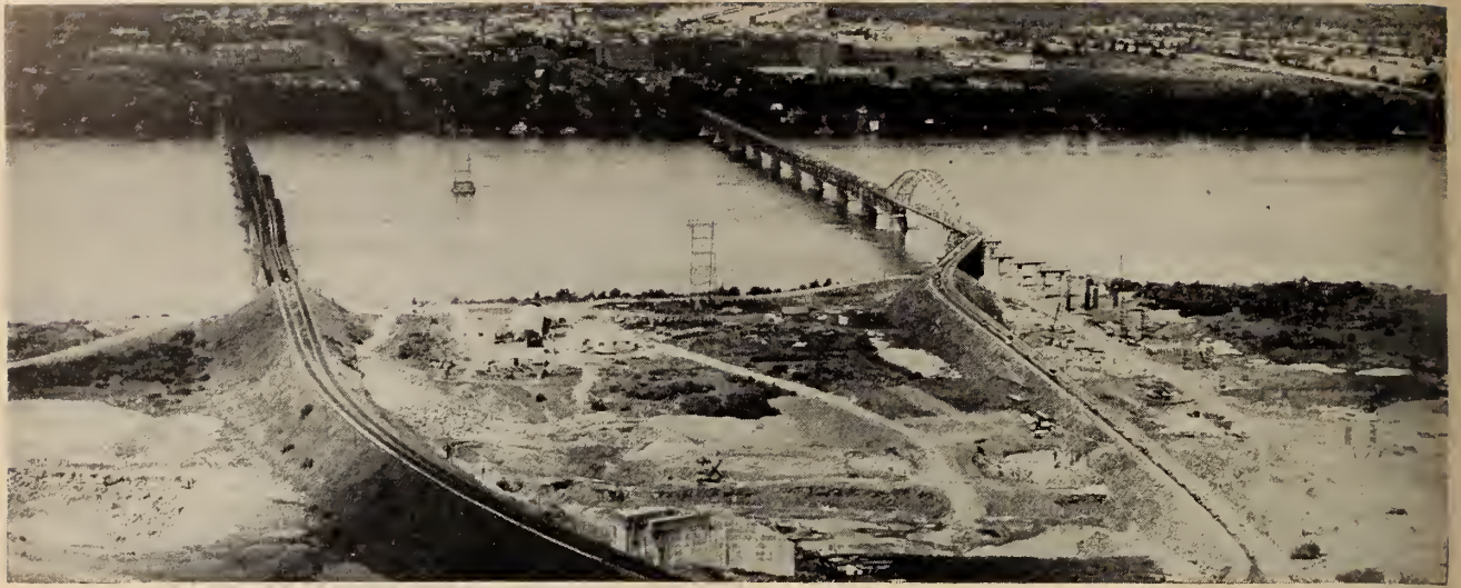
Fig. 4. Honore Mercier Highway Bridge and Canadian Pacific Railway bridge near Caughnawaga. Highway turnoff in operation. New piers for both bridges under way.
