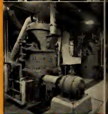
View showing Bowl mill pulverizers which fire the C-E, HT boilers at Gagetown.
