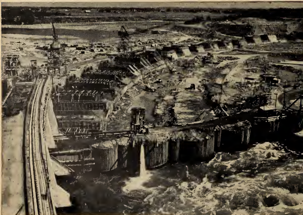
The Long Sault Dam. The shape of the final structure is clearly outlined in this view of stage II construction taken from atop one of the gantry cranes.
