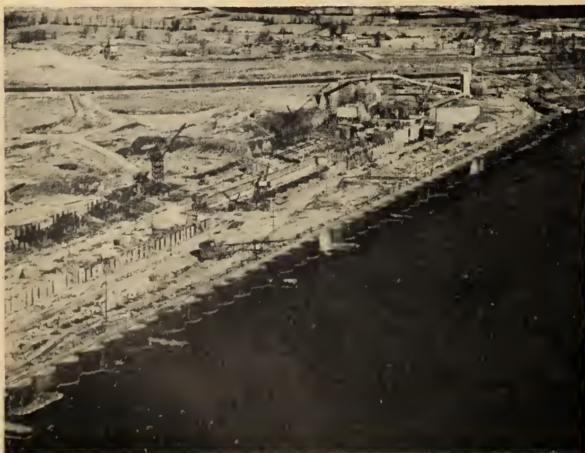
The powerhouse of the St. Lawrence seaway project under construction in December 1956. Both American and Canadian sections are shown, with the former in the foreground.
