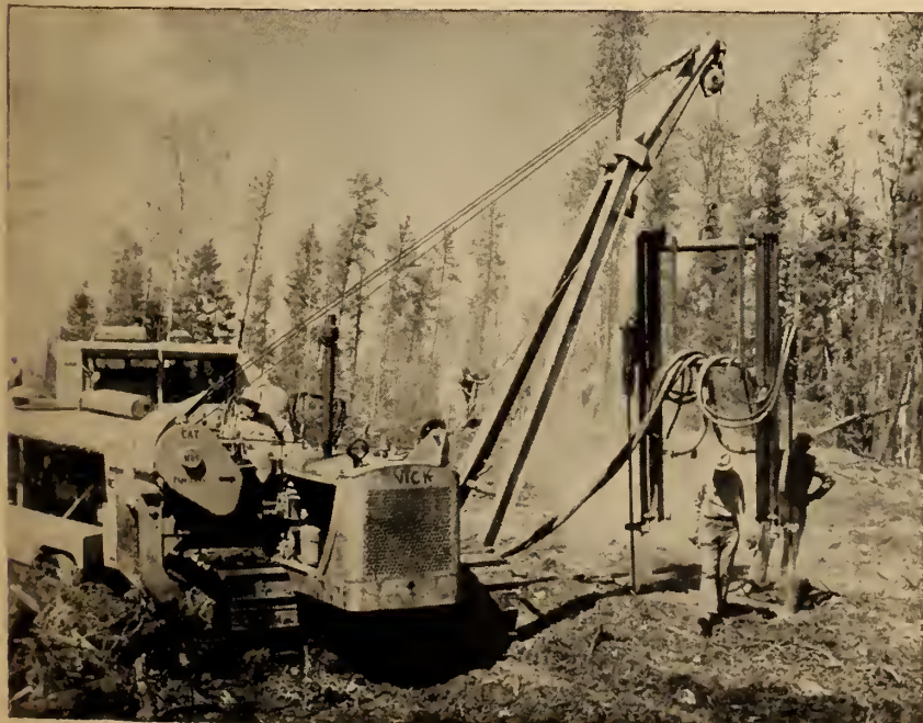
Jack hammers and wagon drills, operated by compressed air, preparing right-of-way in Eastern Manitoba.
