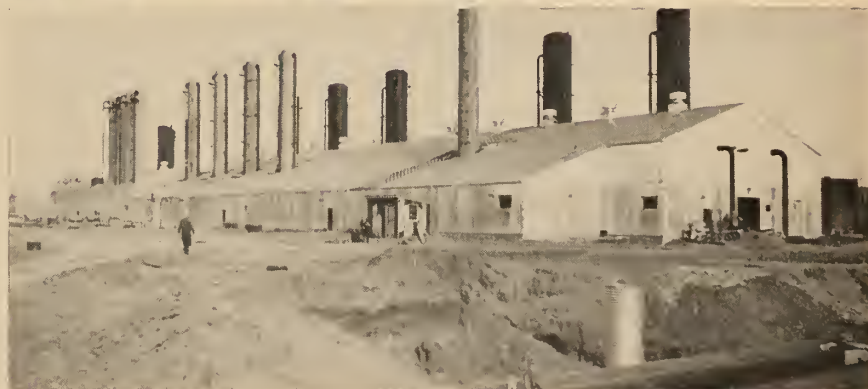
Top to bottom: Laying pipe for the gas gathering system; welding the gas pipeline; a general view of the refinery at Taylor, B.C.
