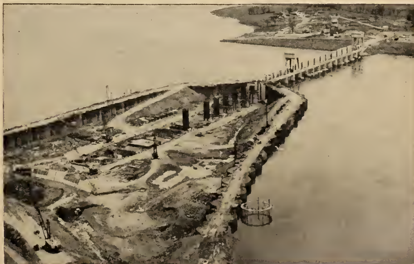
Iroquois dam. Looking downstream from the Canadian mainland on Iroquois Point, Stage II construction in the foreground.
