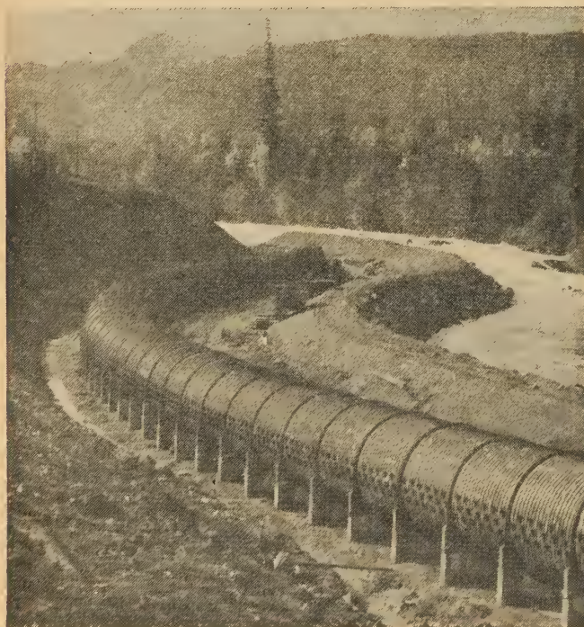
"Pacpipe" continuous Wood Stave Pipe line at B.C. Power Commission's Puntledge River Development.
