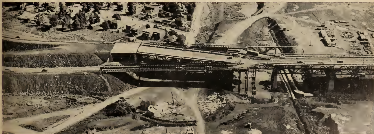
Fig. 1. Jacques Cartier Bridge turnoffs. New abutment and 65 ft. span in place. Stage one jacking of spans No. 1 and No. 2, nearly complete.
