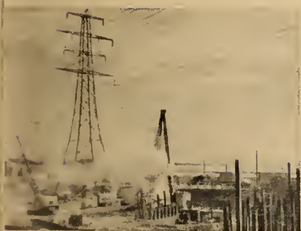
Shown above is a general view of the bridge building activity. Work is progressing on schedule.
