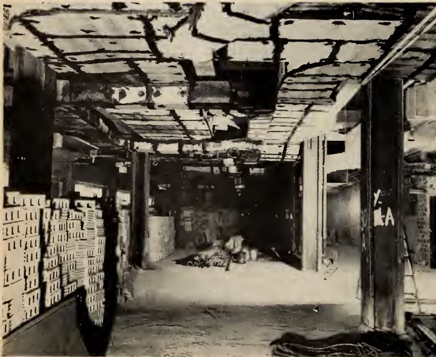
Fig. 4. View of corridor to private dining rooms, showing specific example of crowding of ductwork in certain areas to maintain headroom.
