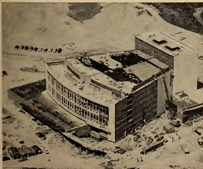
Seen during its construction is the new civic auditorium at Calgary. A duplicate auditorium was also built at Edmonton during 1956. Some 1300 tons of steelwork were used in each.
