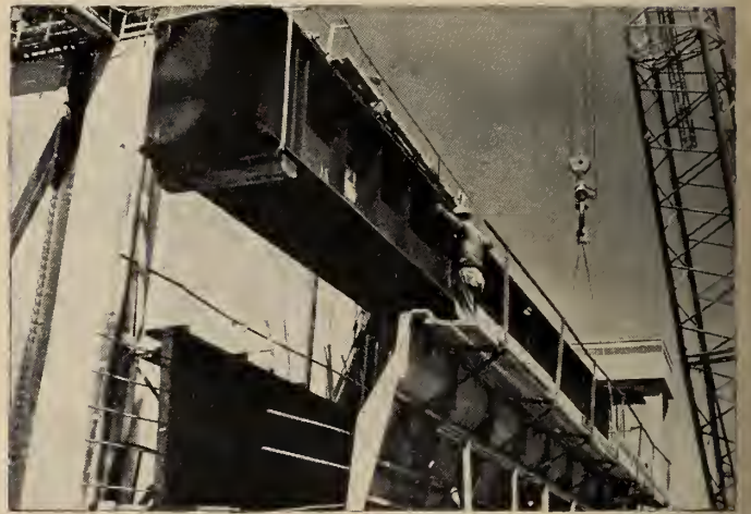
Massena intake (top), as blocks of concrete approached the final grade in August.
