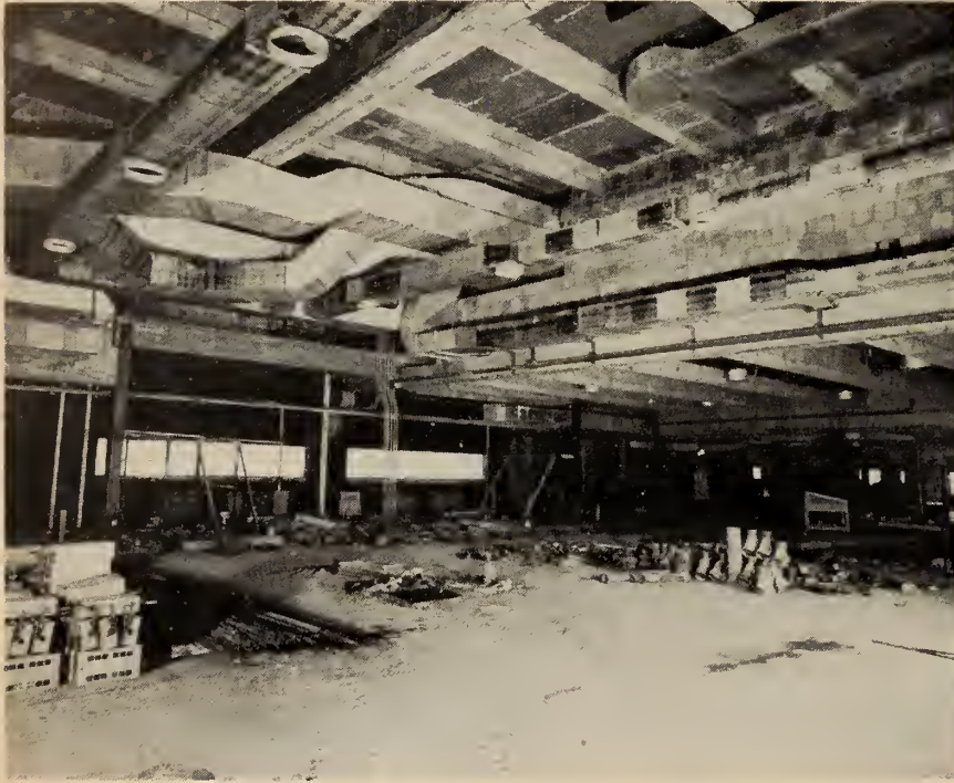
Fig. 3. View of largest of banquet rooms under construction, showing installation of standard low-pressure air conditioning ducts.
