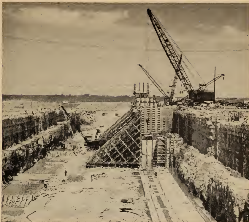
Workmen are dwarfed by the great walls of rock where construction of the lower Beauharnois Lock is under way. Here ships will be raised 42 feet into a canal about a mile in length which will lead them to the Upper Beauharnois lock and a second 42 foot lift, after which they will enter into the Beauharnois canal.
