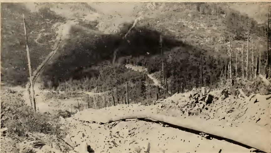
Top to bottom: Boom tractors handling pipe (wrapping machinery in the background); lowering pipe into ditch dredged in Pine River, Pine Pass, B.C., Aug., 1956; view from top of Angels Peak, looking downstream (July 1956).
