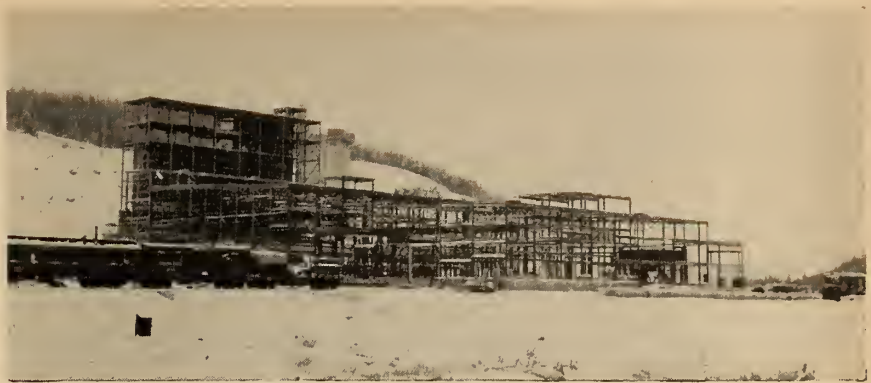
The framework of the Geco Mine mill buildings, at Manitouwadge, Ontario, where large copper and zinc deposits have been discovered and are now being developed, thus opening up another new area. (Photo: Ontario Department of Mines.)
