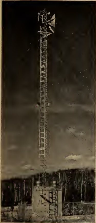
A tower in the micro-wave communication system linking the Bersimis No. 1 and No. 2 sites, Charlesbourg, Montreal, and Beauharnois. ( Hydro-Québec. )
