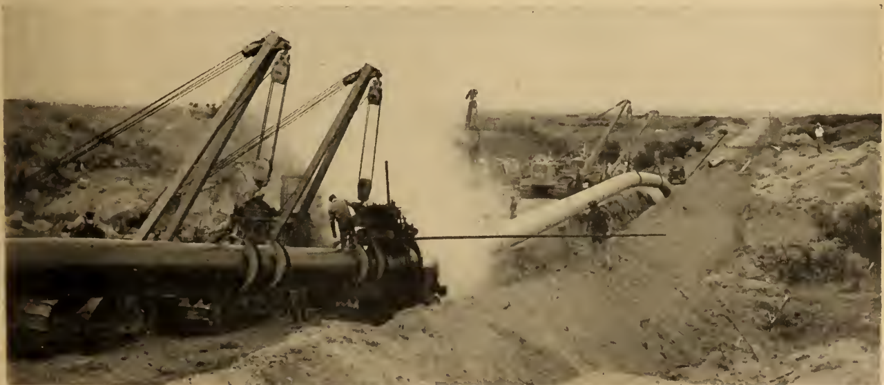
Laying the Trans Canada natural gas line through the Great Sand Hills of western Saskatchewan. The 34-inch line is coated, against corrosion, and wrapped with fibreglass and kraft paper. In the background, the trench has already been back-filled. (Photo: Trans-Canada Pipe Lines Limited.)
