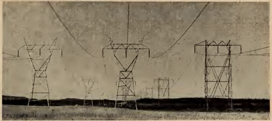
Fig. 4. Three 230 kv. single circuit transmission lines. Two overhead ground wires. Seen from right to left, respectively, are lines constructed in 1934, 1950, and 1955. (The Shawinigan Water and Power Company)
