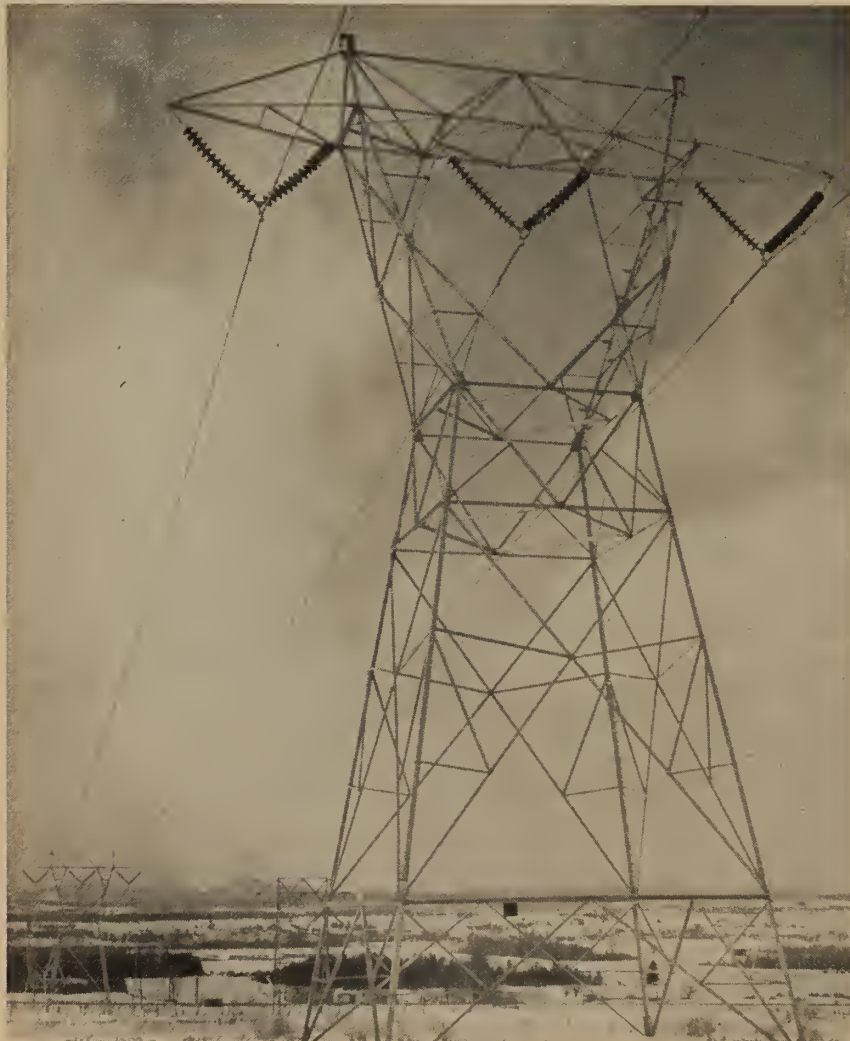
Fig. 3. 230 kv. single circuit V-strung suspension structure with 16 ft. 6 in. phase spacing. Two overhead ground wires. (The Shawinigan Water and Power Company)
