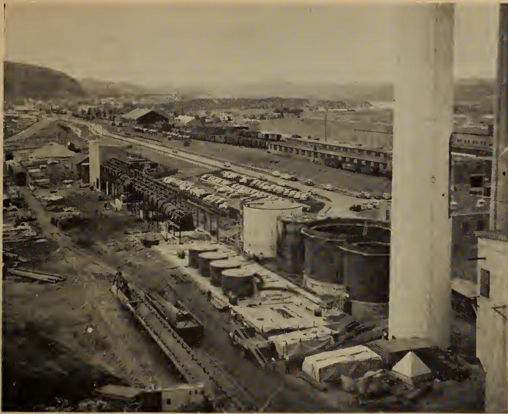
Fig. 4. New 250-ft. concrete brick-lined stack for the recovery furnace. Tanks connected with the caustic plant are seen under construction, and beyond this the lime kiln has been erected. The structural steel frame under the lime kiln is for a roof, to be installed, but no side walls will be provided despite temperatures reaching 50 deg. below zero. Heat radiated from the kiln, which never stops, keeps the ground dry under the roof.
