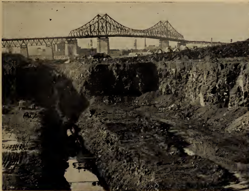
Fig. 10. Longueuil water supply intake being placed below the St. Lambert lock approach channel. The Jacques Cartier bridge is seen in the background.
