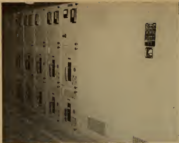
Fig. 11. Double ended 2400/600 volt unit sub-station in the power house.
