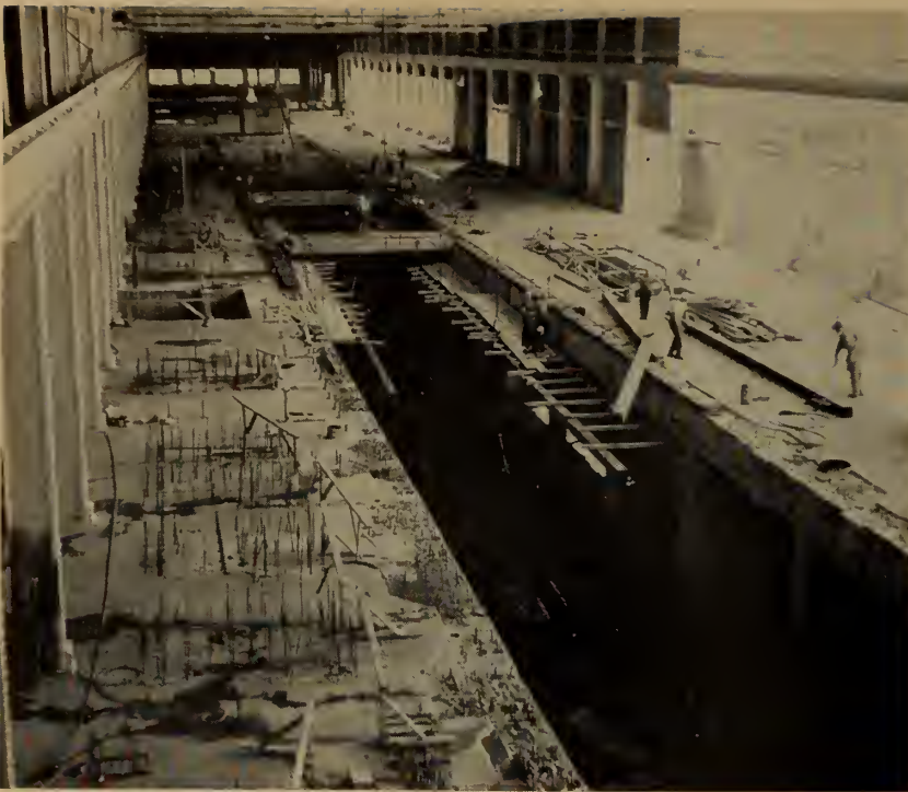
Fig. 10. Looking down through the machine room, showing the sole plates being installed for the side frames of the paper machine. The basement floor had not yet been poured. Reinforcing steel projecting through the floor (foreground) is to take the drives for the various machine sections.
