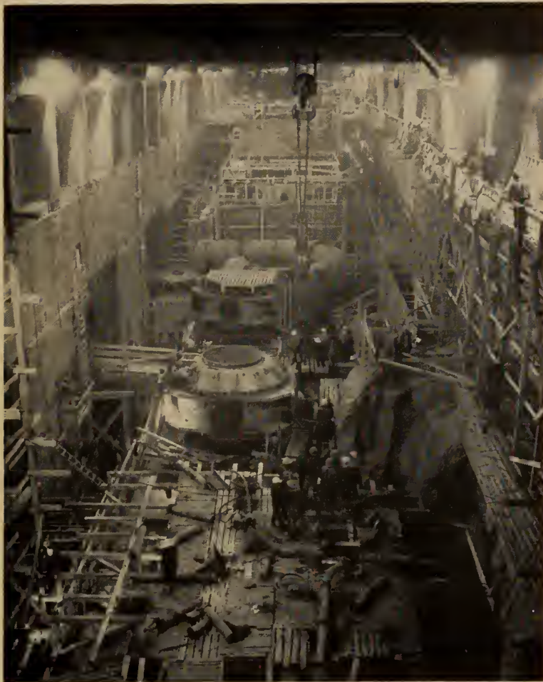
The underground power house of the Bersimis Power Development. This cavern is 565 feet long, 65 feet wide and 80 feet high. It houses eight Francis turbines—fifty-five feet apart—each rated at 150,000 h.p. under a 785-foot head at 277 r.p.m. The power house was constructed by Dufresne Engineering Company Limited.
