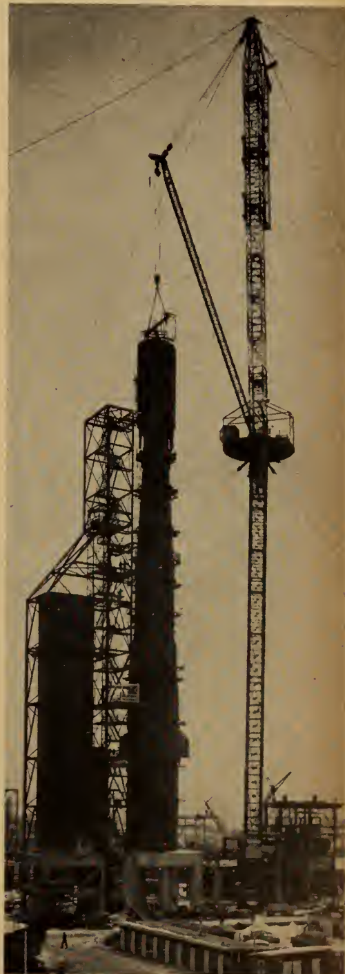
Fig. 8. The top unit of the catalytic cracker, the 85-ton catalyst disengager, is finally placed in position after a single lift of over 300 feet.
