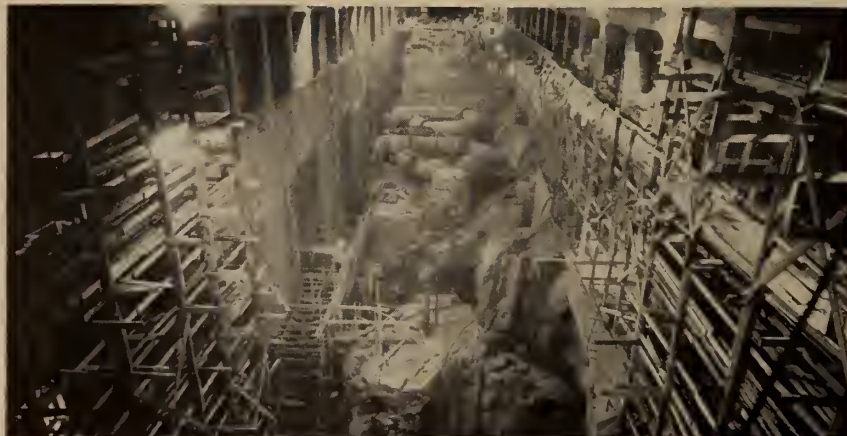
Fig. 13. General view of power house showing scroll cases No. 2 and 3 in position.
