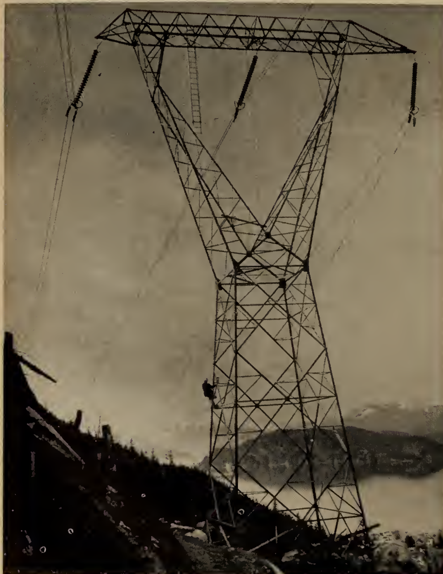
Fig. 7. 345 kv. single circuit suspension structure; bundled conductors. Bridge River No. 2 transmission line. (B.C. Electric Co. Ltd.)
