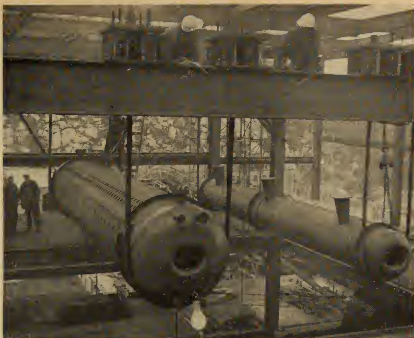
Fig. 8. Recovery furnace required a 10-storey extension to the existing building; here, the top drums have just been installed.
