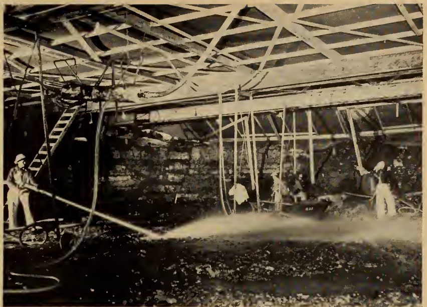
Iroquois dam. Rock foundation is prepared for concrete by cleaning surface with high pressure streams of water.
