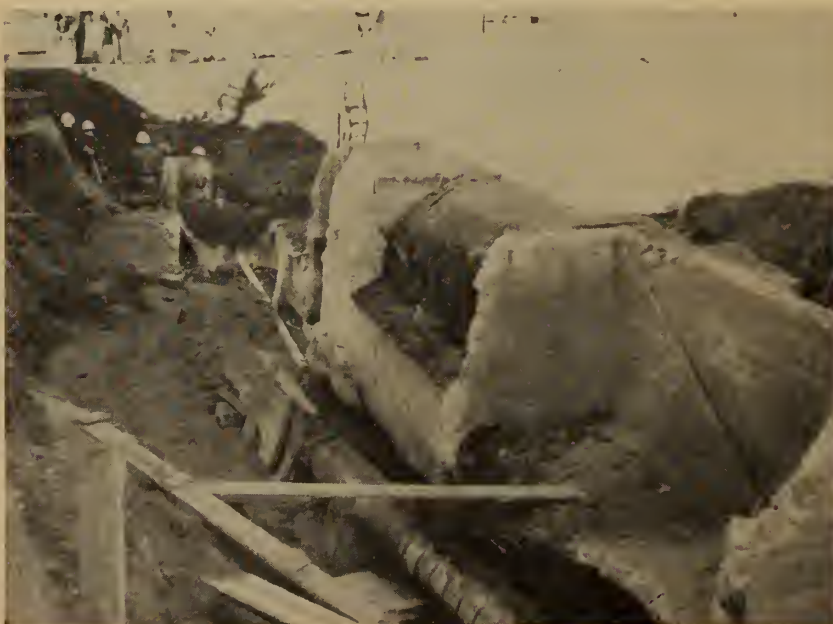
Fig. 1. Before starting excavation for the sewer shown here it appeared that there was virgin soil in this area. Excavation revealed an old concrete Venturi flume used at some time to measure effluent.
