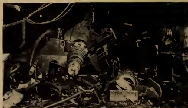
Fig. 27. General view of failure of 60 Mw. machine.
