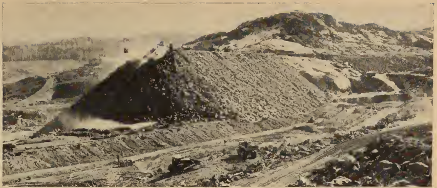
Fig. 10. South end of Lac Cassé dam under construction, showing monitor jets at work.
