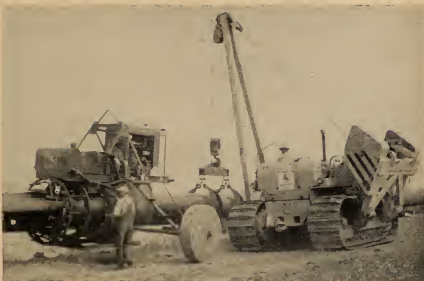
The cleaning and priming machine rides the pipe under its own power. At the front revolving knives scrape dirt and rust from the pipe, after which revolving brushes coat the pipe with a priming base for the coal tar coating.
