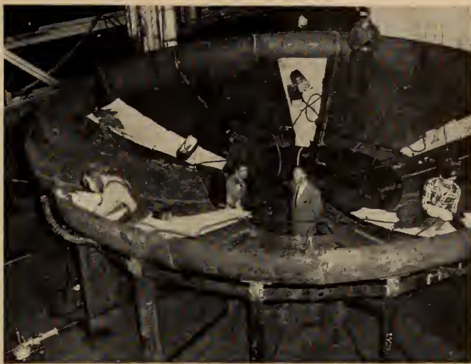
Fig. 4. Large jigs were built for the assembly of the heads for the catalytic cracking unit. Welders worked from rotating asbestos hammocks inside the head. Seams were pre-heated by controlled propane burners, of which a closer view is seen in the left-hand picture.
