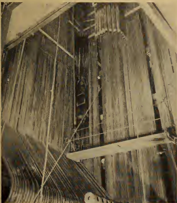
Fig. 7. Looking up through the partially assembled water cooled walls of the 250,000-lb./hr. power boiler. Arrangement of the tubing to allow installation of a tangential type burner is shown at the centre of the picture.
