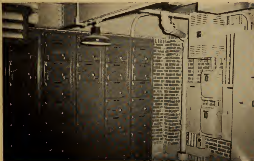
Fig. 16. Motor control unit in one of the process buildings.
