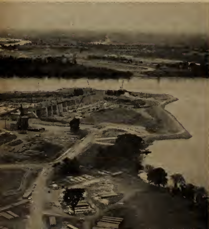
Relationship between the Iroquois control dam and the Iroquois lock is shown here. The channel, still open over to Iroquois Point, soon will be cofferdammed and the water allowed to run through the sluices. The wall of the approach from upstream to the Iroquois lock, being built in Canada, is at upper left. Navigation uses the Galop Canal, which may be seen behind the lock.
