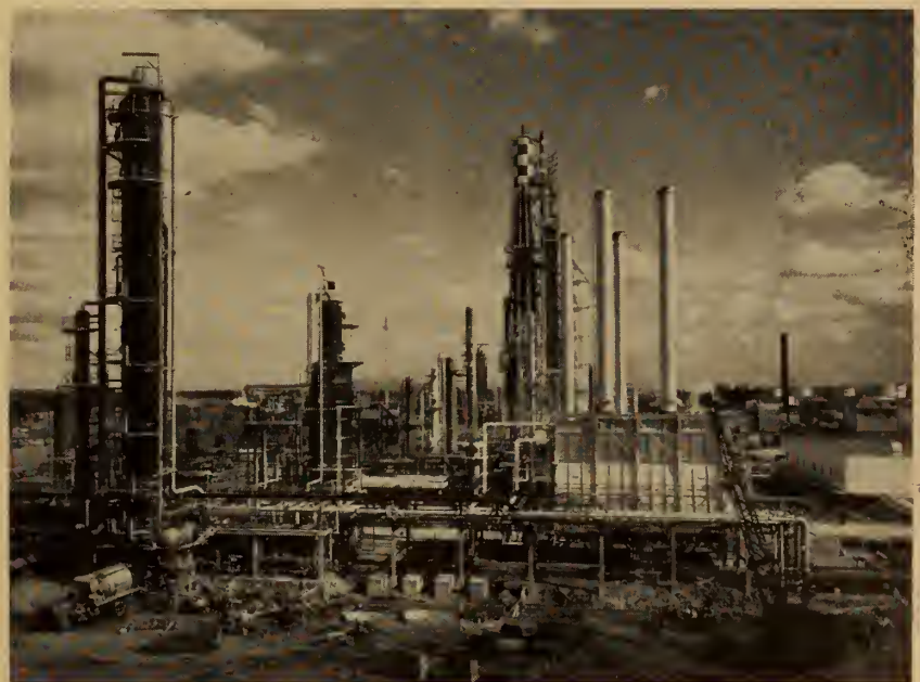
Fig. 2. Crude tower, stripper, and furnace. Excavations and forms in foreground for coke unit. Control house at extreme right.
