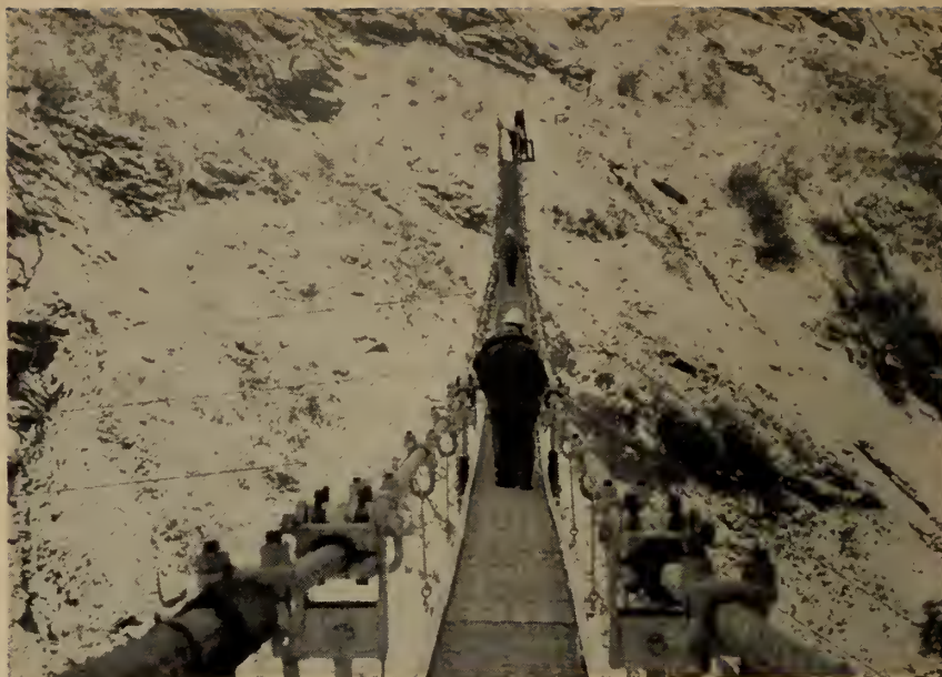
Fig. 12. View from catwalk looking towards north-east anchorages during hook-up of last conductor. Cable car can be seen at far end of catwalk.
