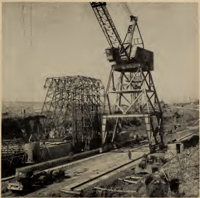
Gantry placing concrete for first section of the mile-long walls of Iroquois locks. Crane swings bucket of concrete over forms. Work is now well advanced.
