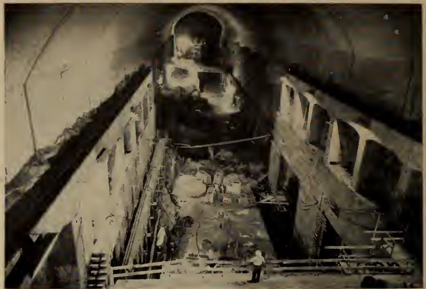
Fig. 12. General view of underground power house showing arch-roof, crane rails, beams, and columns. At centre, the supports for unit No. 2 scroll case.
