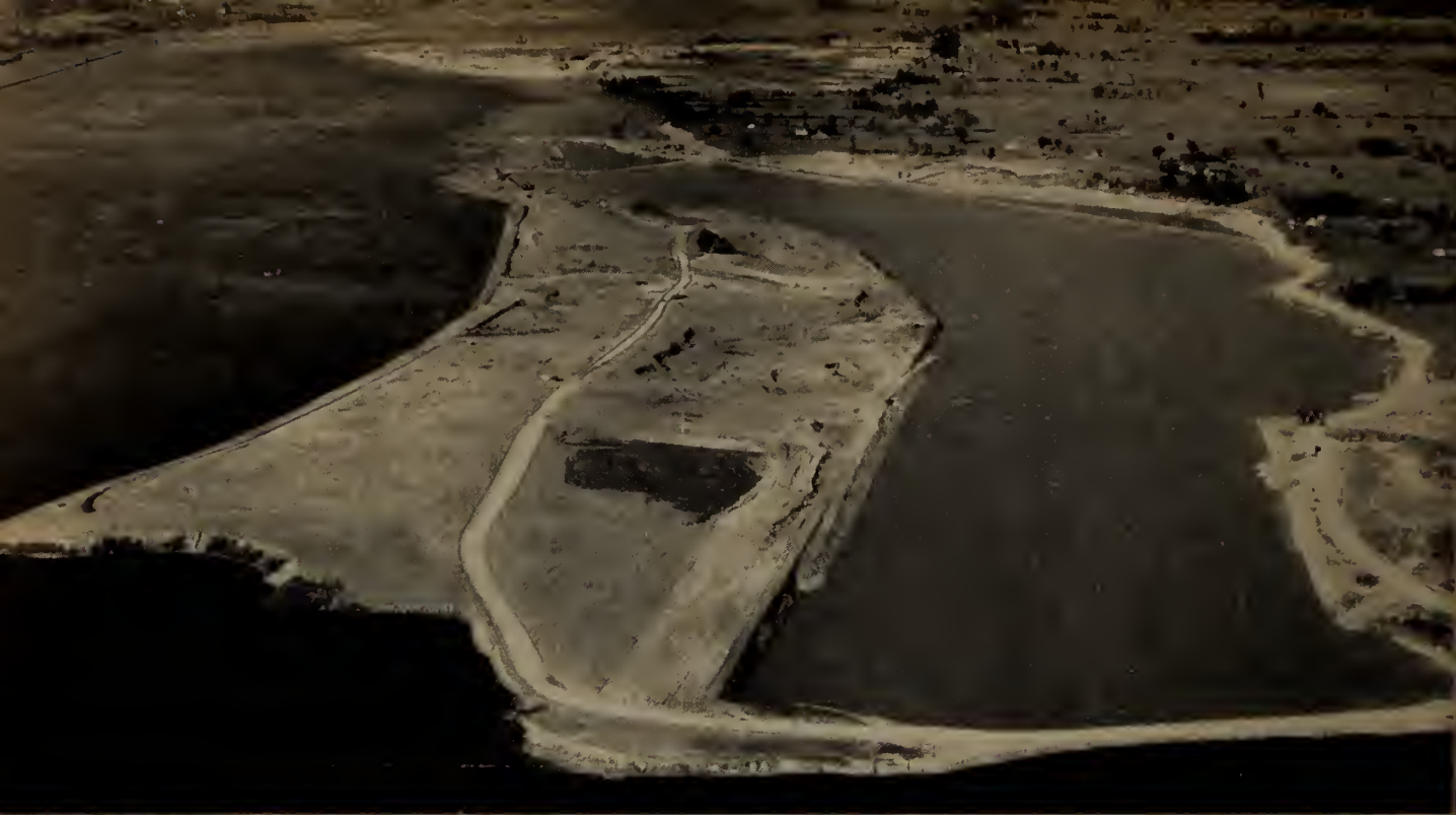
Looking downstream at Galop Island south channel; excavation complete and area flooded. Cleaning up at downstream end is seen still in progress.
