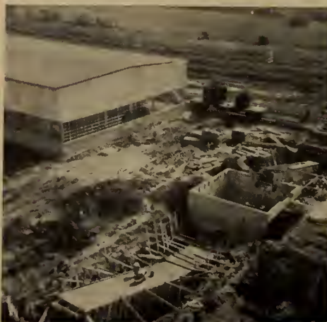
Fig. 1. Site of the primary crusher at Cadomin (left) with formwork for loading bay. Right, secondary crusher under construction.
