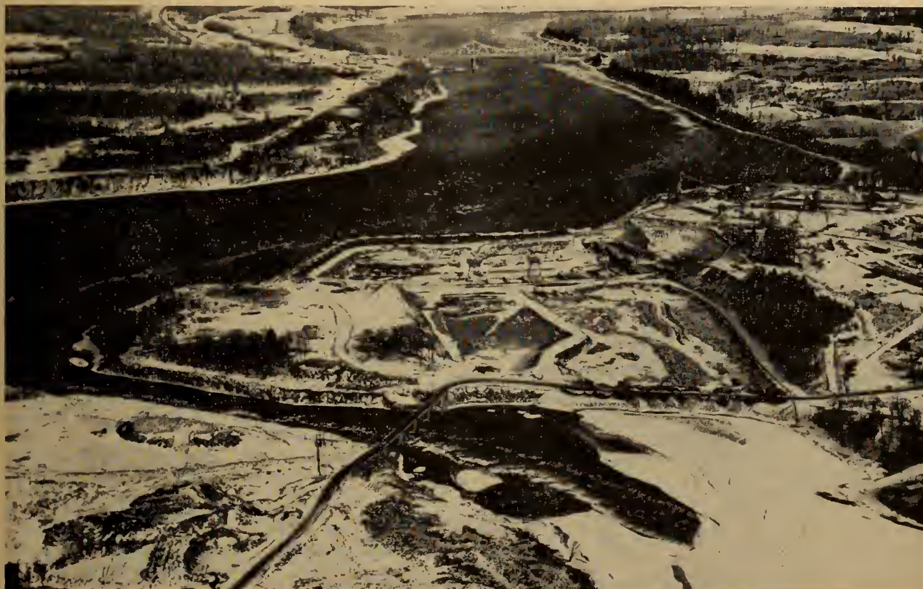
Long Sault Dam. The south channel is covered with ice and construction in the dam area lies dormant until spring.
