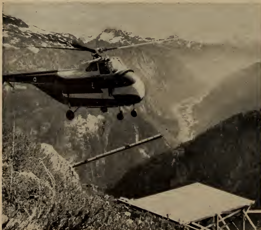
Fig. 13. Sikorsky S-55 helicopter ready to drop 850-lb. load of two 2-1/2-in. dia. x 25-ft. long anchor bolts at platform near north-east anchorages of cross suspension.
