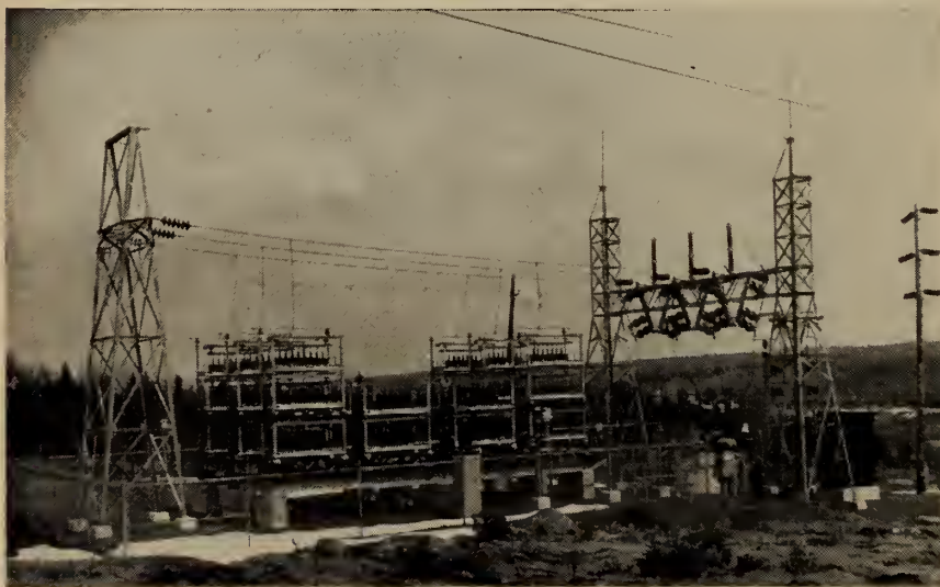
A 9,000 kilovar 60,000-volt capacitor installation at a sub-station in the asbestos mining district of Quebec. Power transmission is of major concern to the engineer.
