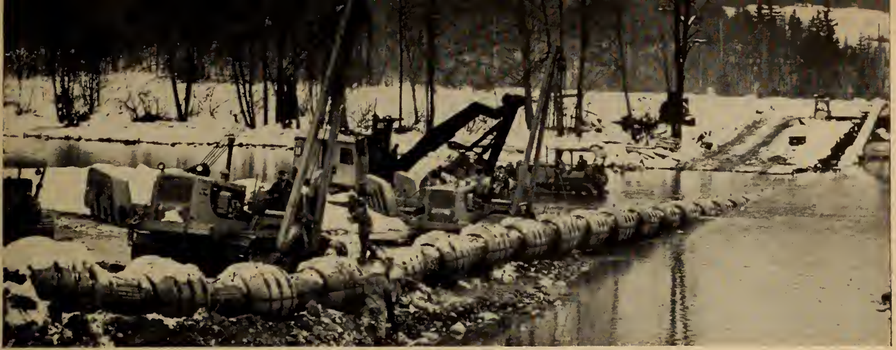
Work on the Westcoast-Transmission Co. Ltd., gas pipeline. The crossing of the Coquihalla River, near Hope, B.C.
