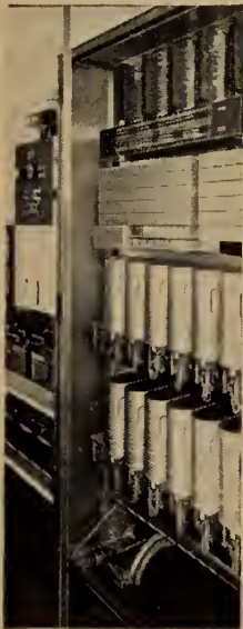
PBX (Private Branch Exchange)—a dial switchboard system which is faster and more efficient.
