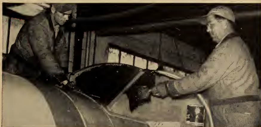
FOR THE TANK SPLASH AREA (shown above), a black neoprene coating (brush) is used. For the rest of the tank, a grey coating is applied (spray).
