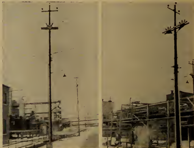
Fig. 12. 13-kv. poles and circuit.
