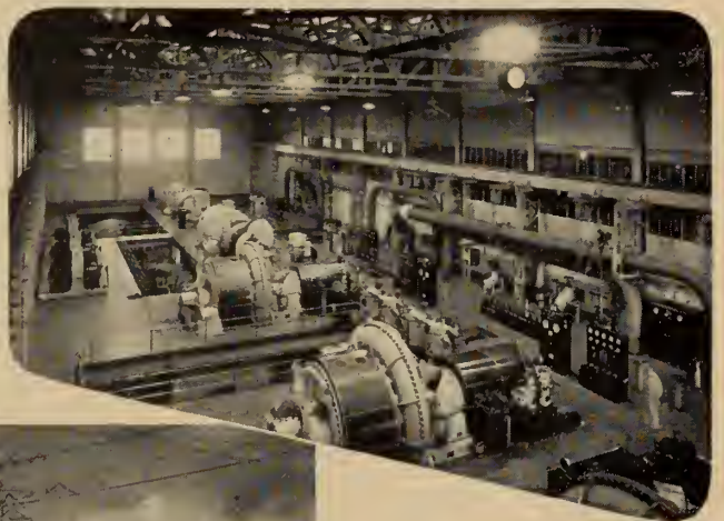
Four turbo-blowers (duty of each blower 80,000 cubic feet of free air per minute delivered at 30 lbs. per square inch pressure.)
