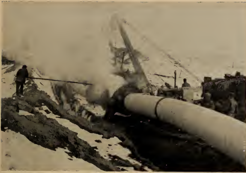
The natural gas line from Alberta to Eastern Canada moves ahead despite winter working conditions.
