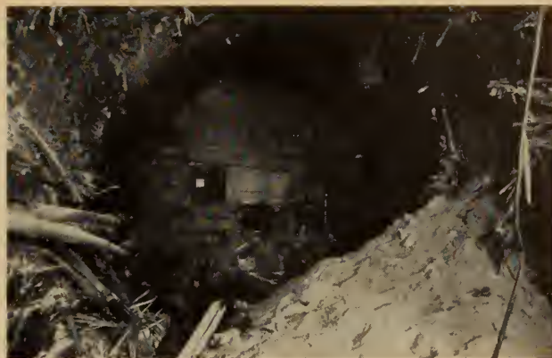
Fig. 28. Damage to timber lining.
