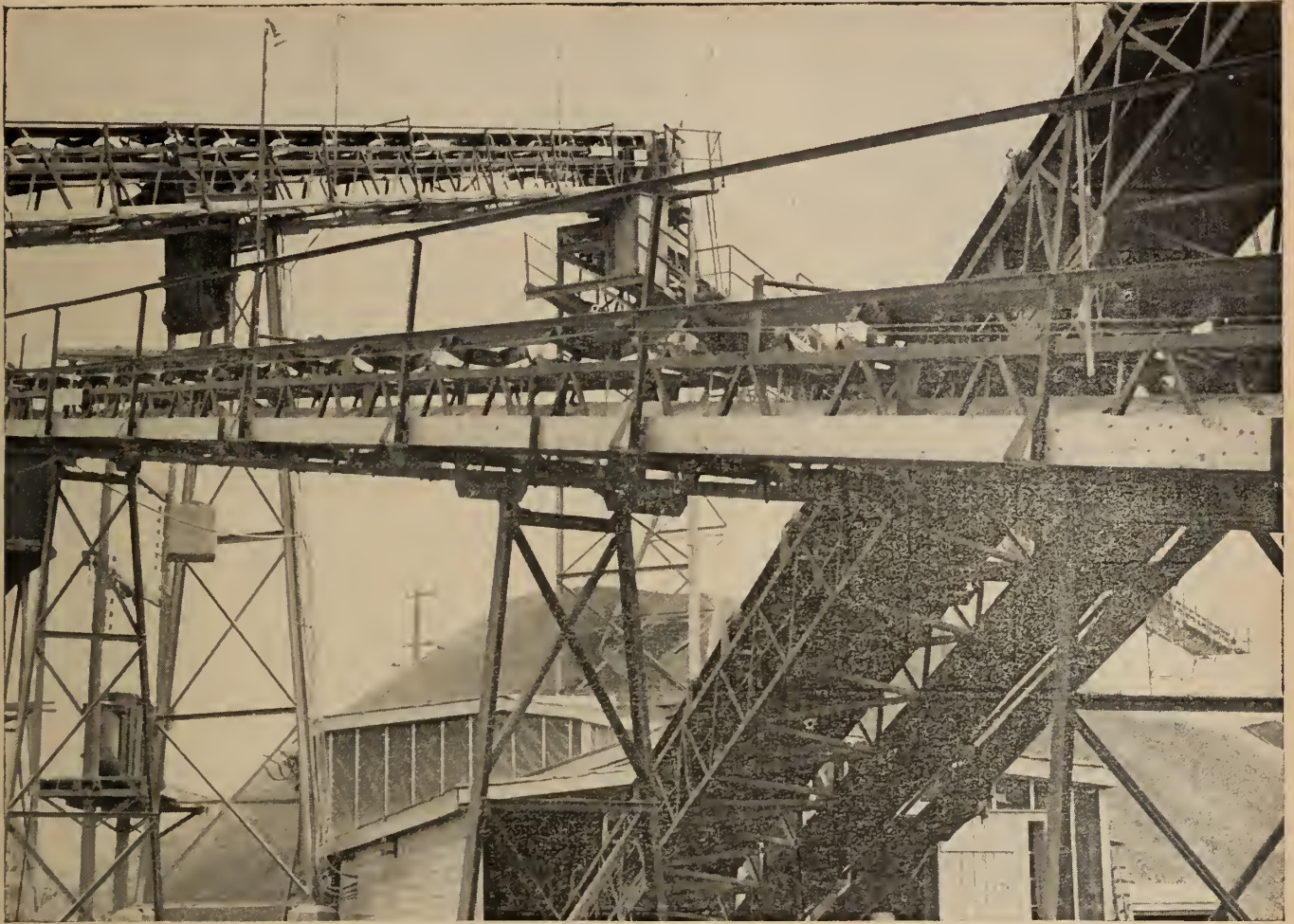
Four of the twenty-two Barber-Greene Conveyors at the Cornwall operation of the St. Lawrence Seaway.
