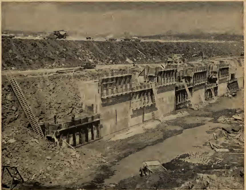
The approach walls of the St. Lambert lock. Great steel and wood forms are used to contain the concrete for each lift until it hardens, and then the forms are raised to the height of the next lift.
