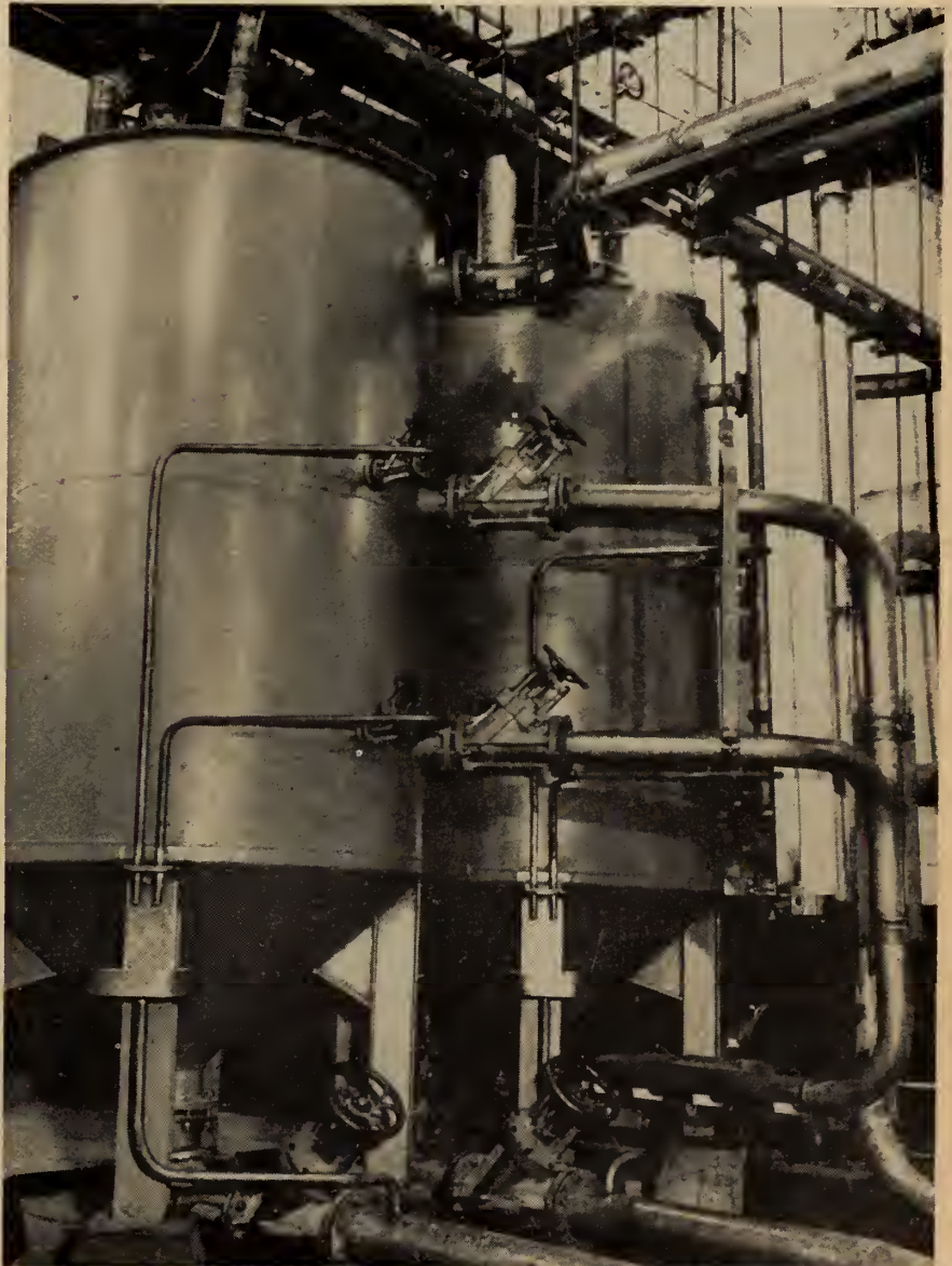
Fig. 11. Two settling tanks in one of the spin acid preparation departments. Sediment is drawn off from the conical bottoms; clear acid through the side connections. Steel plate tanks are lined with sheet lead burned in place after installation. Lead pipes at ceiling are supported on wooden blocks in steel channels.
