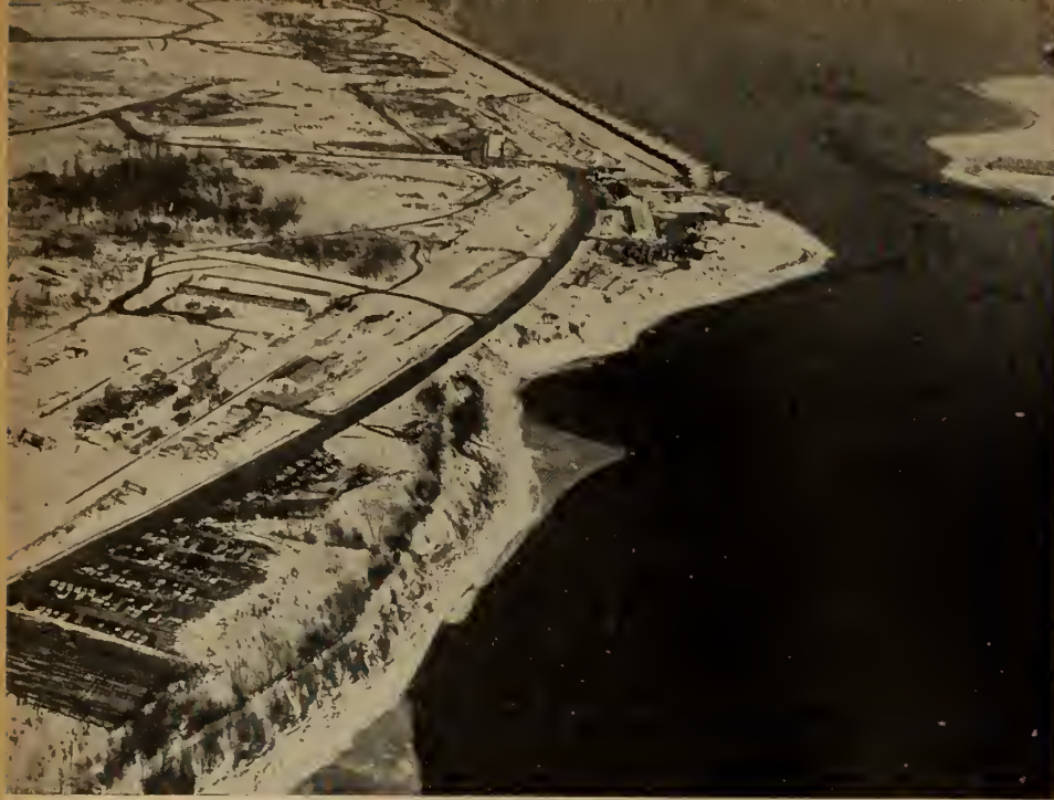
St. Lawrence power-house, Barnhart Island. Looking downstream at construction plant and power-house excavation, from U.S. side.
