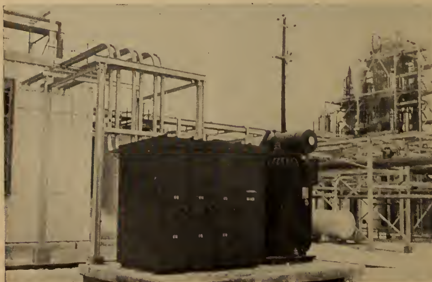
Fig. 13. Out-door unit sub-station, 13 kv./600 volt, 1500 kva.
