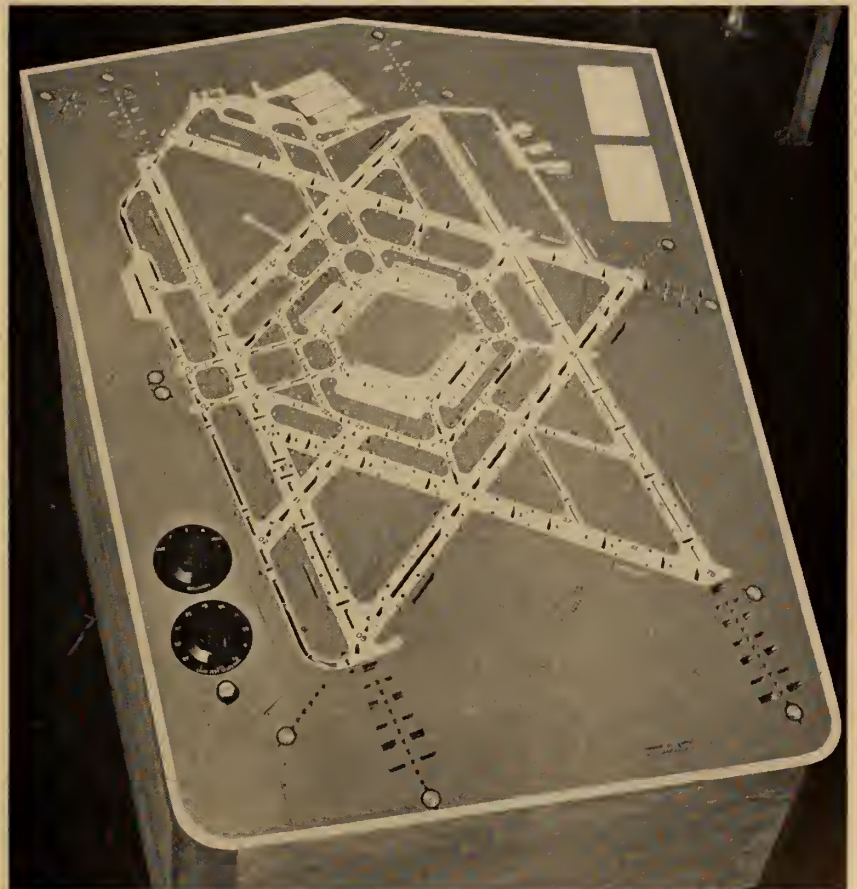
A mimic diagram of airfield lighting is used in the control tower.
