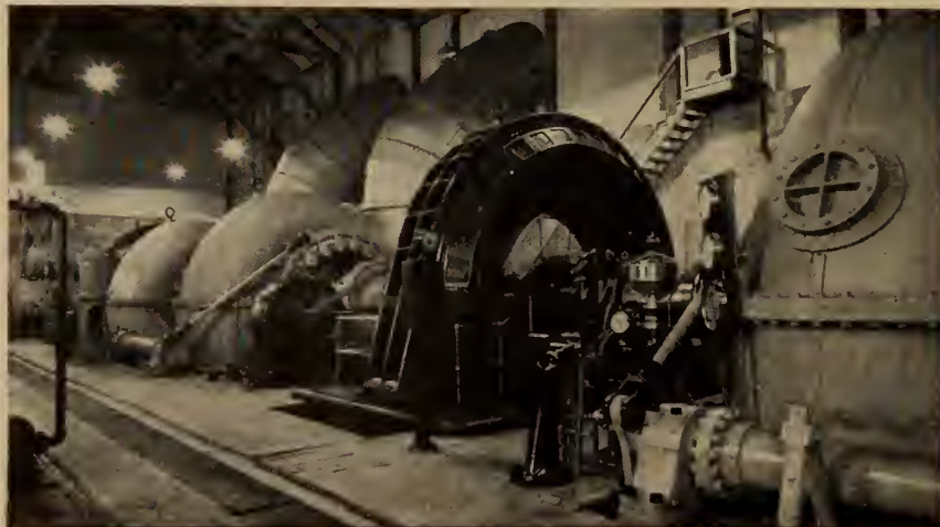
Fig. 16. Interior view of temporary power house.
