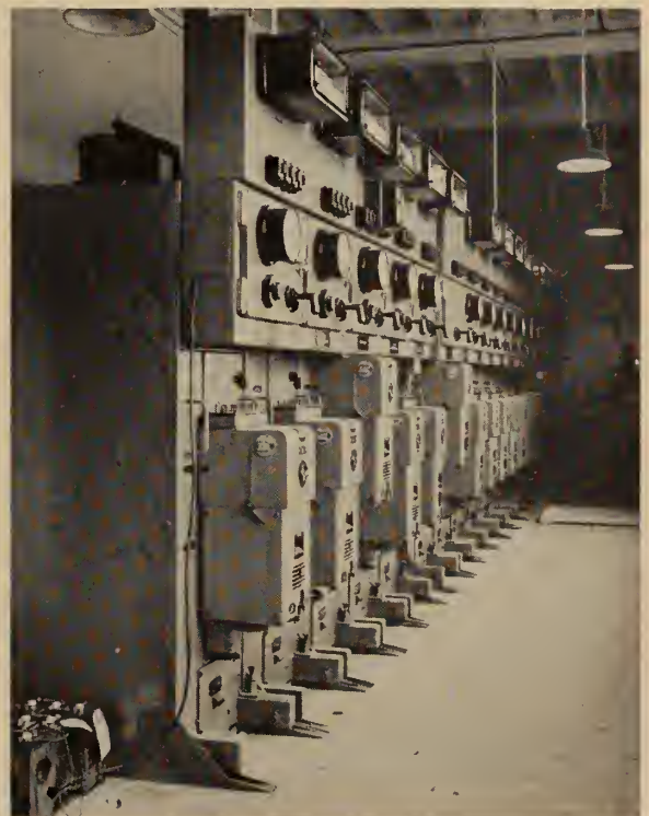
An 11-kv. switch-board in the central area control building, sub-station 23.
