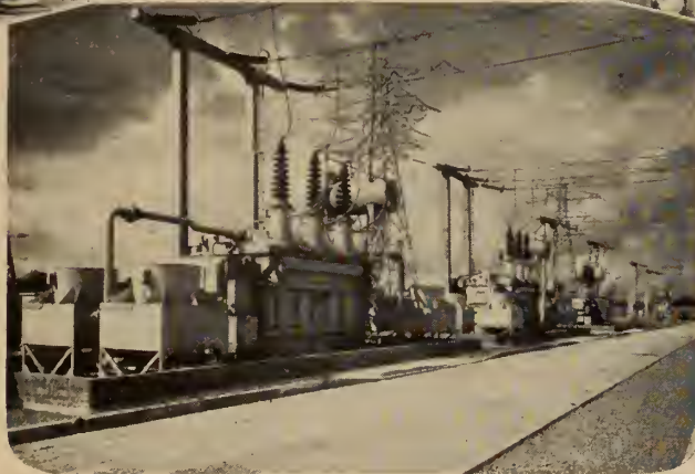
Two 36 M.V.A. generator transformers and two 5,000 K.V.A. station transformers.
