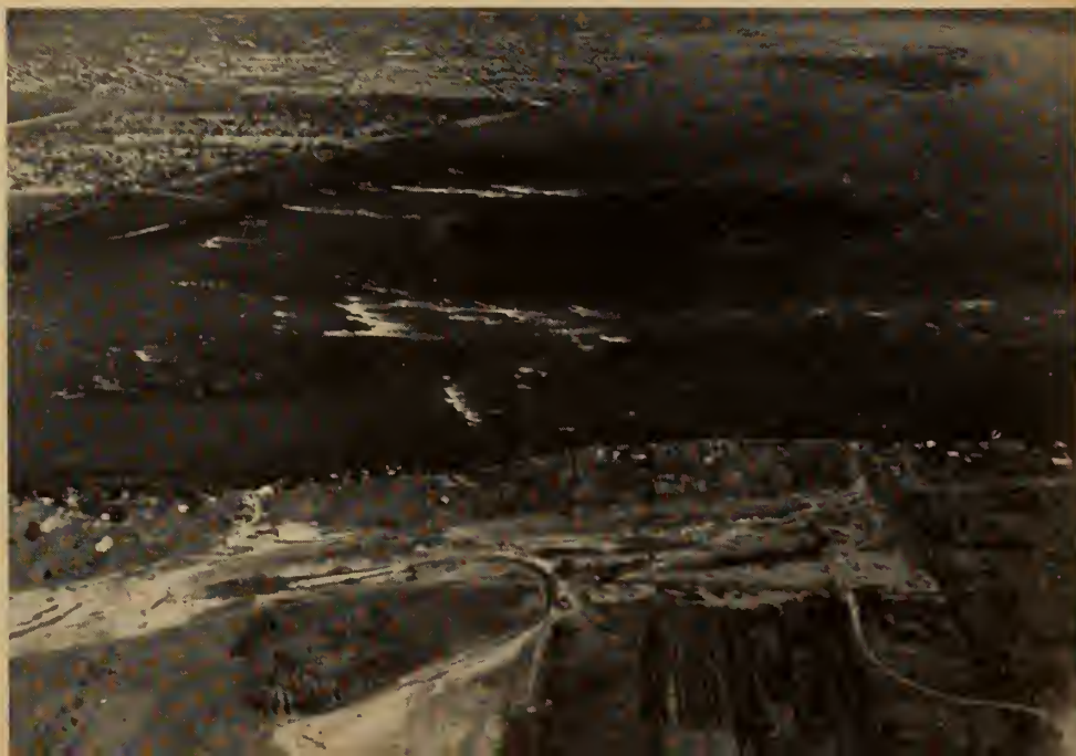
Air view of excavation on overland navigation channel near Cote St. Catherine. Heron Island at Lachine Rapids, in background, is probable location for upstream of two future power developments by Hydro-Quebec.
