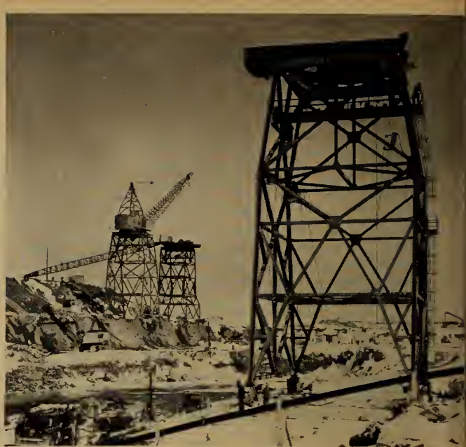
At the Barnhart power plant, one gantry crane assists in construction of the second.
