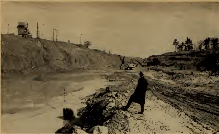
At the 80-ft deep excavation for the Iroquois lock at Iroquois Point, Ontario, the contractor will soon be placing concrete for the structure. Here ships will pass between the power pool or seaway lake and the upper river to enter the Thousand Islands section of the seaway.
