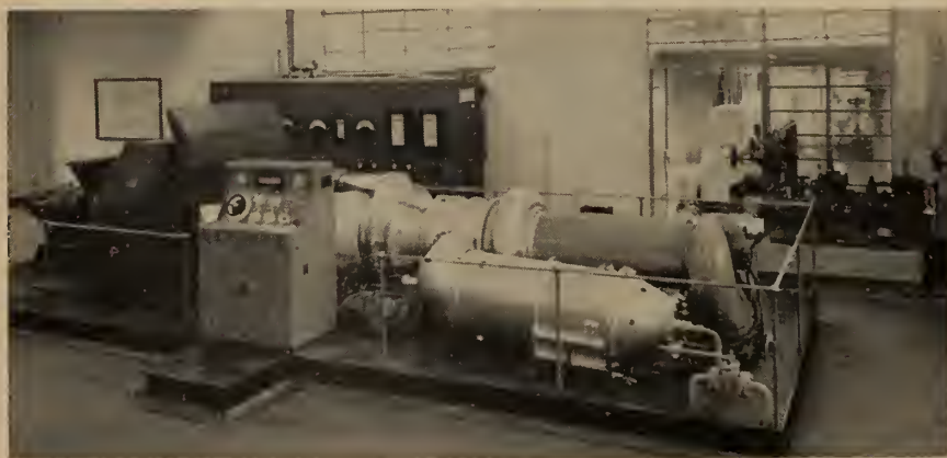
This industrial gas turbine installation at Cortemaggiore, N. Italy, operates on natural gas. The set has run for over 6000 hours; continuously for 3500 hours.
