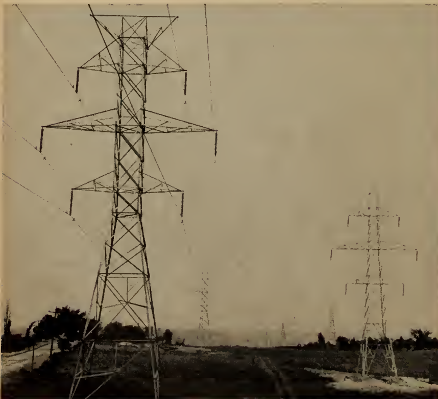
Fig. 5. Three examples of double circuit lines. Left to right: 230 kv., two overhead ground wires; 230 kv., single overhead ground wire; 115 kv., single overhead ground wire. (right background) (Hydro-Electric Power Commission of Ontario)
