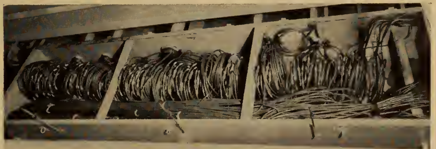
Fig. 6. One of the largest distributing boxes at Maitland.
