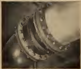
Garlock Rubber Expansion Joint on vacuum line between turbine and condenser
