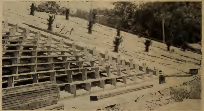
This concrete slab, for the grandstand at Portage la Prairie, Manitoba, was pre-cast and raised according to the patented Youtz-Slick system of lifting slabs. Structural design was done by Cowin and Company Limited, structural engineers; the lifting contractor was F. R. Lount and Sons; the general contractor was James F. Hamilton.
