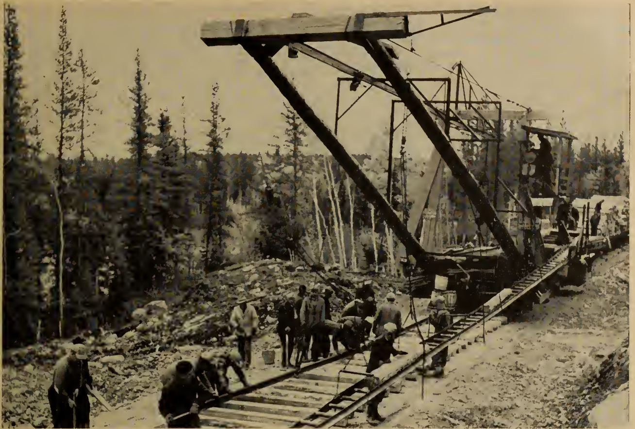
Fig. 3. Front view of "Pioneer" showing ties rolling forward and rail being lowered into position.
