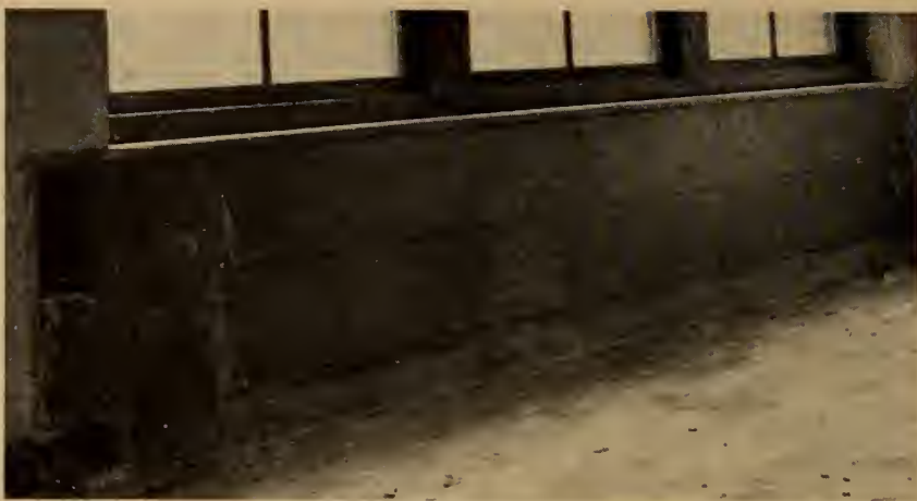
Fig. 2. Typical installation of radiant panels under windows in Dominion Textile Building.
