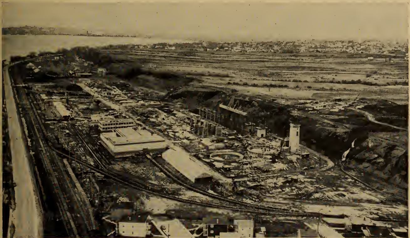
This picture of the St. Lawrence Cement Plant was taken on May 7, 1954. It shows:— at extreme right—crushing plant foundations; right centre—construction of smoke stack; centre—foundations of slurry basins and erection of steel shell, columns for crane rail beam of storage hall, scaffolding ready for the whole length, slurry mill bin walls poured, temporary storage shed, and workshop and offices already occupied; extreme left—foundations and platform of packing station completed, column form work started. Railway siding ready to receive trains with material in the yard.
