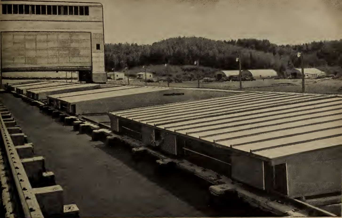
The practical design of the new Chute-a-la-Savane powerhouse is photographically illustrated above. Hatch covers of crimped, batten-seamed aluminum, form the roof over the G-E Generators. The aluminum housed, rail-mounted 250-ton gantry crane, can be spotted over each generator for servicing. The covers roll back and aluminum sides can be lowered on the crane to make a weather-proof work area above each unit. If rotors must be removed for repair or inspection, they can be moved to a large repair bay at one end of the powerhouse.
