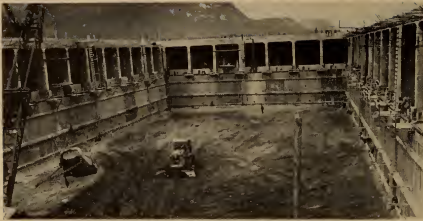
Fig. 81. Caissons ready for launching, bulkheads, ladders, lighting plants, etc., all in place.
