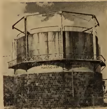
Left: 40,000 cu. ft. Horton gasholder 50 ft. in diam. and 50 ft. high.
