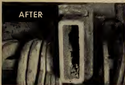
This job was accomplished in 8 hrs. while previous lancing methods required up to 30 hours.
