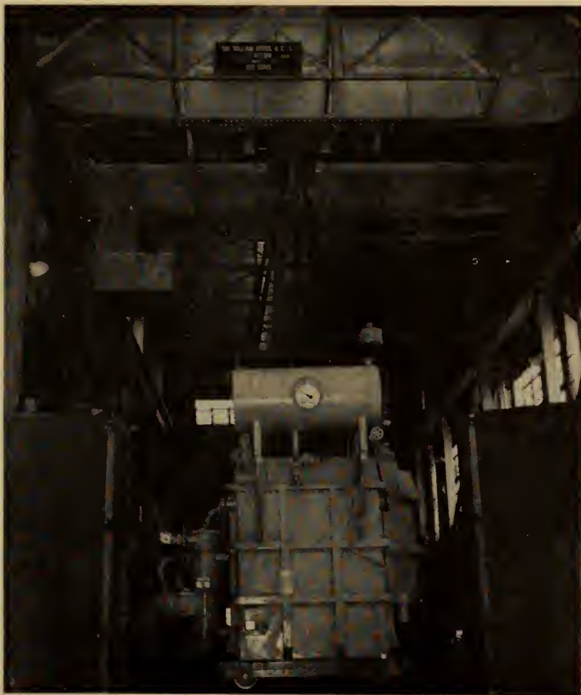
Fig. 117. 100-ton transformer crane in electrical repair shop. Showing transformer about to be lowered into pit.
