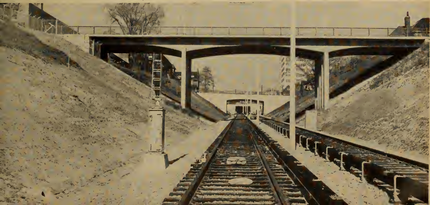
Fig. 5. Typical open cut section showing the location of the contact rail and automatic block signal.
