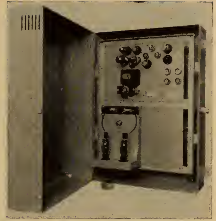
Fig. 5. Electronic grinder load regulating panel; electronic watt meter at upper right.
