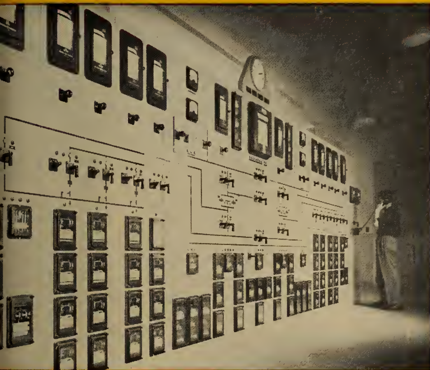
MODERN SUBSTATION SWITCHBOARD, Hydro-Quebec.
