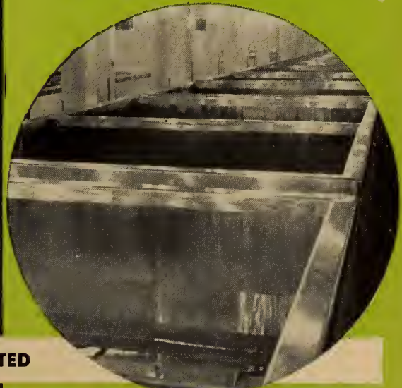
Twenty-two tanks of Type 304 clad stainless steel installed in the up-to-date fermenting room at Vancouver Breweries Limited, Vancouver, B.C. The tanks were fabricated by Ellett Copper & Brass Co., Ltd., Vancouver, B.C.
