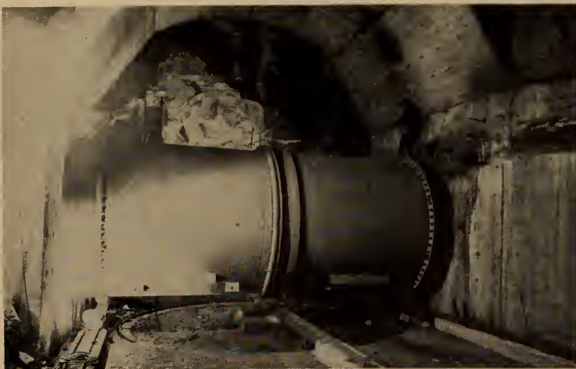
Fig. 47. Removable section at head of penstock.
