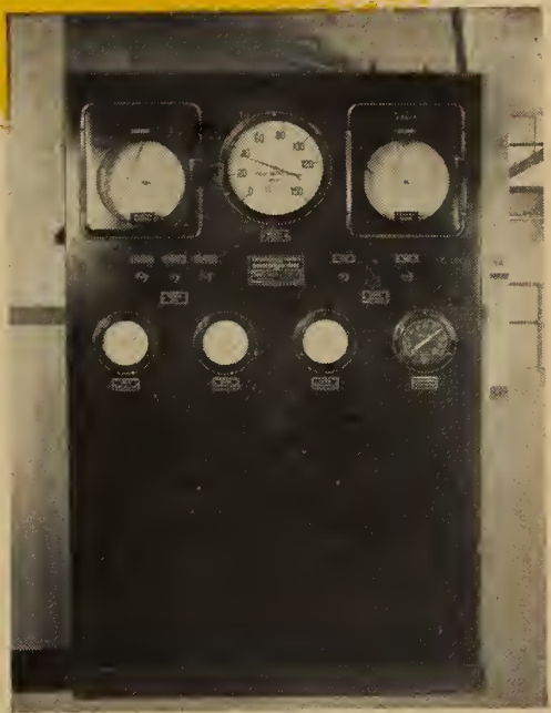
Municipal waterworks pumping station control panel. System includes automatic level control of elevated water tank, water flow and pressure records and instruments to assist operator in continuously checking clear-well level and pump suction pressures.
