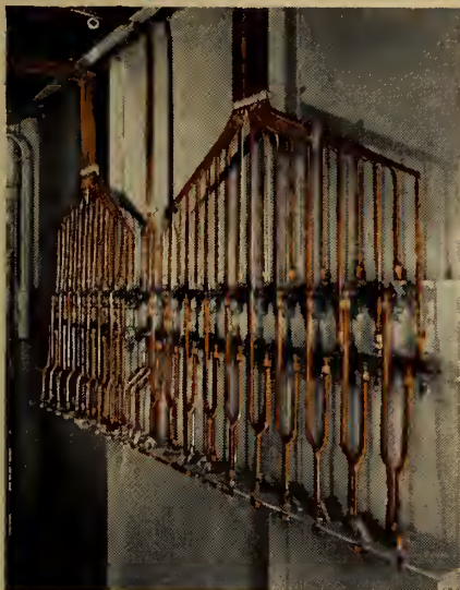
MOIST COMPRESSOR AIR can never form rust or scale to impede control in this installation made by Bailey Meter Co., Ltd.
