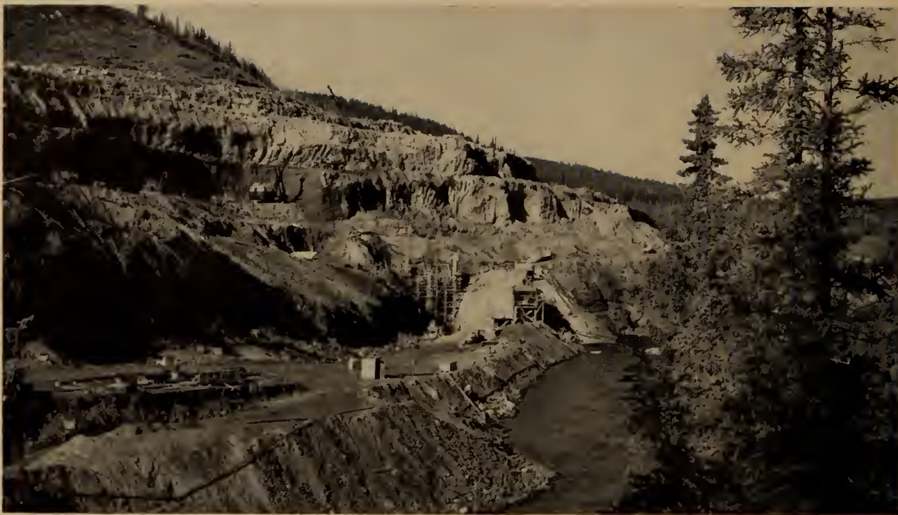
Fig. 4. Nechako River before diversion. Stripping in progress and forms for tunnel gate structure in place.
