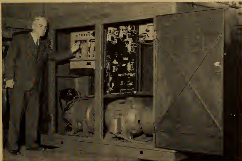
Fig. 4. 40 hp. electronic speed control power unit; motor generator set at bottom; magnetic control at upper right; electronic control at upper left.
