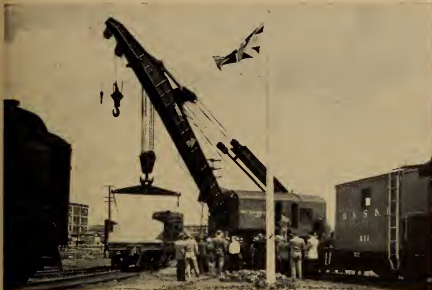
Q.N.S. & L. Crane No. 1200 on test
