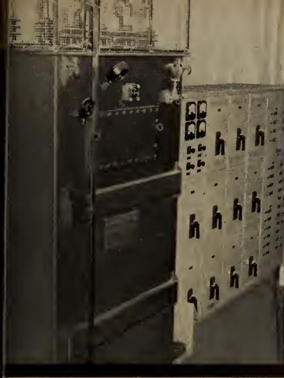
The transformer in the foreground—one of four on the "Hydro-Quebec"—delivers current at 600 volts to the 7-voltage distribution panel (background) which relays power to points all over the dredge.
