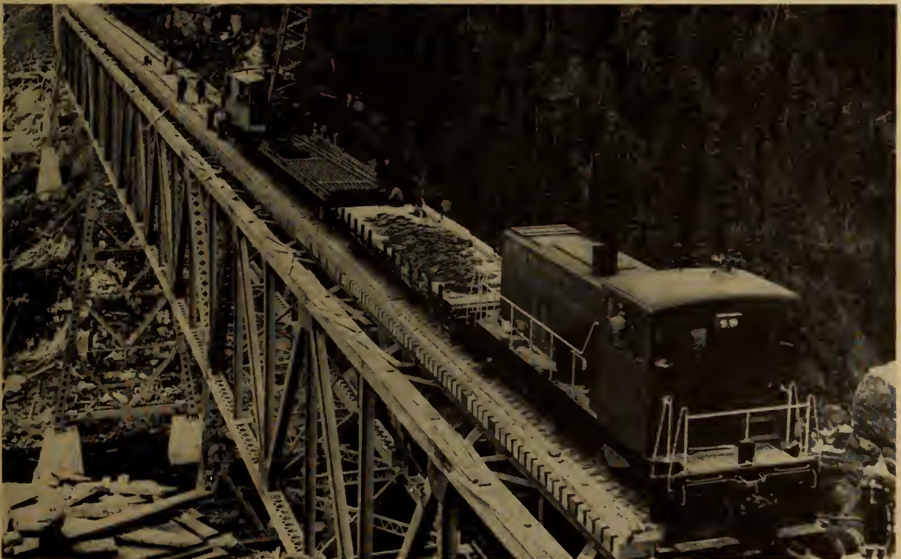
Laying tracks on the bridge at Mile 12. The largest between Moisie River and Knob Lake.
