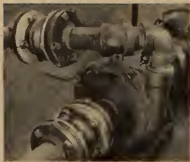
Expansion joints in operation on 2 1/2" suction and discharge pipes
