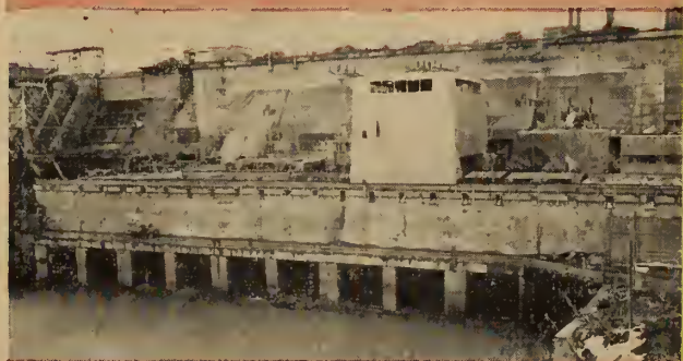
Peribonka No. 2 Powerhouse—located at Chute o la Savane, Quebec. Owner and Engineers same as No. 1 Project. Contr.: Pentagon Construction Co., Ltd., Montreal.
