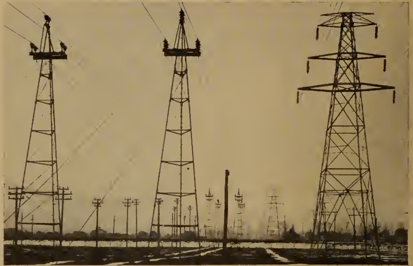
Fig. 6. 60,000-volt line of O.P. Co. and 110,000-volt H.E.P.C.
