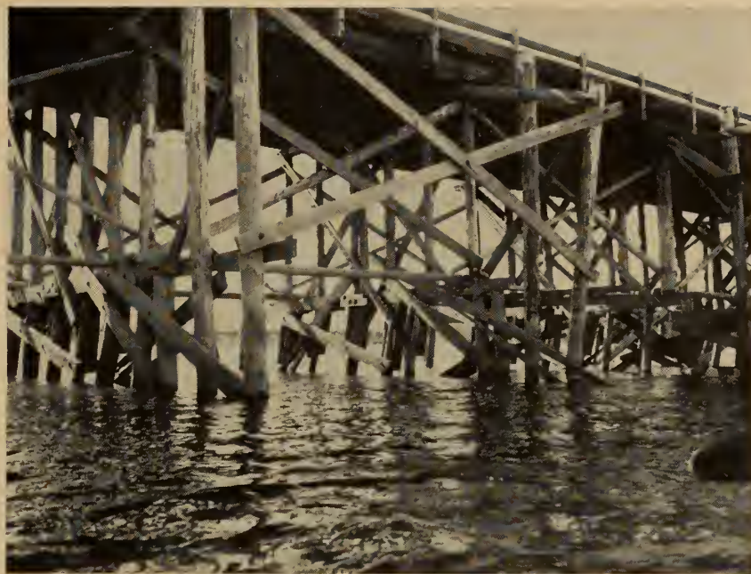
Fig. 6. Nisutlin Bay trestle, Mile 804; ice damage each spring requires continual maintenance.
