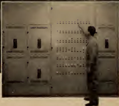
View of motor control panelboard located in sub-basement. Motors on all floors can be controlled from this location.
