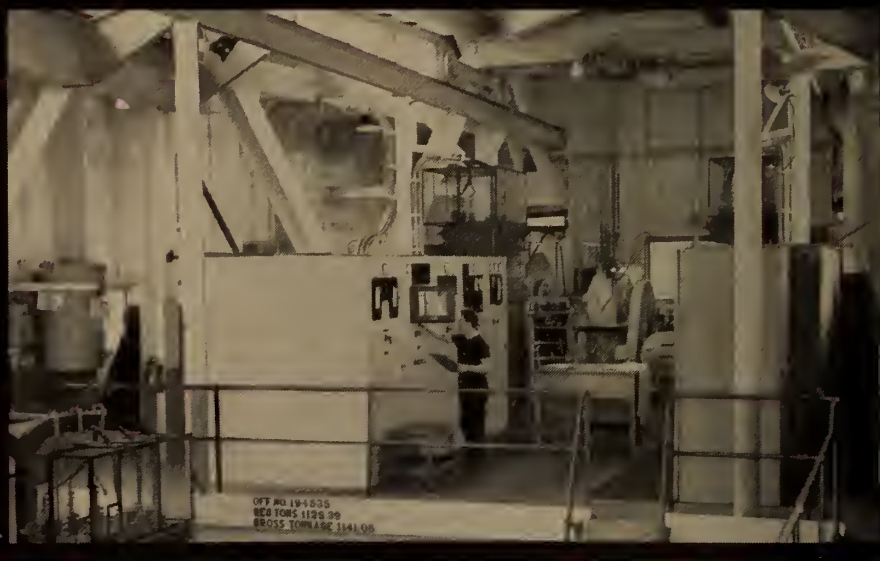
The dredge's switchgear—15-kv vertical-lift drowout metal-clad type—is built for all-weather duty. It consists of a 1200-hp synchronous motor starter, an 8000-hp motor starter, a 600-kw transformer feeder, a 600-hp synchronous motor starter, a combination bus entrance and auxiliary compartment, and a set of metal-clad accessories.
