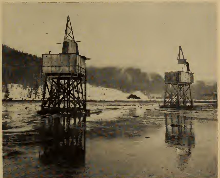
Fig. 76. Platforms for soil borings, on stilts to take care of 22 ft. tides.
