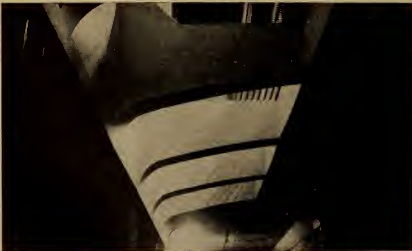
Fig. 6. Looking up into the vent shaft at the north end of St. Clair Station platform.
