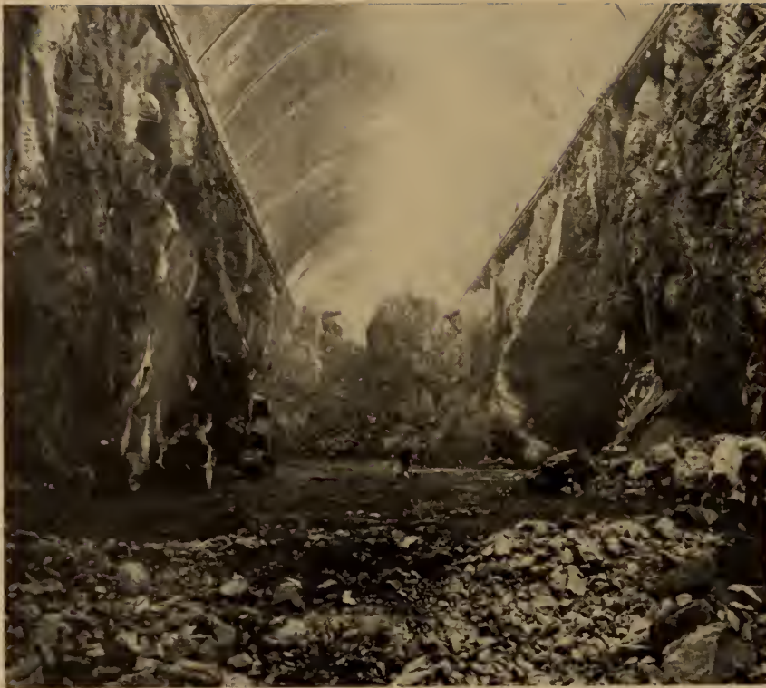
Fig. 30. Working out from the center the main body of the power chamber excavation was blasted by shooting off slabs 80 ft. high.
