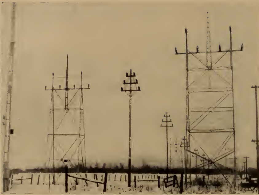
Fig. 1. T.N.P. power lines — 60,000, 44,000 and 99,000-volt lines.
