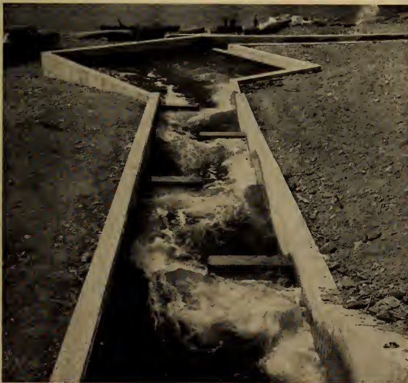
Fig. 5. Tobique Fishway. Looking downstream to first resting pool.
