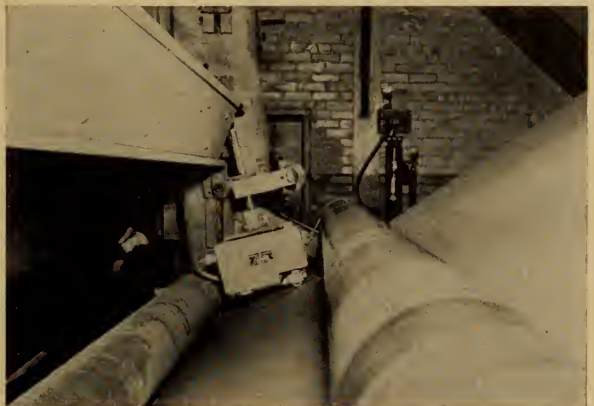
Fig. 12. Tensiometer installed between two calender sections and mounted on screw to adjust for different pass line to second calender.
