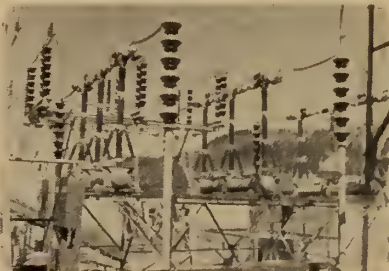
High Voltage Stations
