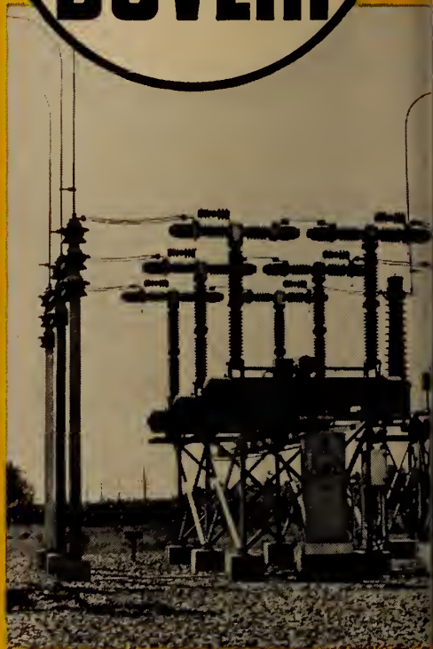
HIGH VOLTAGE AIR BLAST CIRCUIT BREAKERS, Saguenay Power Co. Ltd., Isle Maligne., Quebec.
