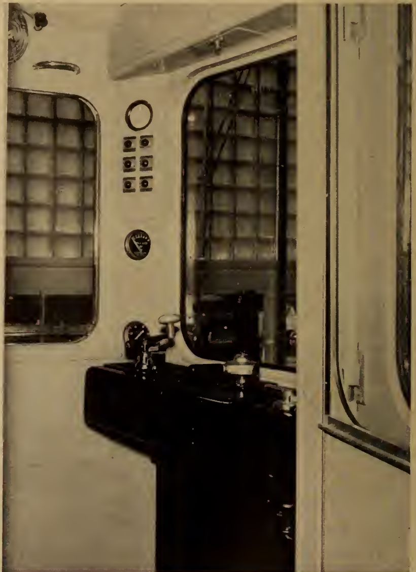
Fig. 2. A subway driver's cab showing the main controls and the indicating light panel.
