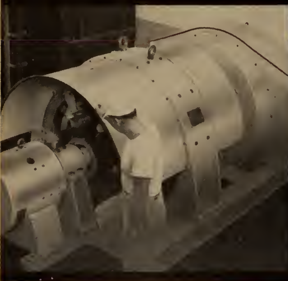
G-E three-unit mg set provides current for the adjustable-voltage cutter drive. This unit is made up of a 1200-hp 900-rpm synchronous motor, an 800-kw 600-volt generator and a 20-kw 125-volt d-c exciter.
