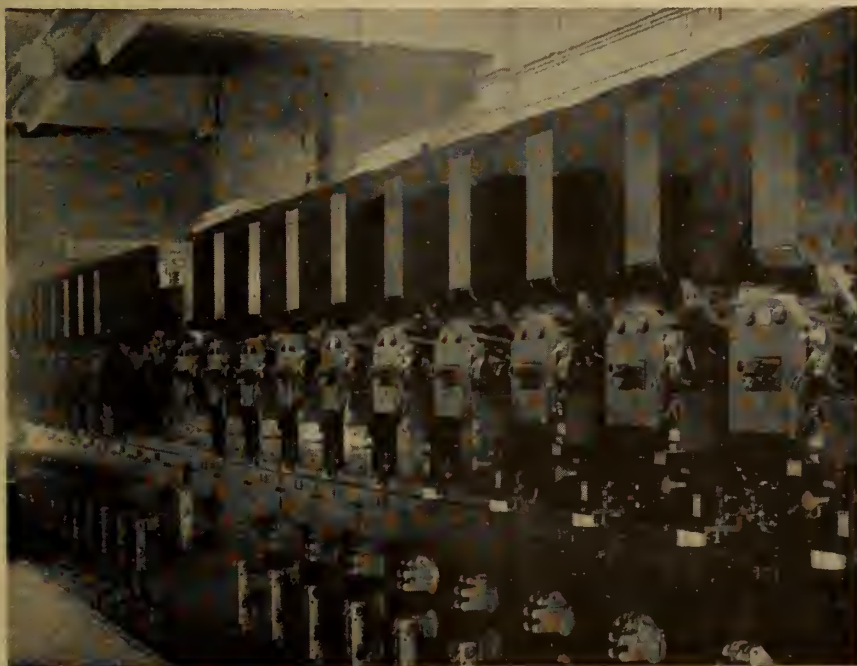
Fig. 3. A 600-volt d-c. breaker board in a typical automatic rectifier substation.
