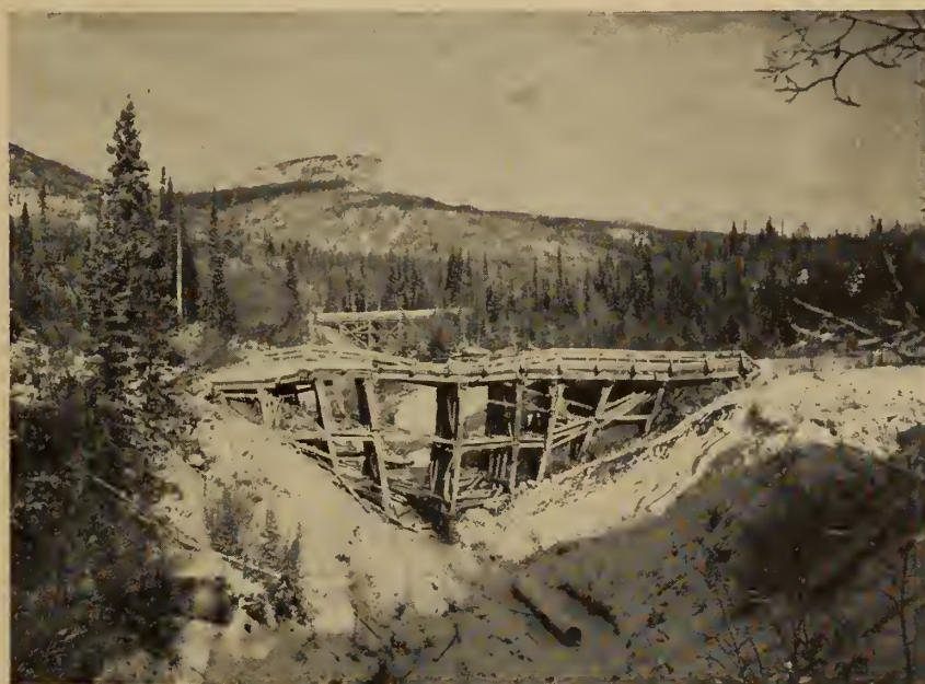
Fig. 4 Gardiner Creek Bridge, Mile 358, illustrates the extent of soil movement.
