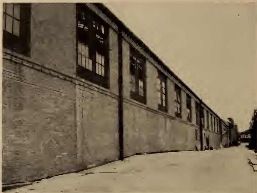
Fig. 4. Distortion of long factory building on fill.
