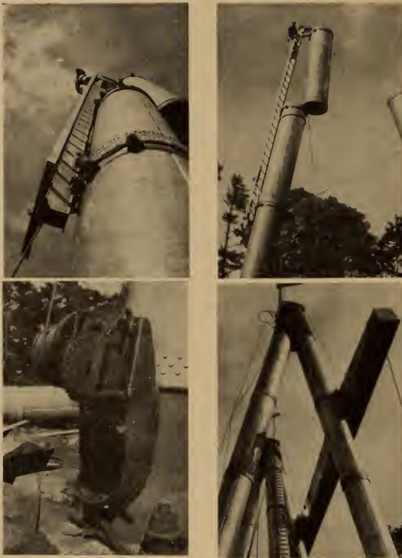
Fig. 71. Erection methods; upper views show "climbing ginpole". Lower left shows 5-ton hand winch; lower right shows cross-arm pulled up.
