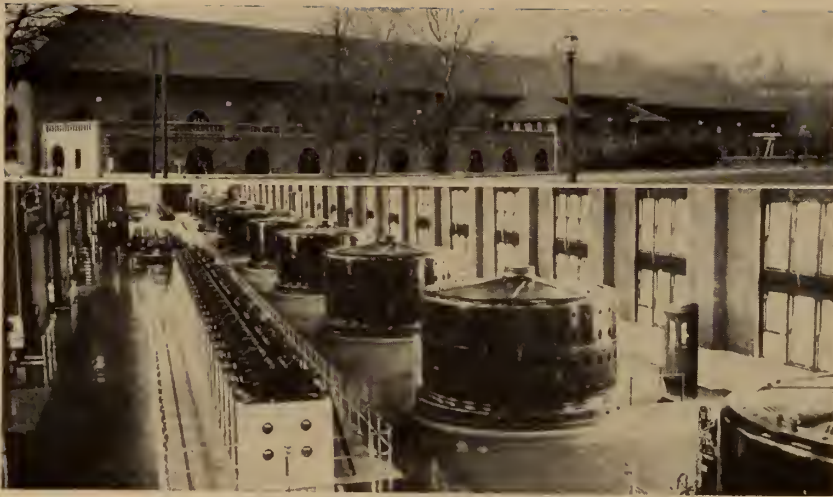
Above: Exterior view of Canadian Niagara Power Company, a private power company located on the upper Niagara River.
