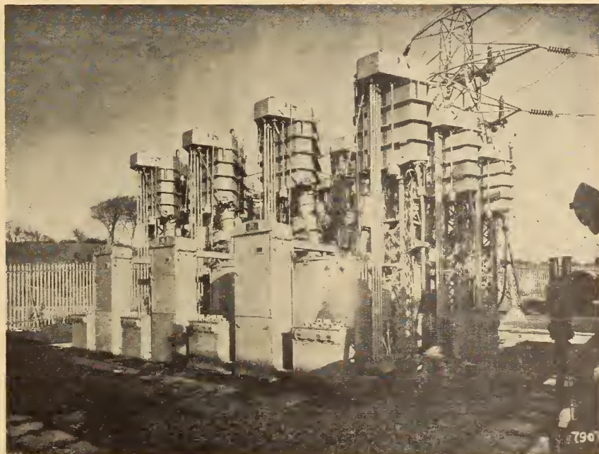
Fig. 5. Tongland substation. Reyrolle 132-kv. switchgear.
