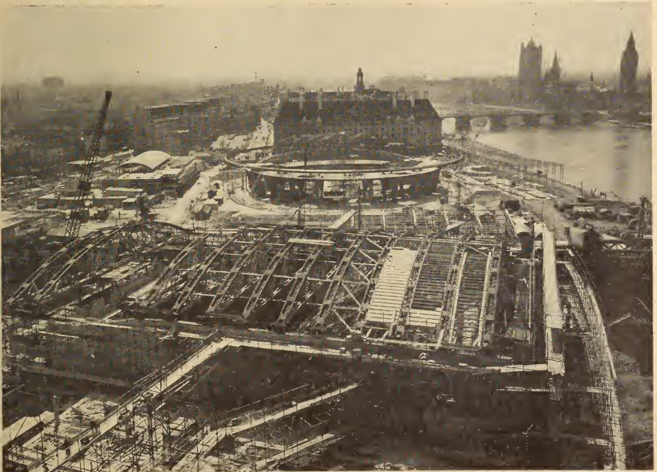
Fig. 3. Construction of the Royal Festival Hall showing erection of roof girders nearing completion.
