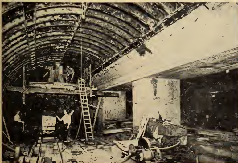
Fig. 16 (right). London underground railway. Increased length of station showing running tunnel ironwork still in place. Note small clearance around rolling stock
