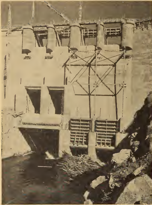
Fig. 7. Upstream face of the dam showing by-pass openings. Water is passing through 50-ft. channel (lower left) and two 21-ft. channels, closure gates for which are seen mounted above the openings. Above the 50-ft. opening can be seen the two additional 21-ft. channels for limiting the head on the lower gates.
