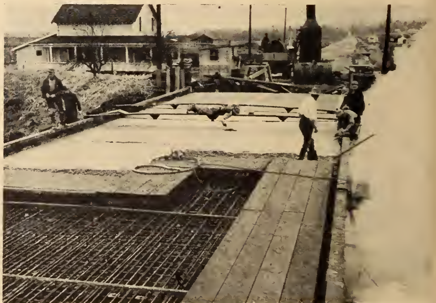
The composite timber-concrete bridge provides the answer for public works departments faced with bridge replacements as labour and material becomes increasingly scarce and costly.
