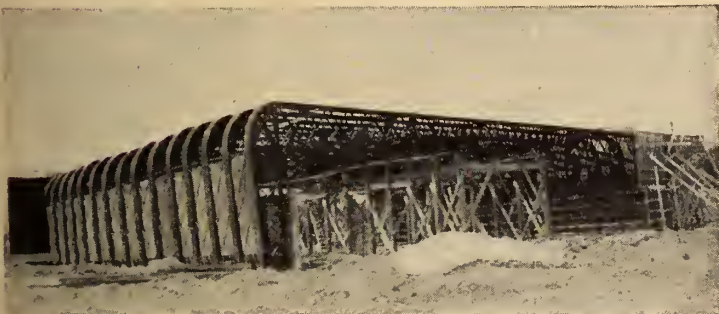
Steel structure for overpass at intersection of Toronto-Barrie dual highway and Toronto by-pass
