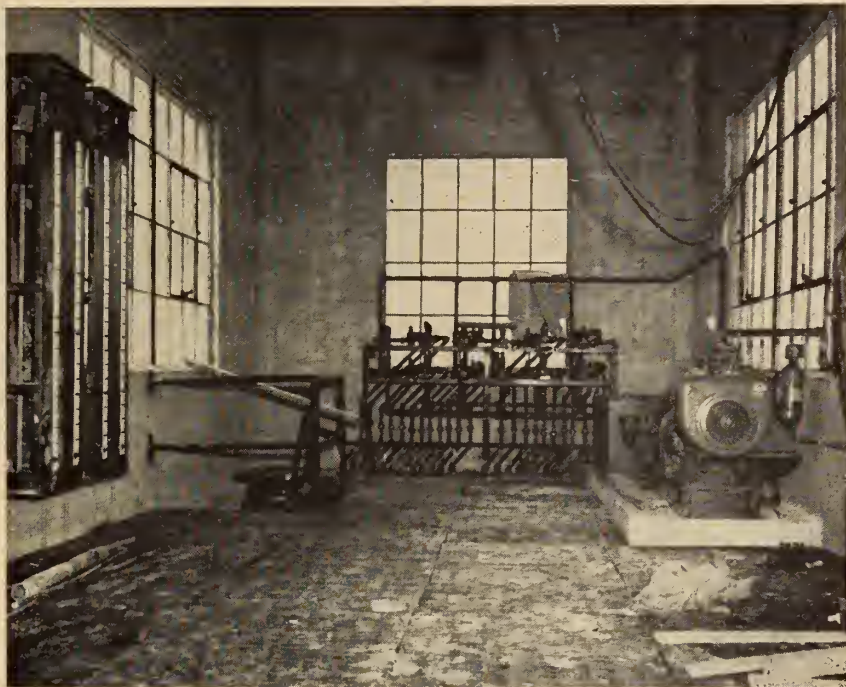
Fig. 4. Control house of irrigation tunnel, showing controls for outlet gates. Gates 90 ft. below floor of control house.
