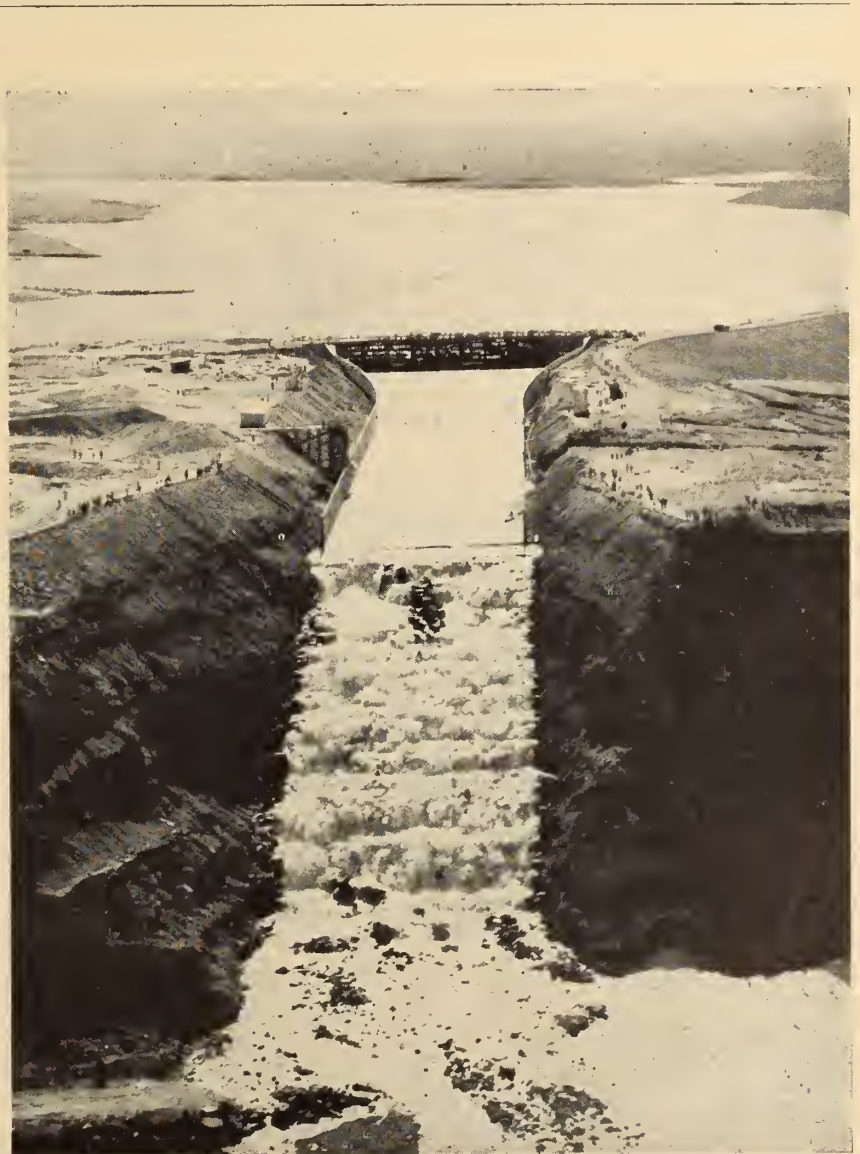
Fig. 2. St. Mary spillway with water dropping 150 ft. on uncompleted chute section. Chute section will be paved when completed.
