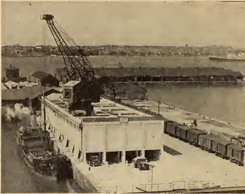
Fig. 4. Storage and transit bunker, erected at Liverpool Docks for ship-to-truck movement of granite. All the wall panels and the supporting piers were precast.
