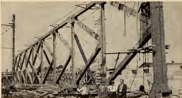
80 ton truss 220 feet by 28 feet ready for raising on 68 ft. columns on new Kitchener Auditorium.
