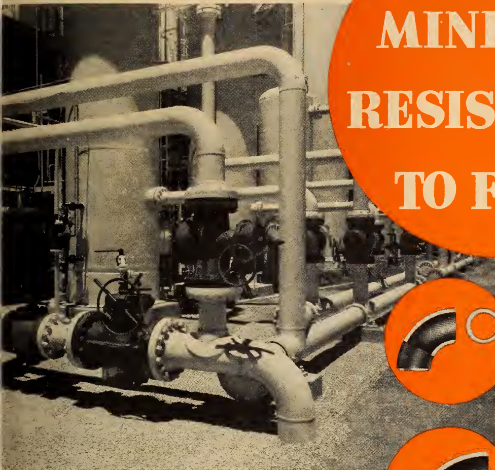
Grinnell Welding Fittings on towers of natural gasoline plant.
