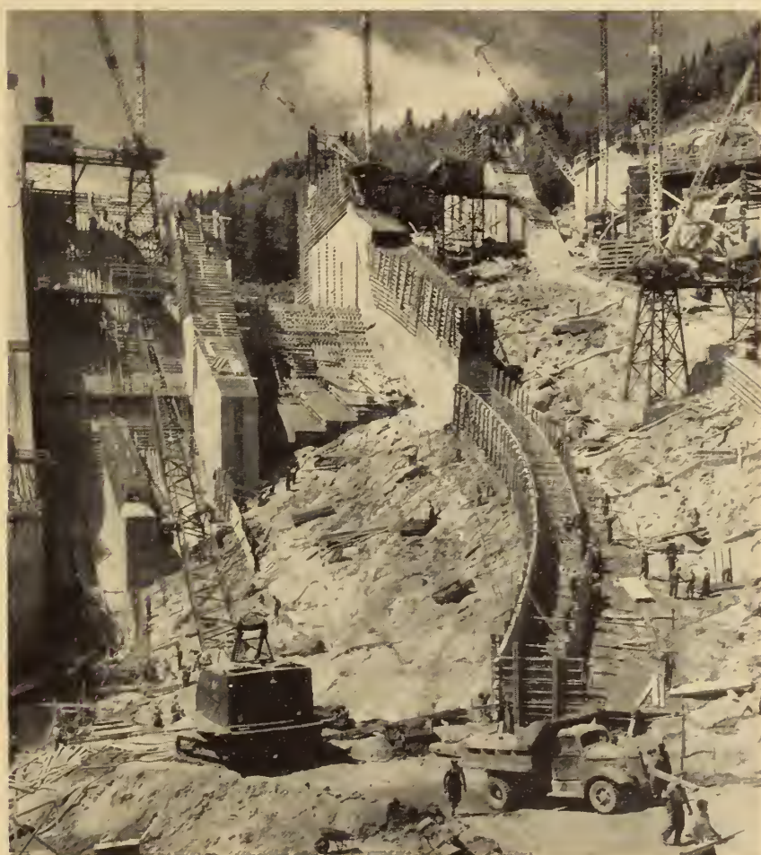
Fig. 6. Sluiceway and flood channel under construction. The maximum discharge will be 170,000 cubic feet a second, including the projected five turbines, four regulating gates and the four sluice gates, each of which is 50 feet by 31 ft. 6 in. The sluice section is 260 feet long, and the flood channel extends 450 feet downstream from the sluice.
