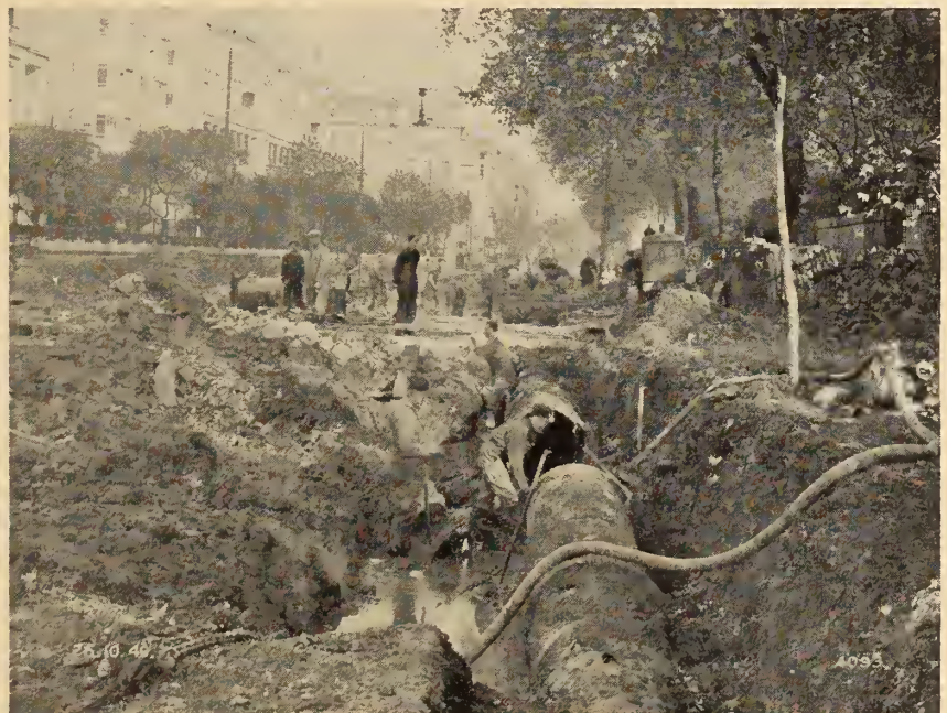
Fig. 7. Broken water mains and sewers on Bayswater Road, London.
