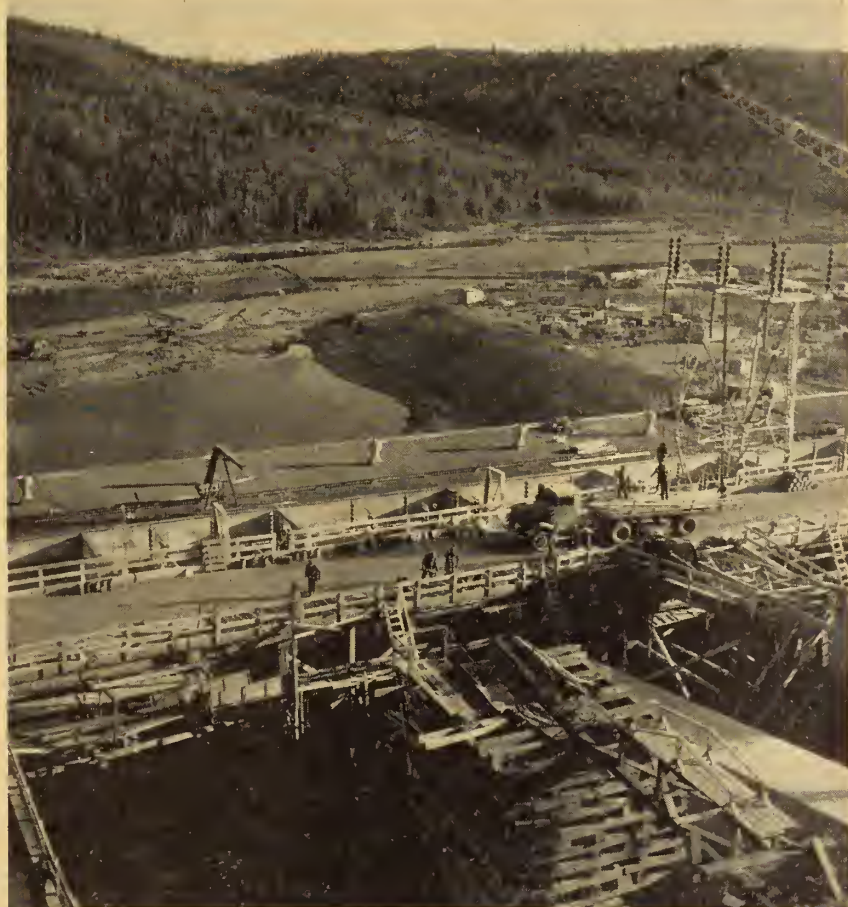
Fig. 3. The top of the intake section of the Trenché dam. The tailrace in the background, drained almost dry while the headwater level was being raised, is some 235 feet below the crest of the dam.
