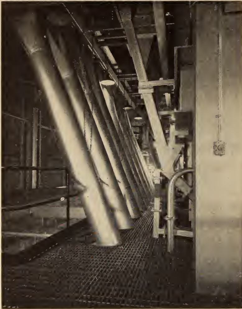
Fig. 6. Front of boilers showing coal and bark chutes.
