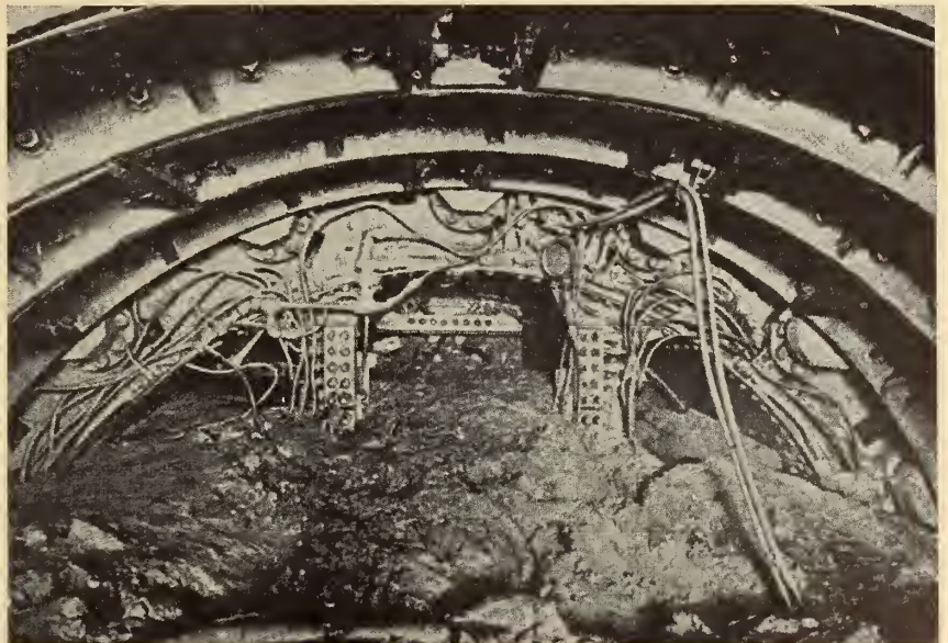
Fig. 12. Tunnel shield after serious blow.
