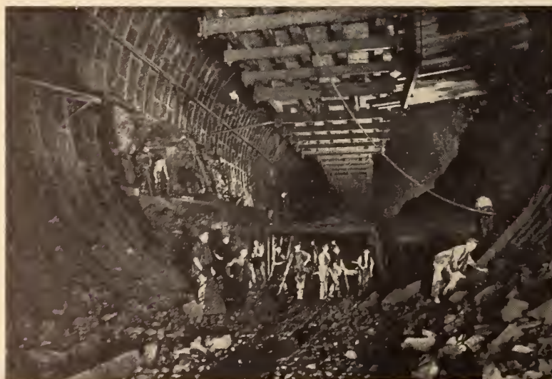
Fig. 5 (right). Complicated cast iron segment work in ventilating shaft of vehicular tunnel.
