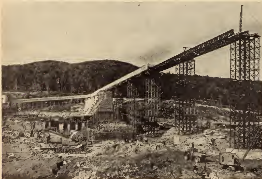
Fig. 14. La Cave Development — View showing application of Bailey bridging for concrete conveyor trestle. Powerhouse draft tube forms are at left centre.
