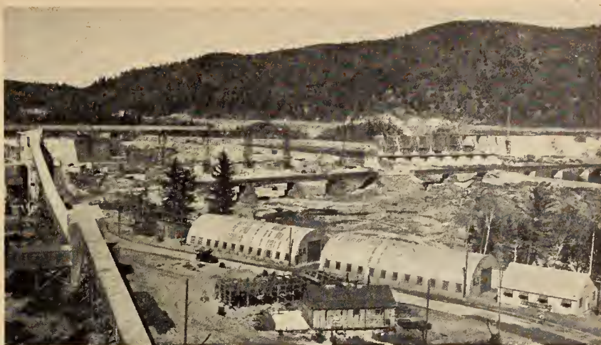
Fig. 15. La Cave Development — General view showing concrete conveyor system. Bailey access bridges and partially completed dam looking from right bank of river.
