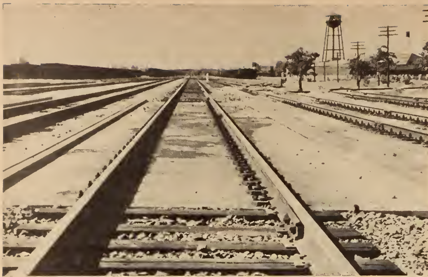
Fig. 5. The track design for the Subway was developed from the design shown in this illustration. It is a type that has been used by the C.N.R. on bridge decks.
