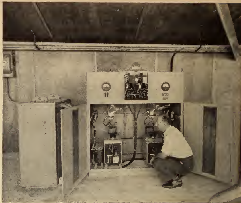
Fig. 4. D-c Rectifier assembly.
