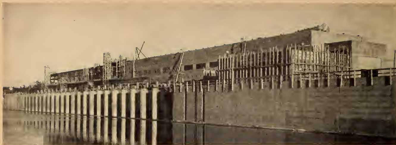
Fig. 11. Chenaux Development — View of headworks and powerhouse from the partially filled forebay.
