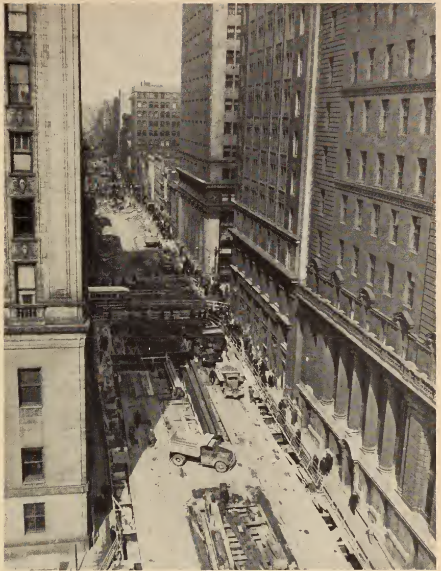
Fig. 2. Panoramic view of Yonge Street looking north from Melinda. In the foreground may be seen the complete decking in this area and proceeding through the photograph may be seen top lift excavation and the temporary suspension of utilities operating in the King intersection area with track and track-bed removed from the area between King and Adelaide Streets. In the background may be seen the pile driver in operation between Adelaide and Richmond Streets.
