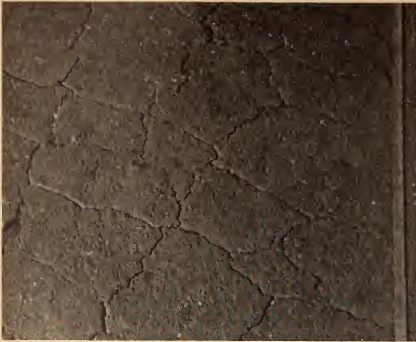
Fig. 1. Typical pattern of pavement cracks caused by deflection due to inadequate sub-grade support.
