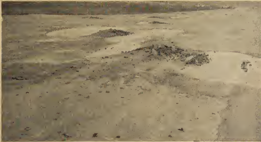
Figs. 3 and 4 (centre and bottom). Two views of damage caused by settlement of building foundations in the Kamloops area of British Columbia.
