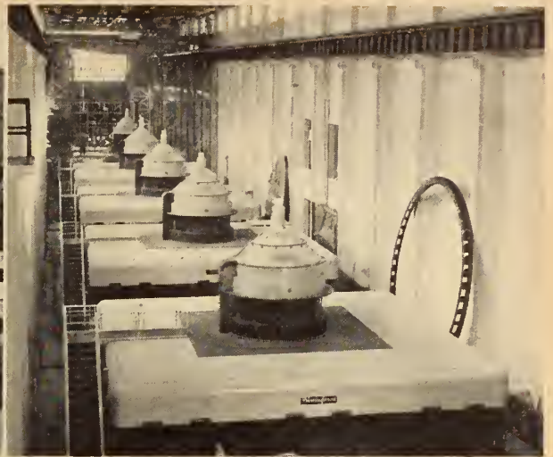
Fig. 4. Des Joachims Development — Interior view of powerhouse.
