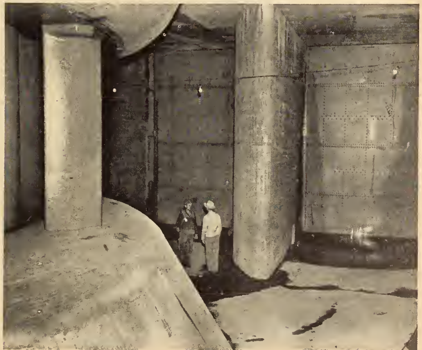
Fig. 10. Chenaux Development — Head gates viewed from within the scroll gate.
