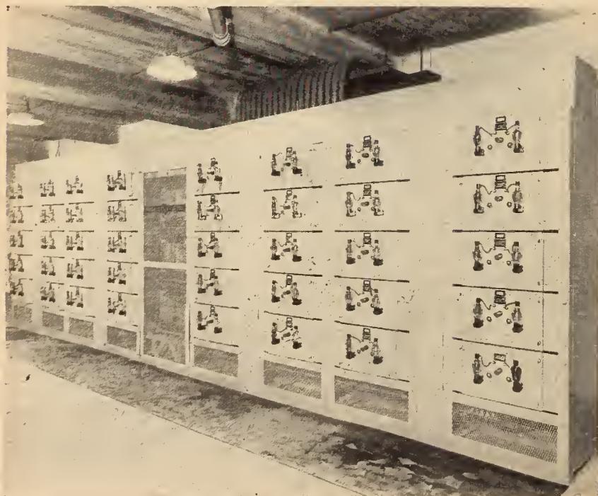
Fig. 5. Reactor frame — general view.
