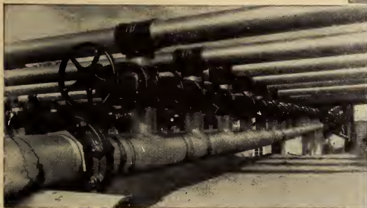
▲ CRANE VALVES and fittings on manifold in field gathering system.
