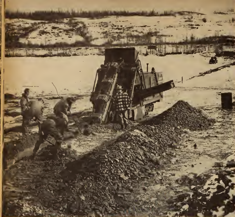
Fig. 5. Imperial-Leduc development. On this particular pipeline job, workmen are trenching through two feet of river ice and into the bed of the river in order to lay pipeline from the Leduc field gathering system into the new Woodbend area. It is something of a race against time as a quick thaw could leave them stranded on the river with a 14-ton digger and no means of getting it up the bank.
