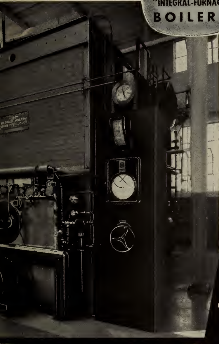
This Type G "Integral-Furnace" boiler at a cellulose plant, Weston, Ont., produces 9000 lbs of steam per hour at 125 lbs. pressure
