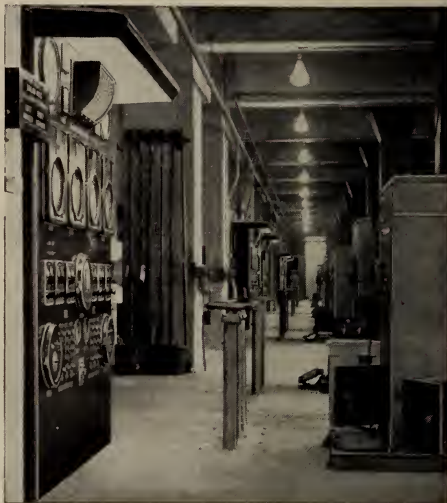
↓ (Below) View at Front of Boilers showing Boiler Metering and Control Panels.
