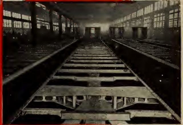
Underframe of all-welded steel car in position prior to assembly of side sheet assemblies.
