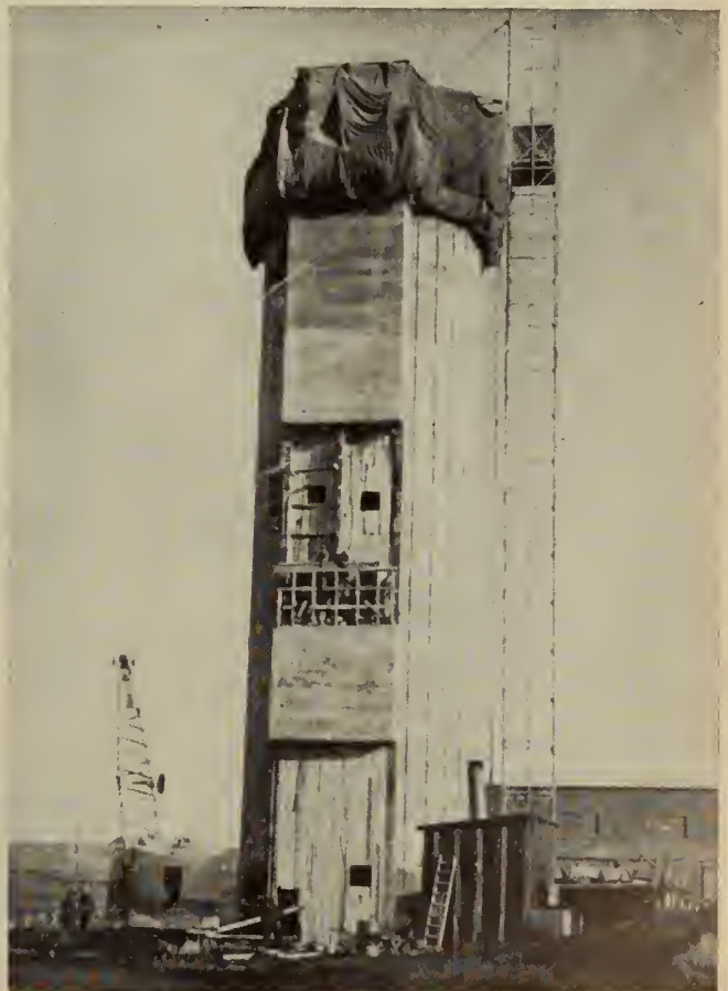
Fig. 6. Sliding forms approach the top of the tower as concreting operations reach the final stage.
