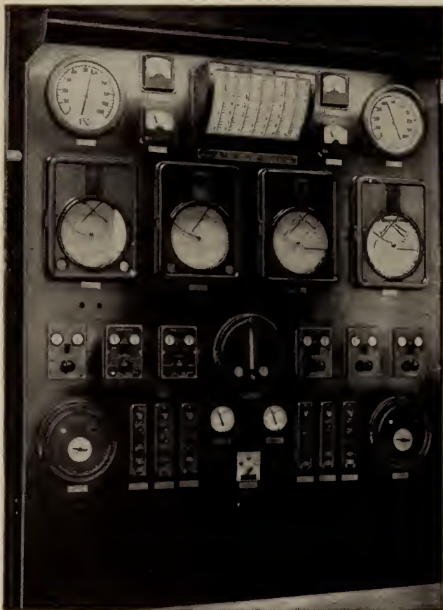
← (Left) Individual Boiler Panel showing Meters, Recorders, Controllers, Gauges, Selector Valves, Ammeters and Pushbutton Stations.
