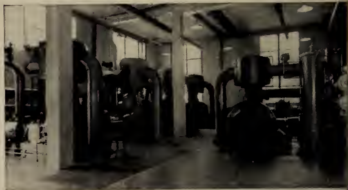
... installation of five "XVHE-2" Synchronous Motor-Driven units compressing air for the operation of forging hammers and many other purposes in the manufacture of high-speed alloy and stainless steels.
