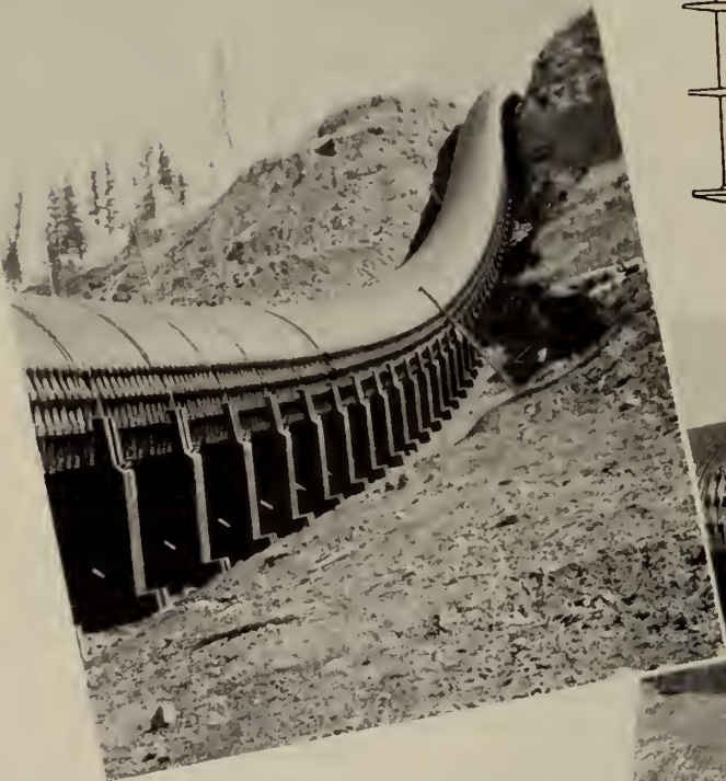
Two views of the ten-foot Creosoted Continuous Wood Stave Pipe, installed for the Calgary Power Company Limited at Banff, Alberta. Pacific Metal Butt Joints (Patented) were used for connecting stave-ends.
