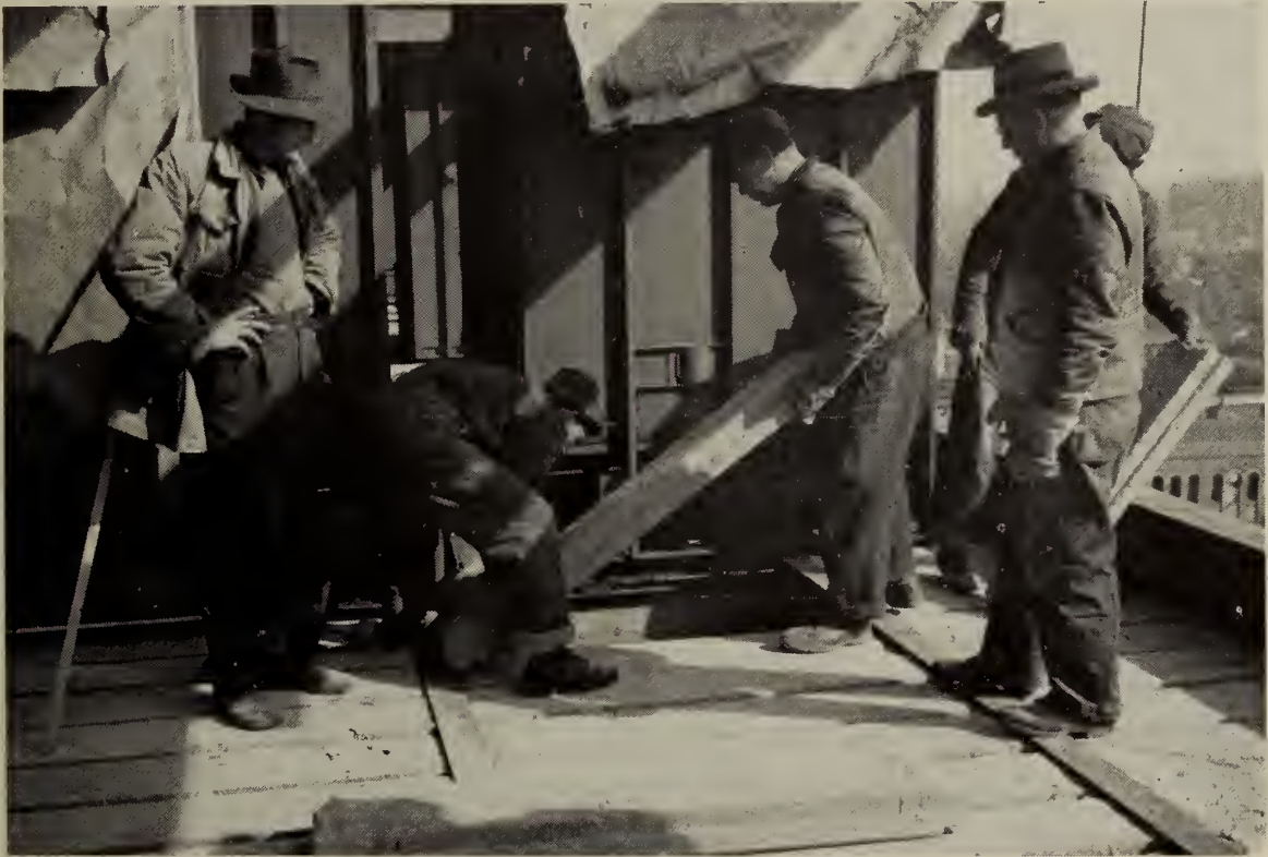
The above picture shows 4" precast Aerocrete slabs being laid at the new Laurentien Hotel, Montreal, in which all the floors and roofs (both Aerocrete and channel-type slabs) were supplied and erected by the Aerocrete Construction Company, Limited.
