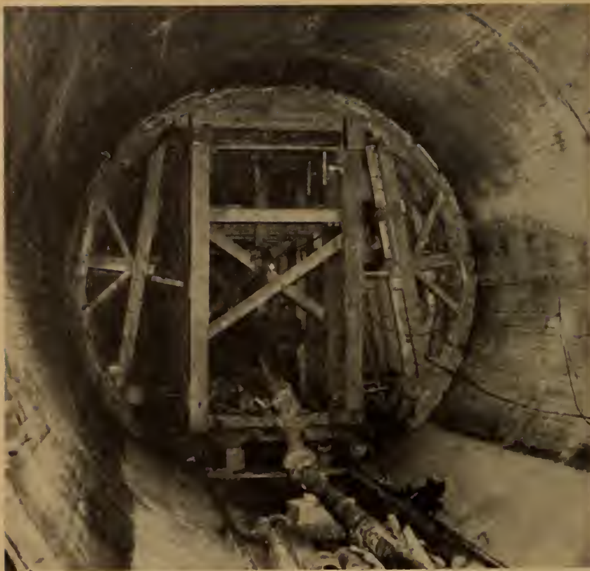
Fig. 7. Pouring concrete in diversion tunnel, St. Mary Dam, using travelling form for the crown.
