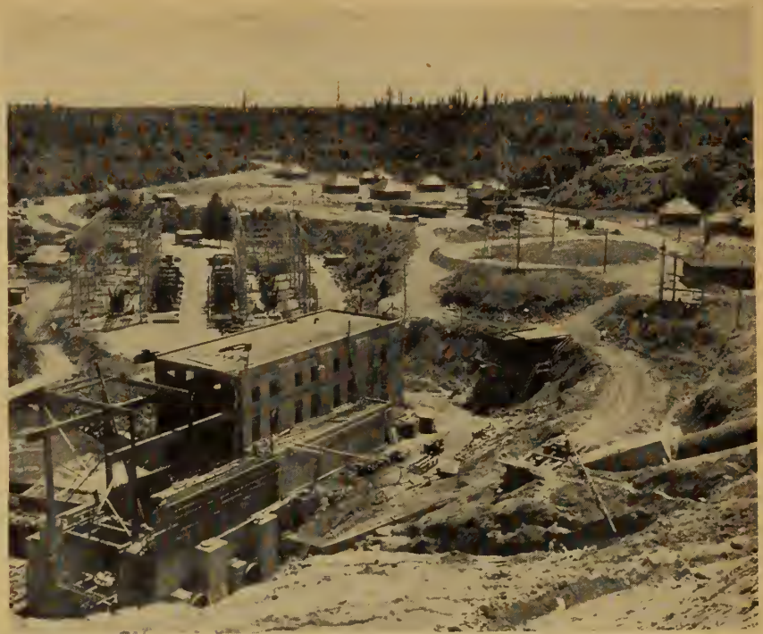
Powerhouse and penstock in foreground. Switching station and operators' cottages at rear.
