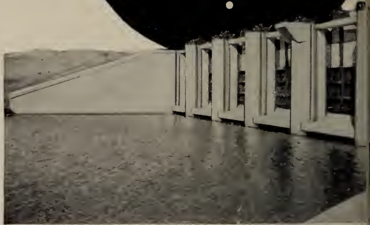
P.F.R.A. project in Saskatchewan, East End Dam Spillway showing gates. Constructed by W. B. Ramsay, Regina.
