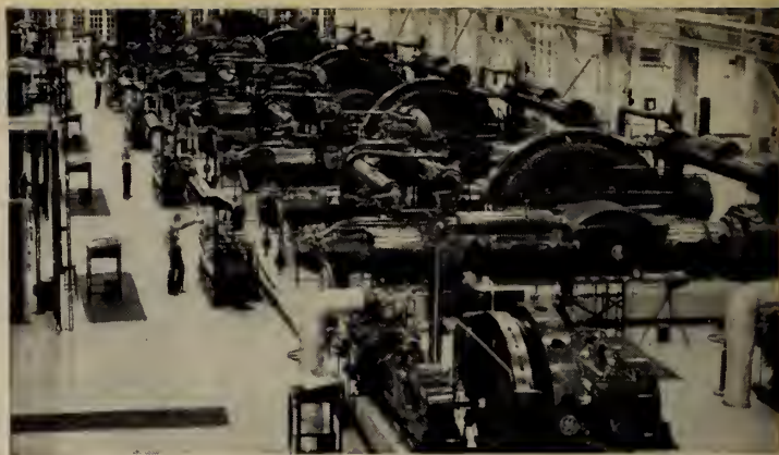
... five 2500 hp 5000 PSI gas compressors installed in a Canadian synthetic ammonia plant.
