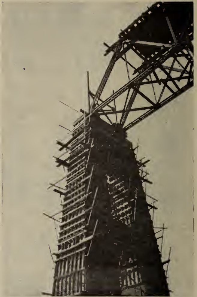
Fig. 3. View showing north approach span landing on Pier 3—July 1947. Photo by J. W. Copeman, resident engineer.
