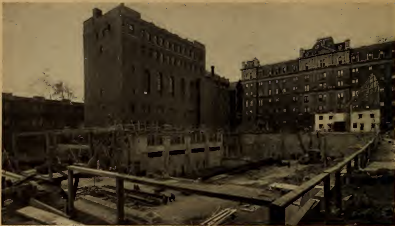
Above —Foundations completed and arrival of the first structural steel on the site. October 10, 1946.
