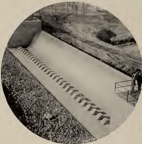
Concrete overflow dam with dentated sill, Wawanesa, Manitoba. Dutton Brothers, Winnipeg, Contractors. P.F.R.A.
