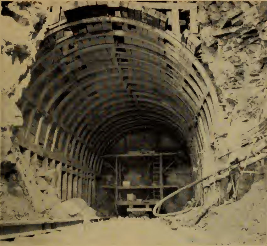
Fig. 5. Tunnel supports at inlet end of the diversion tunnel, St. Mary Dam.
