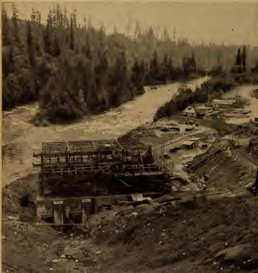
Construction of power house at Trout Pool, showing entrance to two of six turbine units and location of centre penstock and wye.
