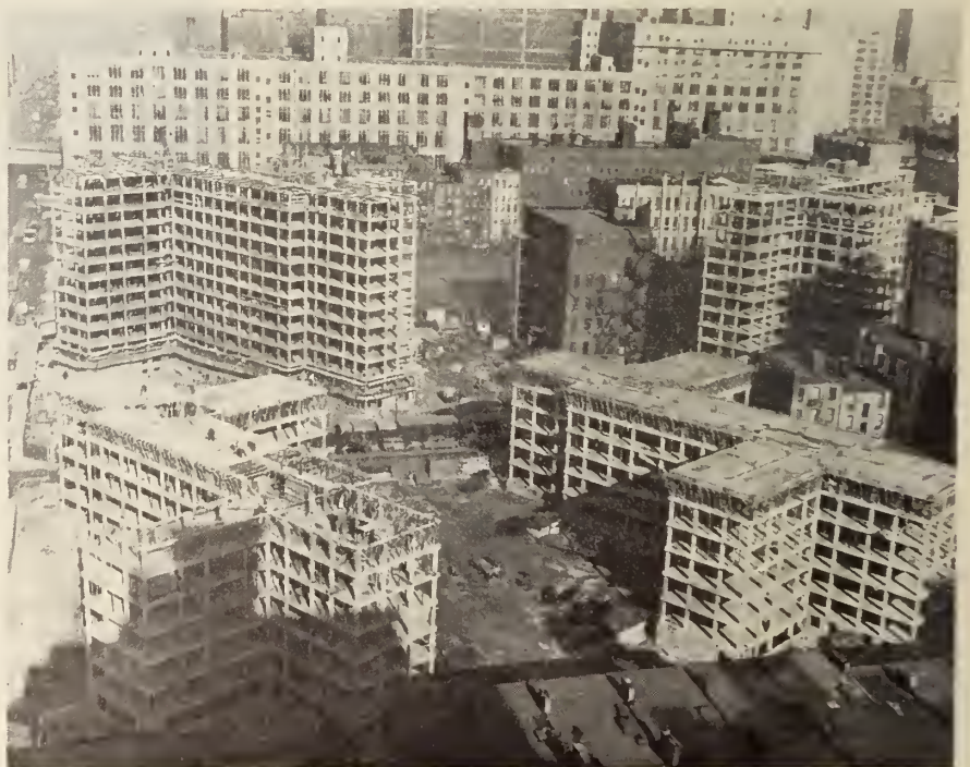
Elliott Houses. First project undertaken after the war, in the fall of 1945, and financed entirely by the City of New York. This was the first use in New York of the cavity wall construction which has saved $75 per apartment.
