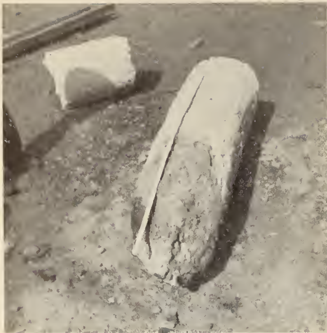
Fig. 2—Example of a waisted and fractured pile.
