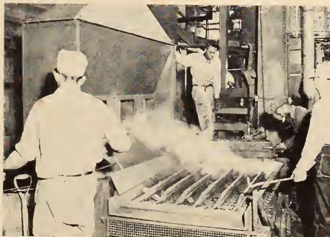
Fig. 4. A sidedraft exhaust hood on a casting shakeout process. Courtesy Kirk & Blum Manufacturing Company, Cincinnati.
