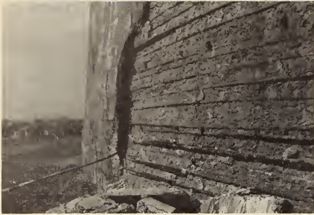
Fig. 2—Loose outer shell and partially exposed reinforcing.
