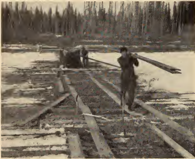
Fig. 2—Close-up of corduroy crossing, Petitot River. Planks taken from tent siding left by Canol project.
