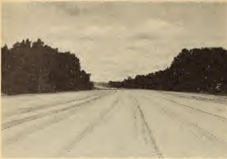
Fig. 2—Sub-grade on a level stretch of the new Toronto-Barrie highway, showing width and easy alignment.
