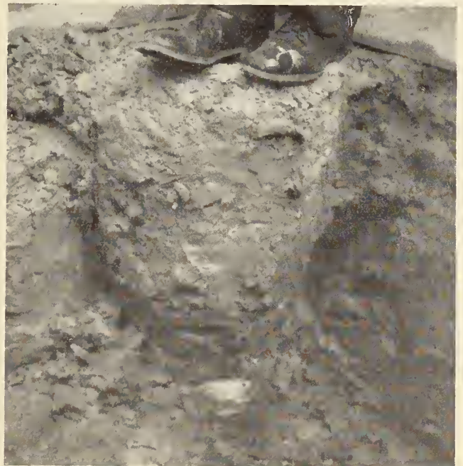
Fig. 1—Typical example "waisting" found on concrete piles.
