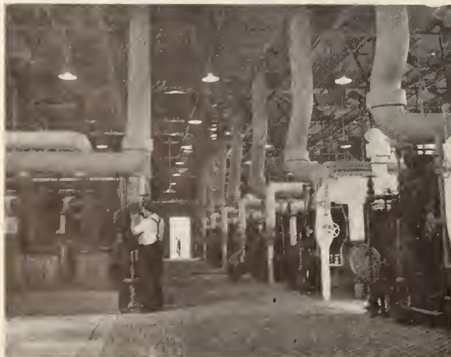
Fig. 8—Fuel gas driven compressors. Butyl rubber plant.
