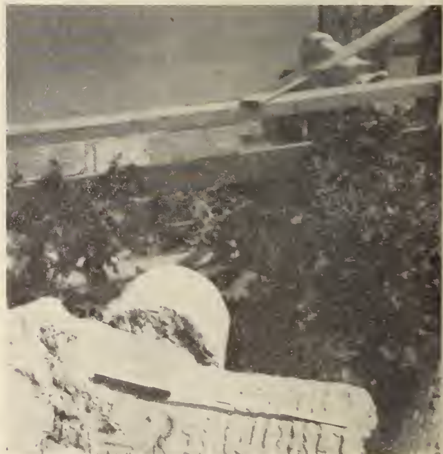
Fig. 3—Typical corrugations in upper portion of concrete piles through top hard clay layer.
