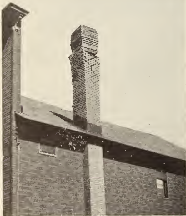
Fig. 11—Mushroomed chimney at Massena, N.Y. This chimney was damaged by the earthquake of September 5, 1944. When a building is very close to the epicentre of an earthquake of which the focus is deep, the chimneys are disintegrated by the almost-vertical shocks. The bricks are loosened but do not fall. It is an excellent sign that one is close to an epicentre.
