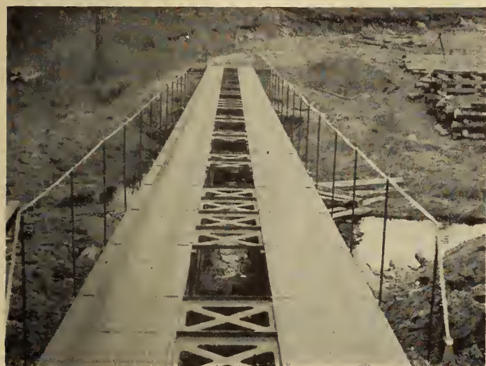
Fig. 8—View along the decks of the 100 ft. span showing double bridge brace frames in position.
