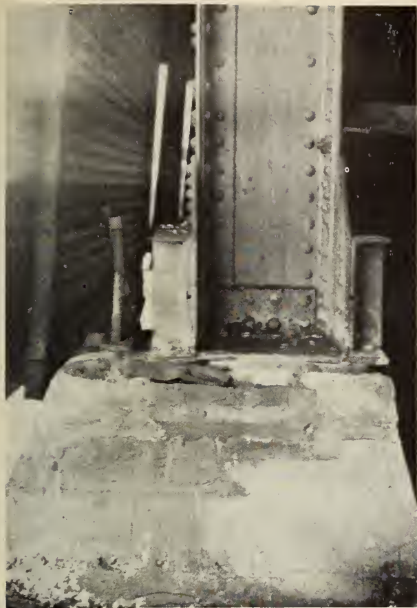
Fig. 4.—Base of steel strut supporting loading sheds at Quebec, shifted by the earthquake of February 28, 1925.
