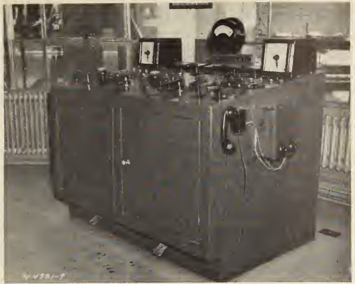
Fig. 12—Operator's desk on top floor of C.T.C. tower.
