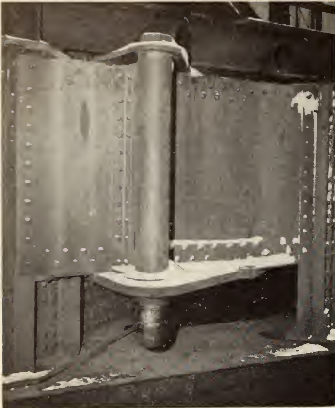
Fig. 6—Centering pin on end of a movable span. This photo was taken with span partly raised. When span is lowered the lower end of pin enters snugly into a round hole in a heavy steel plate riveted to the adjoining fixed span.
