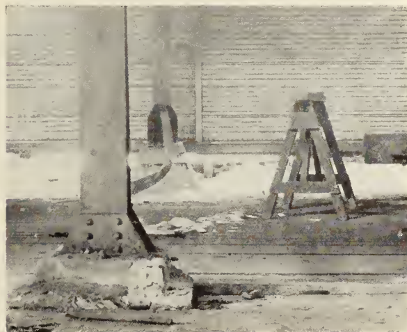
Fig. 5—Back brace at base of loading shed strut, bent by shift of the base of the strut, due to earthquake of 1925.
