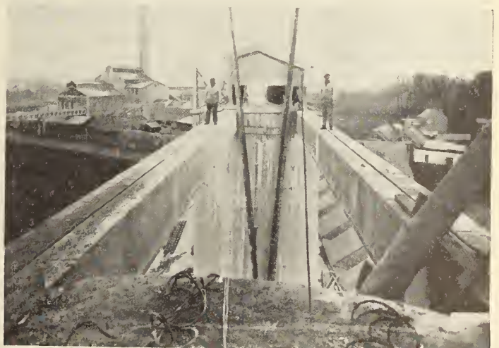
Fig. 8—Pre-compressed concrete beams erected in Belgium to form a bridge between grain elevators.
