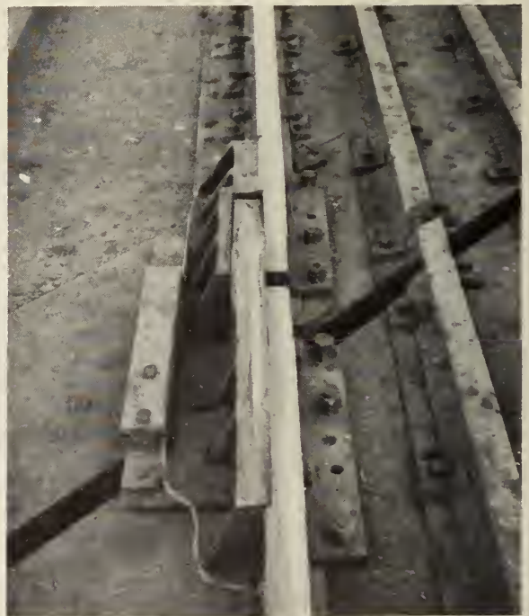
Fig. 7—Rail break assembly. Note the slightly raised casting that carries the treads of the wheels across the gap in the main running rail. The low flat unit to the left of the rail break is an enclosed mechanism for automatically making or breaking the track side of the electric traction circuit when span is raised or lowered.
