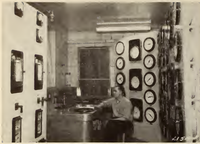
Fig. 14—The compact control arrangements for the initial two electric boilers are shown to the left. This will be duplicated to the right, when additional boilers are added. The panels at the operator's back are the load dispatching board.
