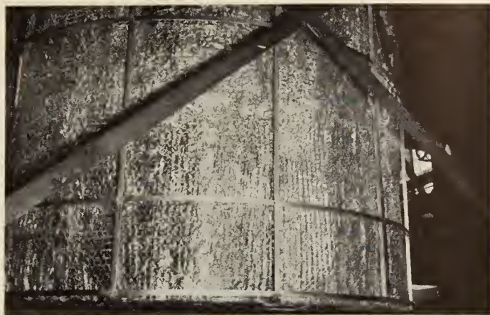
Fig. 7—Preformed aluminum foil-air cell heat insulation applied on vertical portion of electric boiler shell.
