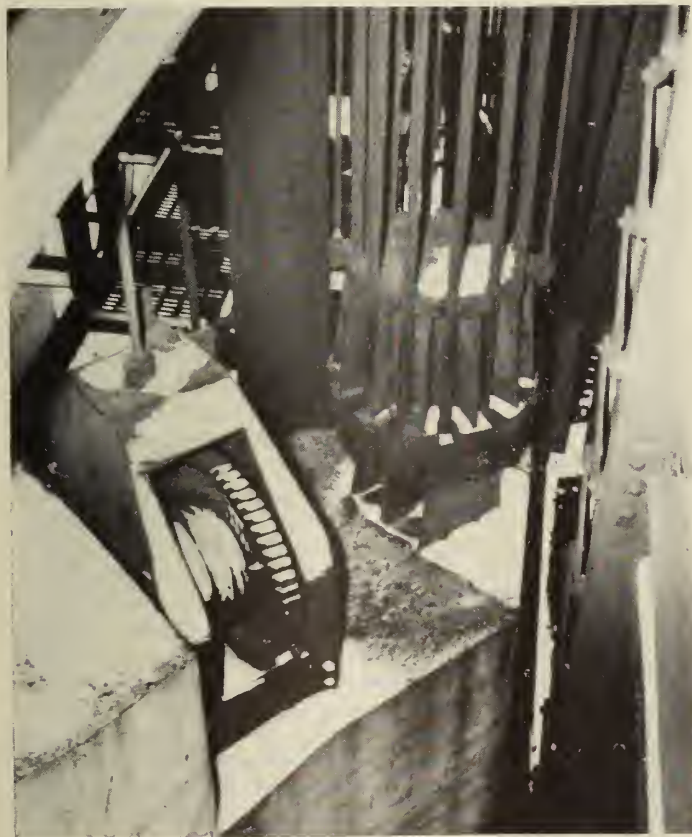
Fig. 8—Showing attachment of counterweight cables to end of a concrete counterweight. Steel framework to which cables are attached is actually part of a structural steel construction buried in the concrete counterweight. The mechanism in the left foreground is for adjusting the tension in the main operating cable.
