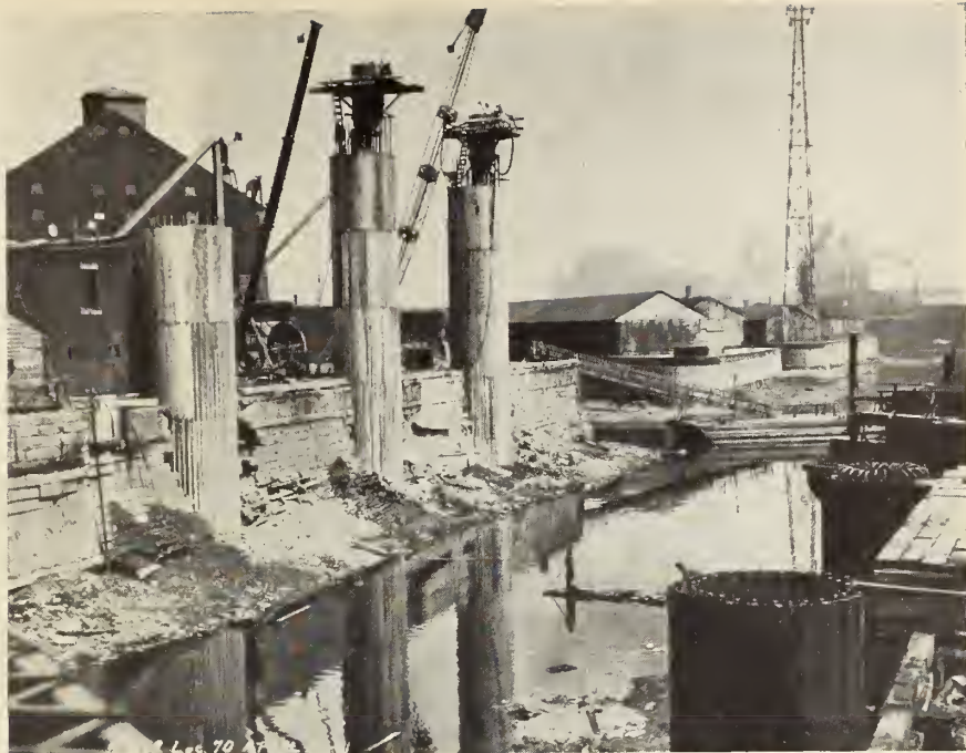
Fig. 4—Showing three wood stave pneumatic caissons being sunk on the shore of the canal. Photo also shows the tops of three completed steel sheet piling caissons on the right side of picture.
