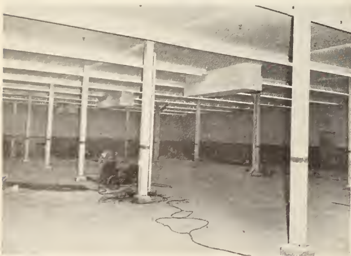
Fig. 4.—Spinning room before installation of machinery.
