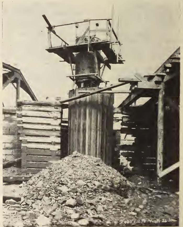
Fig. 3—Steel sheet piling caisson with air lock. The pile of material in the foreground consists of shale and disintegrated stone removed from the surface of the solid lime stone rock.
