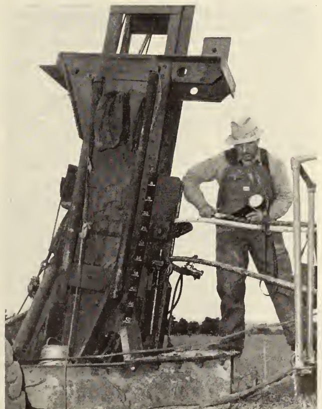
Fig. 1—Gas pressure reading being made on cable prior to entering plough sheath.
