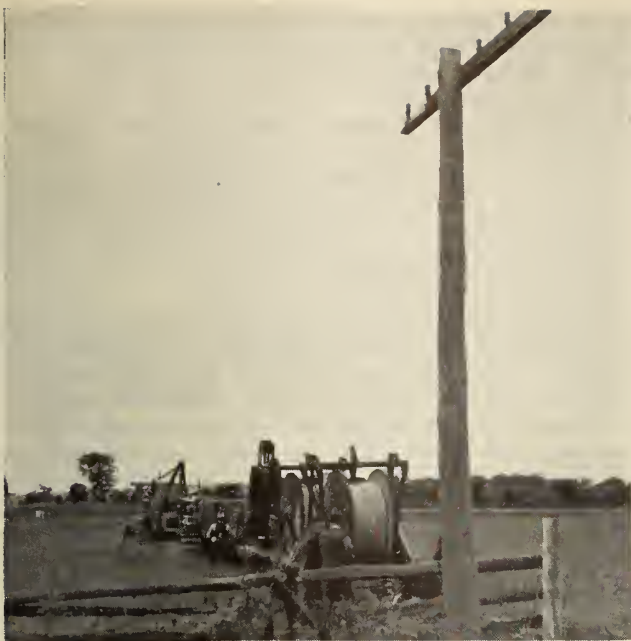
Fig. 3—Plough train in operation across flat country. Open wire line in foreground.
