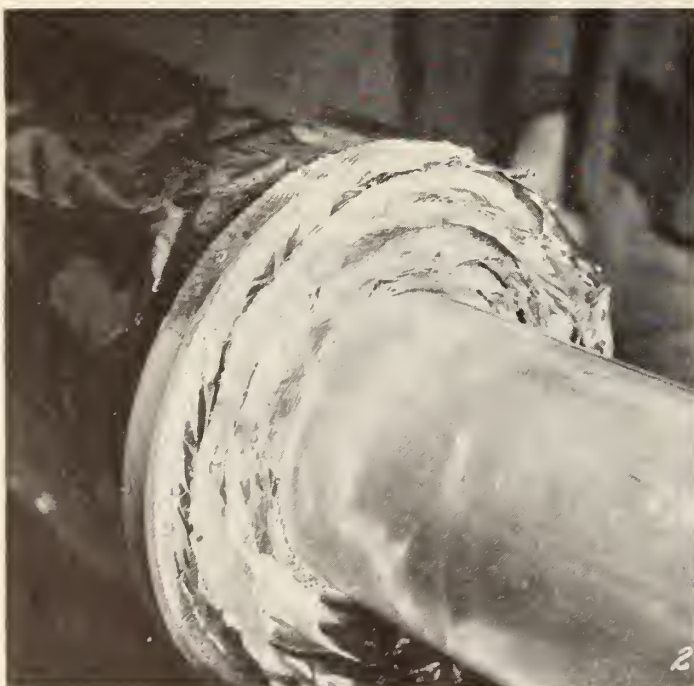
Fig. 10—Helicly-wound aluminum foil-air cell heat insulation on pipe for use with cold water.
