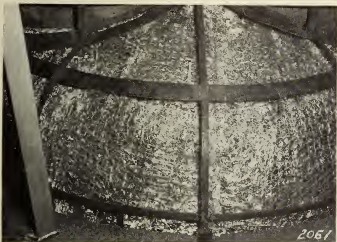
Fig. 6—Preformed aluminum foil-air cell heat insulation bats applied to upper head of electric boiler.
