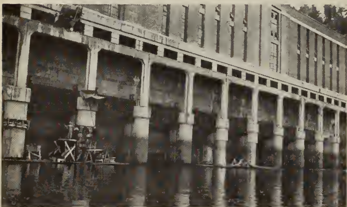
Fig. 4—Tailrace piers under repair. Reinforced concrete covering is applied approximately 6 in. thick. Repaired pier at left. Disintegrated concrete removed from two piers at middle right. Disintegrated condition of concrete on piers at normal water level before repairs is indicated by piers near right. (In this picture the water has been lowered while the repairs proceed.)
