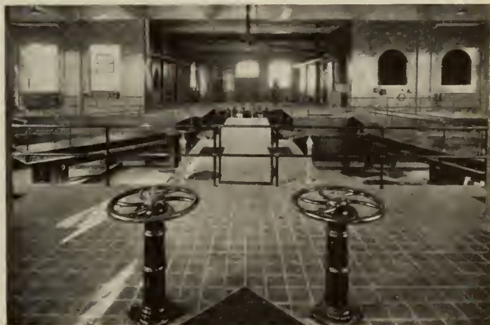
Fig. 5—Sewage Screening Plant, Hamilton, Ont.
