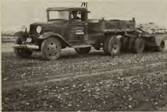
Fig. 5—Runway Construction at Medicine Hat, Alta., Wobble Wheeled Rubber Tired Roller Compacting Base Course.
