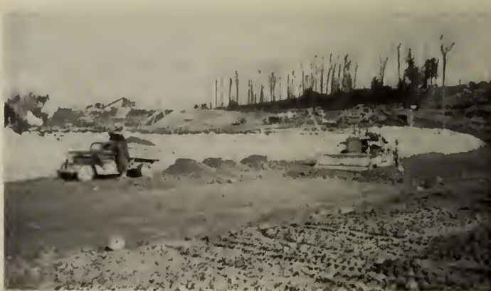
Fig. 14—Pervious zone construction: dumping, spreading in 12-inch layers, and compacting with tractor.
