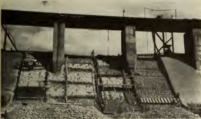
Fig. 1—Reinforced concrete covering on spillway dam. Thickness 12 to 30 in. depending on condition of old concrete. At left: old concrete surface. Left centre: chipping proceeding. Centre: chipping including joints completed. Right centre: reinforcing installed, joints concreted in. Some of the latter contain concrete tile for drainage of leaks. Right: completed covering.
