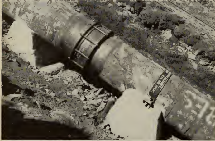
Fig. 10—The Choquetanga Penstock-Johnson Joint.
