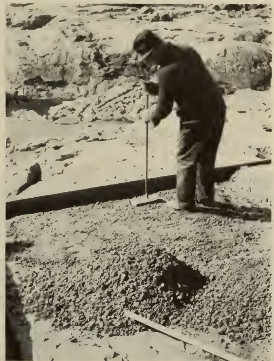
Fig. 2—Placing thin non-reinforced covering at toe of spillway dam shown in Fig. 1. This covering is 3 to 6 in. thick; strength, 4,000 to 5,000 lb. at 28 days. Note the cement bonding coat on the old concrete in the foreground. This type of covering is applied where the old underlying concrete is reasonably strong. After 3 years under severe exposure facing in a southerly direction, including spilling conditions and passage of ice in the spring, this covering showed no appreciable deterioration.
