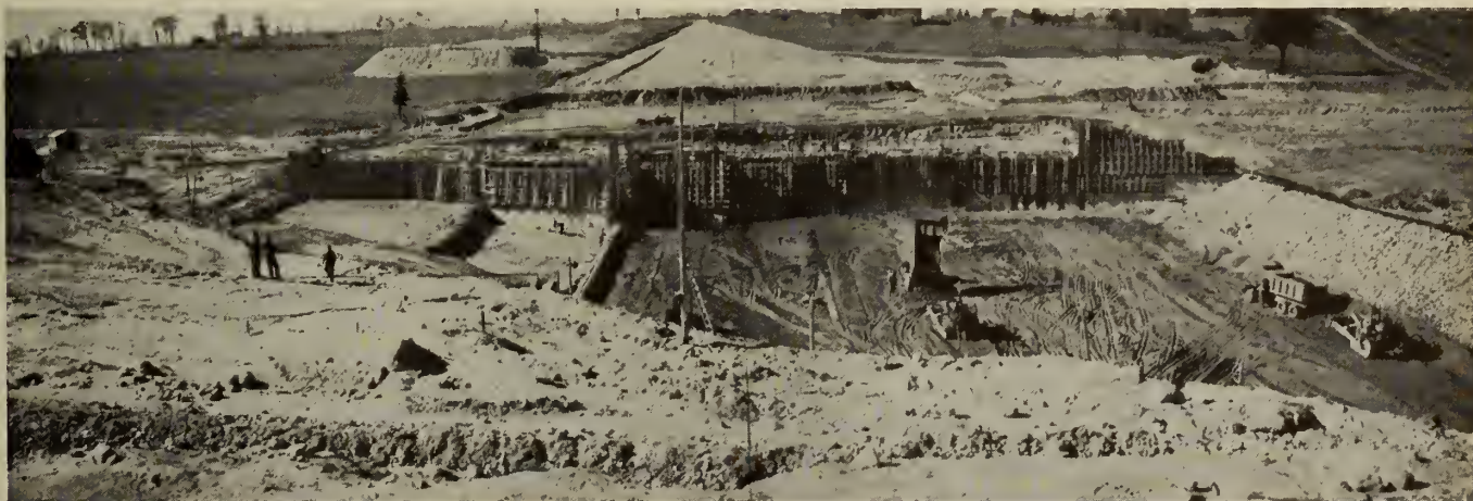
Fig. 12—General view from east abutment, October 1939; east embankment fill being constructed; filter bed and key wall still visible.
