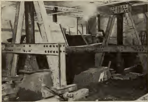
Fig. 5—A-frame shores for steel columns, showing old footing drawn sideways and one column with new footing and extension complete.
