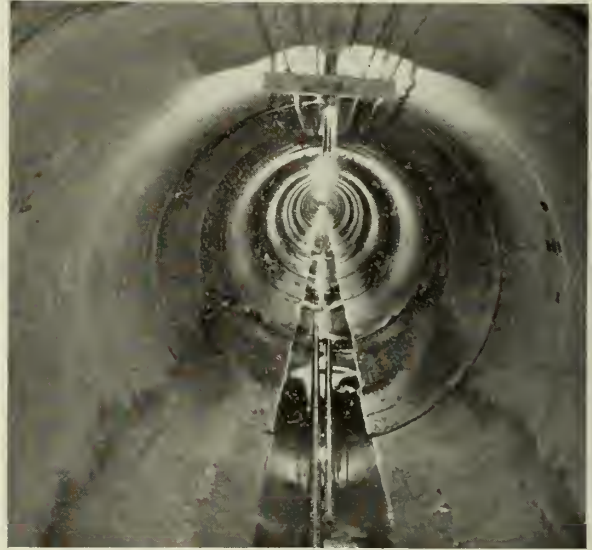
Fig. 14—Grout Holes Discharging Water.
