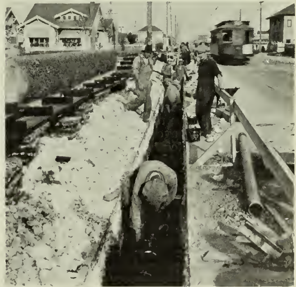
Fig. 6—Insulating Laterals for Hot Water Line, Academy Road.
