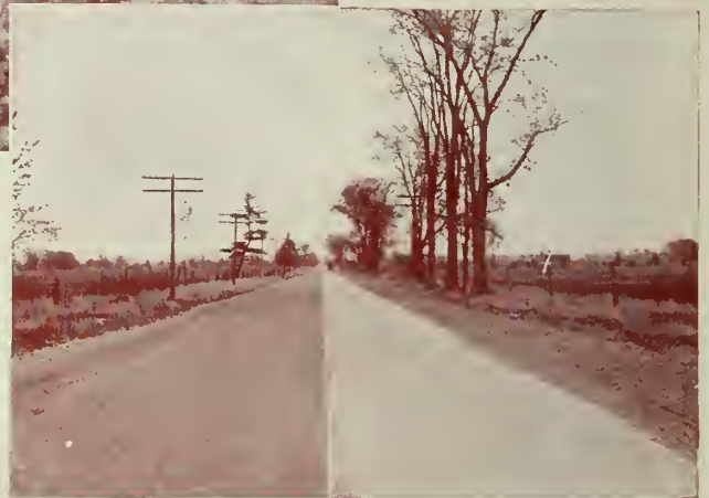
Above:—Single track concrete road under construction, Waverley South, Ontario. Sterling Construction Co., Windsor, Contractors.
