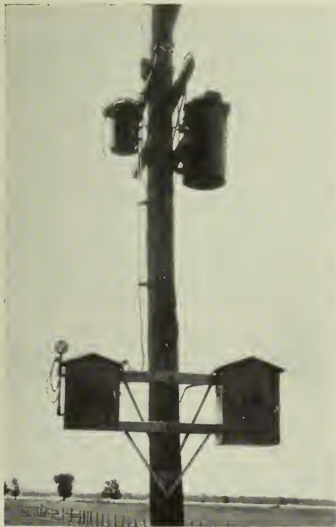
Fig. 4—RO Transformer, Novalux and Photronic Controls and Metering.
