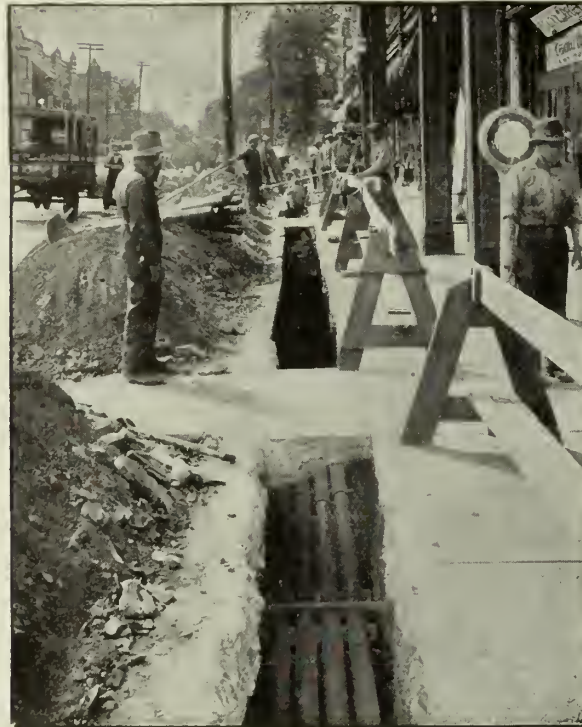
A 16 duct run of Cornwall Fibre Conduit being installed on Park Avenue, Montreal, in August, 1933.
