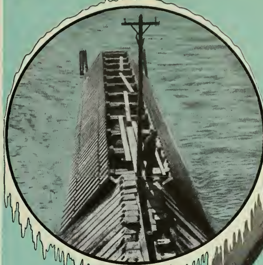
The rebuilding of these jetties was carried out under the supervision of Lieut. Col. C. L. Sturdevant, Army District Engineer. Construction labor under direction of E. F. Bauer, Associate Engineer.
