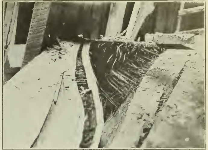
Figure No. 18.—View showing Failure of Timbers in Pit H, August, 1927.
