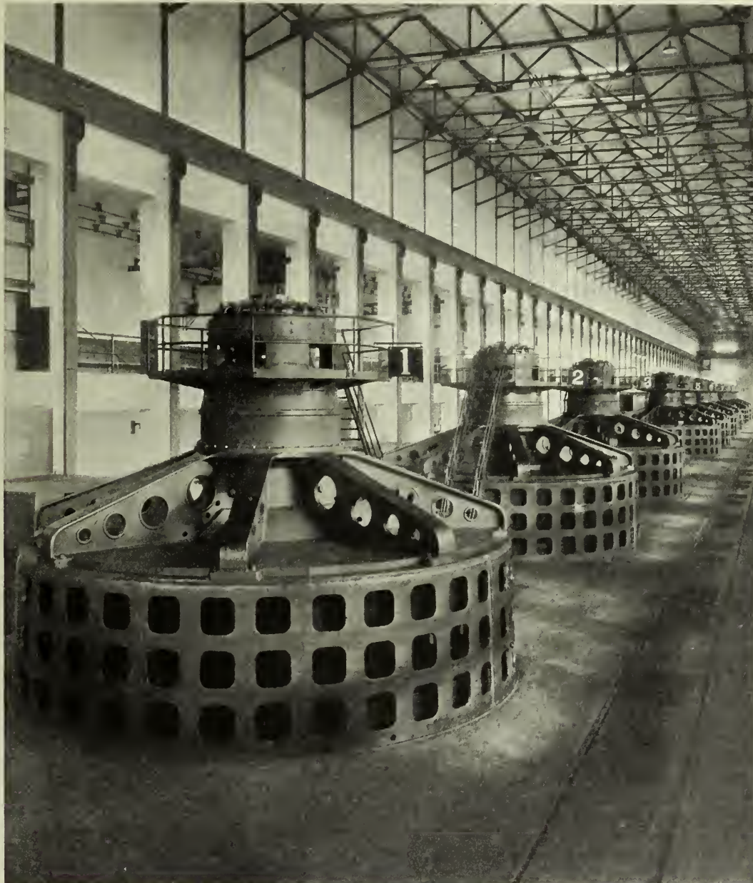
Figure No. 6.—Ten 30,000-kv.a., Vertical Shaft Generators in Isle Maligne Plant of the Duke Price Power Company.
