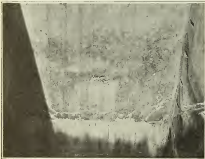
Figure No. 11.—A Stone Pocket in a Concrete Slab.
