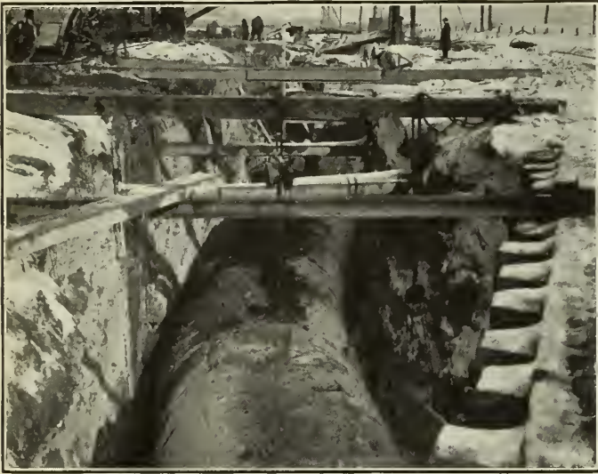
Figure No. 6.—General View of 10' 0" Sewer, Looking Eastwards from Intersection of Canadian National Railway.
