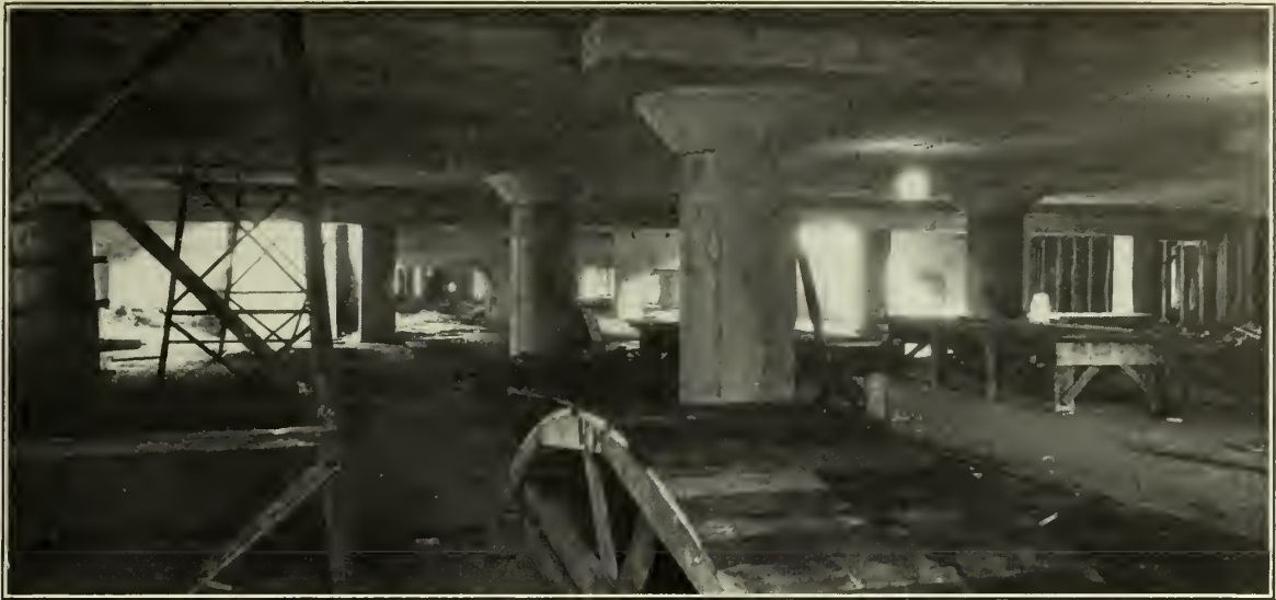
Figure No. 14.—Portion of Train Waiting Room (El.15.5) after Stripping the Forms.
