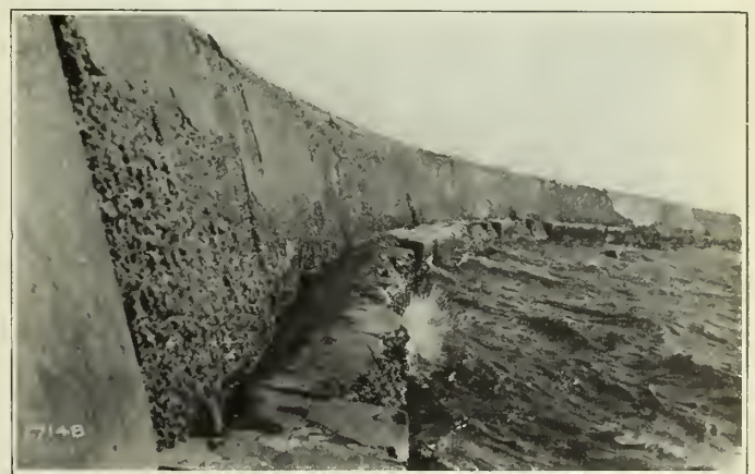
Figure No. 7.—Breakwater Built in 1906 with 1:3:5 Concrete, Illustrating the Effect of Waves and Frost on Porous Concrete, Resulting from too Lean a Mix.
