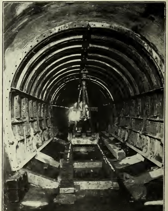
Figure No. 9.—Interior of Sewer, Station 3+78, Looking Westwards, showing 120 ft. of Blaw Knox Steel Forms.
