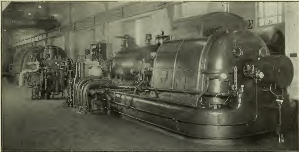
Figure No. 10.—General View of 1,200-pound Turbine Generator Units at the Edgar Station.
