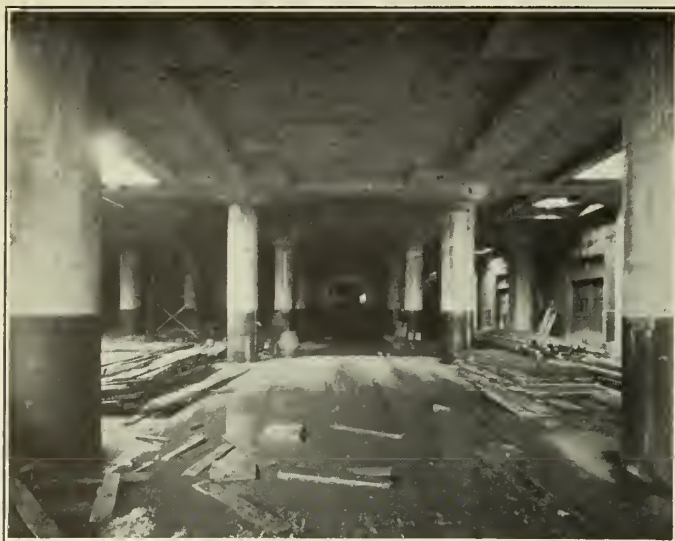
Figure No. 9.—Interior View of the Post Office Area showing Construction around Elevator Hatchways.
