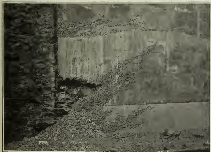
Figure No. 13.—An Extreme Example of Segregation Caused by Depositing the Concrete at the Central Point and Allowing it to Flow into Place.
