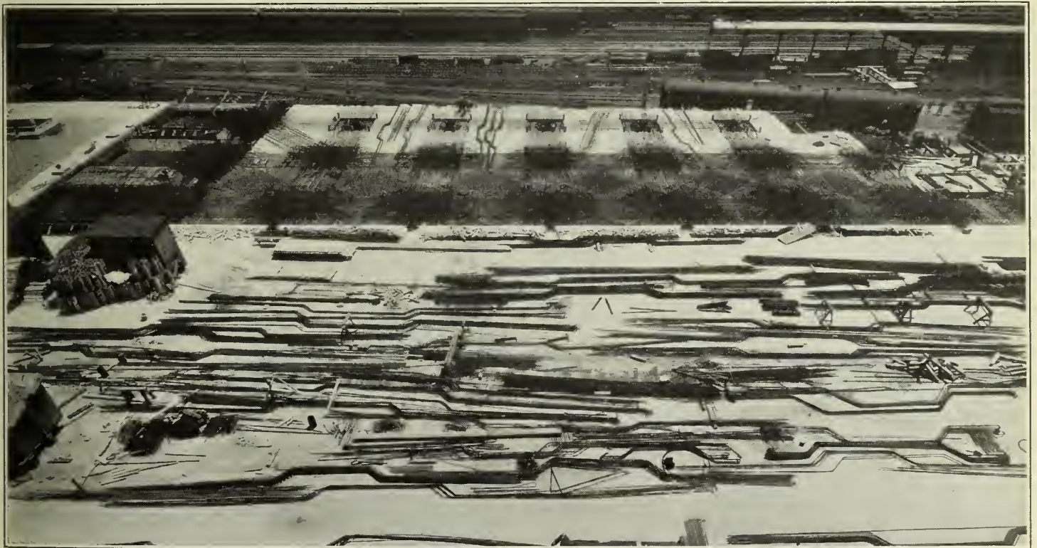
Figure No. 8.—View Looking South from Station Building showing the "Four-way" Reinforcing in Place in the Background and a Portion of the Finished Slab in the Foreground.
