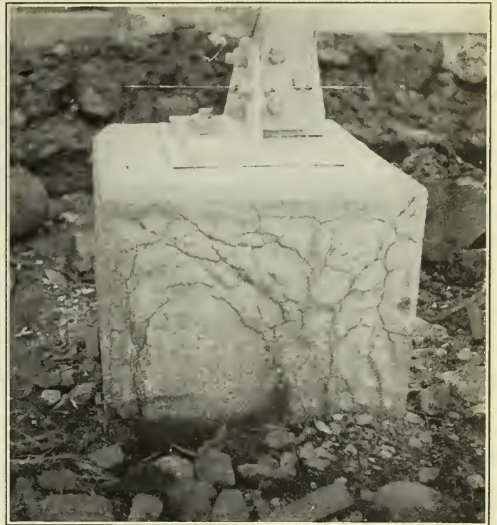
Figure No. 17.—A Concrete Footing Built in the Late Fall. It was protected until hardened, but never had a chance to cure properly. In the spring it became saturated with water and was frozen.
