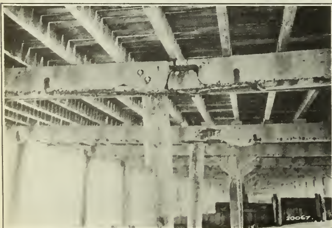
Figure No. 5.—Failure of a Concrete Beam Caused by Corrosion of the Reinforcement Followed by Spalling of the Concrete.
