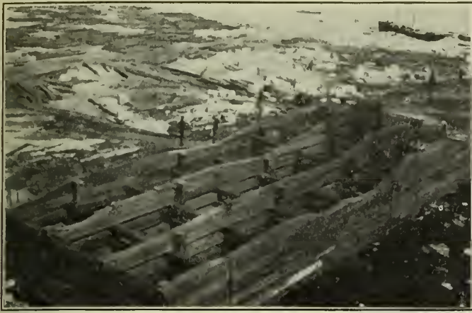
Figure No. 15.—Construction of Timber Crib for Wharf. Crib, 100 by 27 feet, constructed on three small piers prior to overturning and floating into place.
