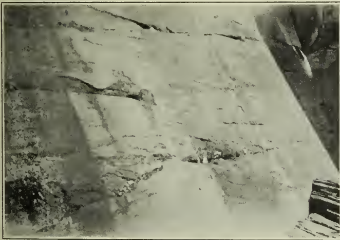
Figure No. 9.—A Concrete in which Pockets and Seams of Laitance were Allowed to Remain.
