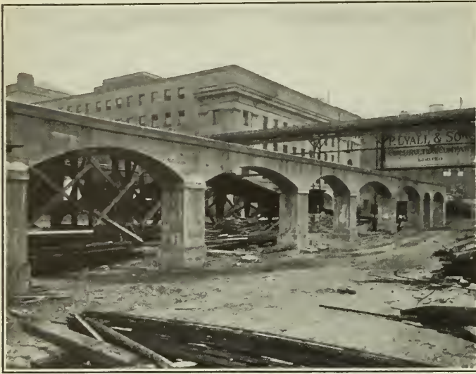
Figure No. 12.—One of the Arch “Bents” on Bay Street Subway which Support the Steel Spans Carrying the Overhead Tracks.
