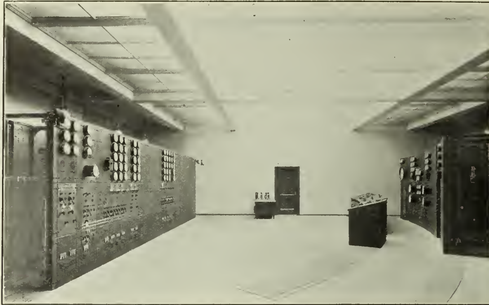
Figure No. 13.—View of Operating Room at Edgar Station.
