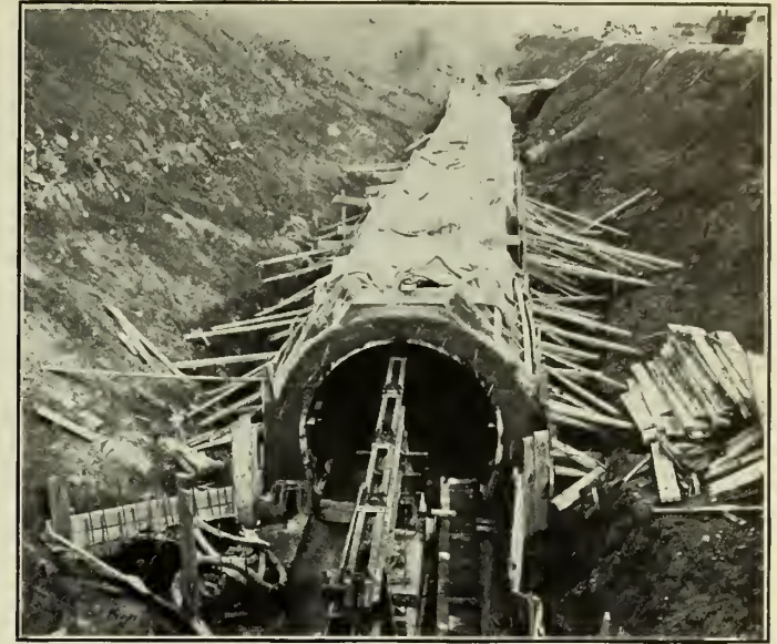
Figure No. 12.—View of End of 9' x 9' Sewer (Station 70 + 77.5) and Invert of Junction Chamber.
