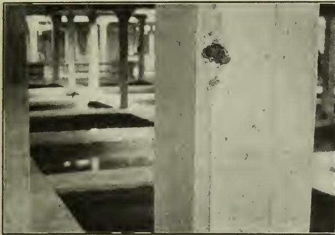
Figure No. 21.—Spalling Caused from a Piece of Aggregate Containing Considerable Sulphates.
