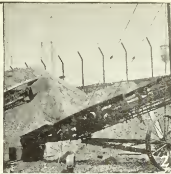
2—Another McCord Radiator scene. The feeder, in a permanent track hopper, feeds to the first conveyor, which relays the coal to the second conveyor. In this manner, a car was unloaded in 50 minutes. This equipment saves the company $17.31 on every car handled.
