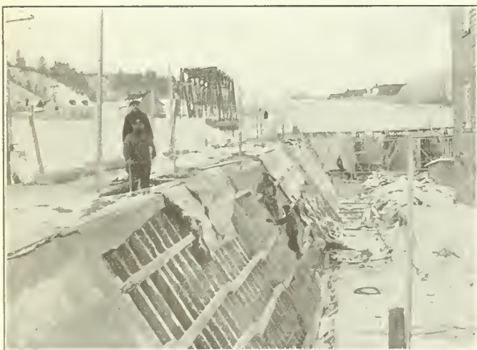
Figure No. 1.—Gravity section wing wall poured in January 1923, with a temperature variation of +20°F to -30.5°F.
