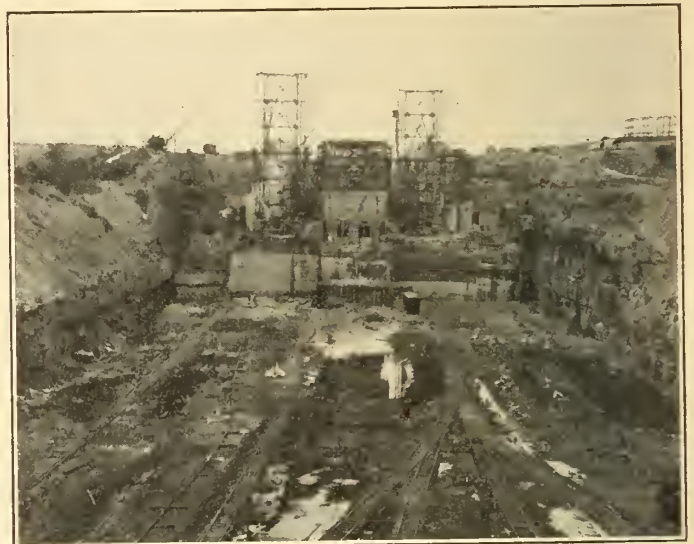
Welland Ship Canal Flight Locks looking south from Grand Trunk Railway Bridge. A general view of the construction of the Flight Locks at Thorold showing the pit for Locks No. 4 and the breast walls of Lock No. 5. Photograph taken June 17th, 1925.
