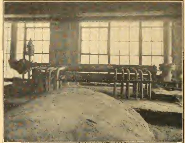
View showing ELESCO Superheater header with units at plant of Illinois Central R.R. Amboy, Ill.
