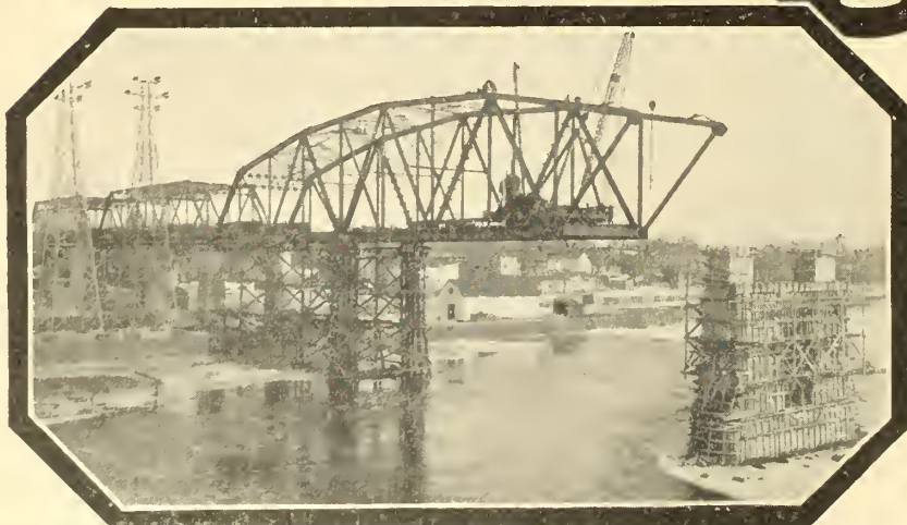
Galipeault Bridge—Ste. Anne de Bellevue. Built for the Province of Quebec, showing the 230' 0" span in course of erection.
