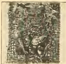
Self-contained strainer — note what this strainer removed in a short time.
