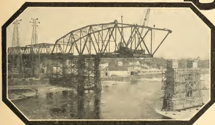
Galipeault Bridge—Ste. Anne de Bellevue. Built for the Province of Quebec, showing the 230' 0" span in course of erection.
