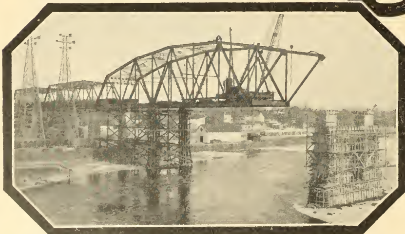
Galipeault Bridge—Ste. Anne de Bellevue. Built for the Province of Quebec, showing the 230' 0" span in course of erection.
