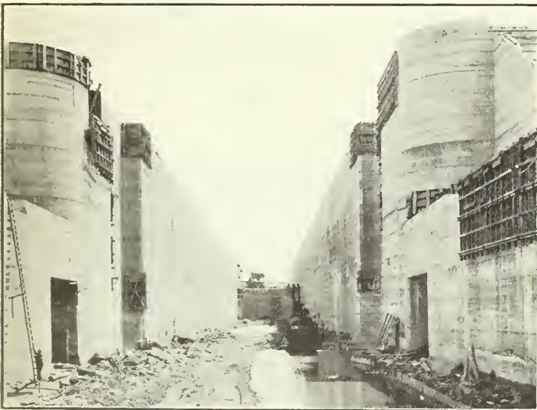
Welland Ship Canal, Lock No. 2, looking South. First work on this Canal commenced October 3rd, 1913.
