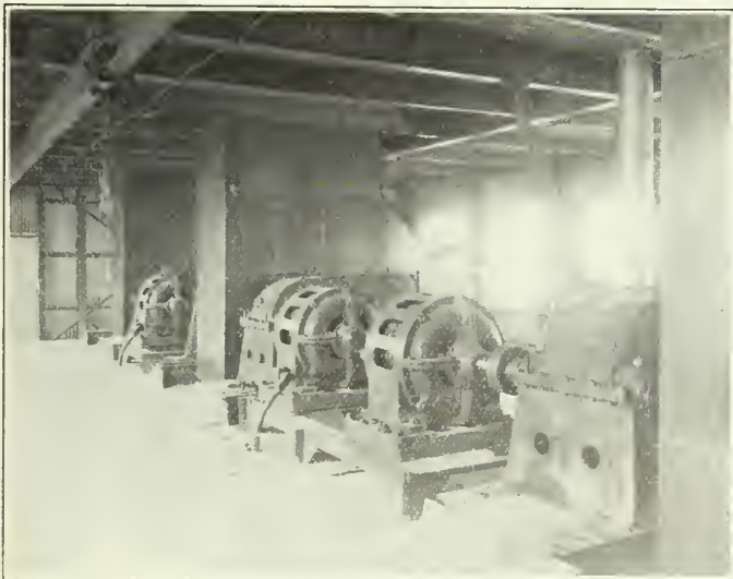
Figure No. 17.—Harbour Commissioners of Montreal Elevator No. 3, double reduction double helical gear drives to leg head.
