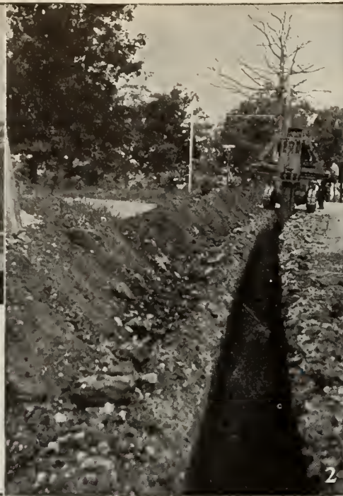
2—Notice the clean cut ditch, and the dirt pile placed well back from the cut.
