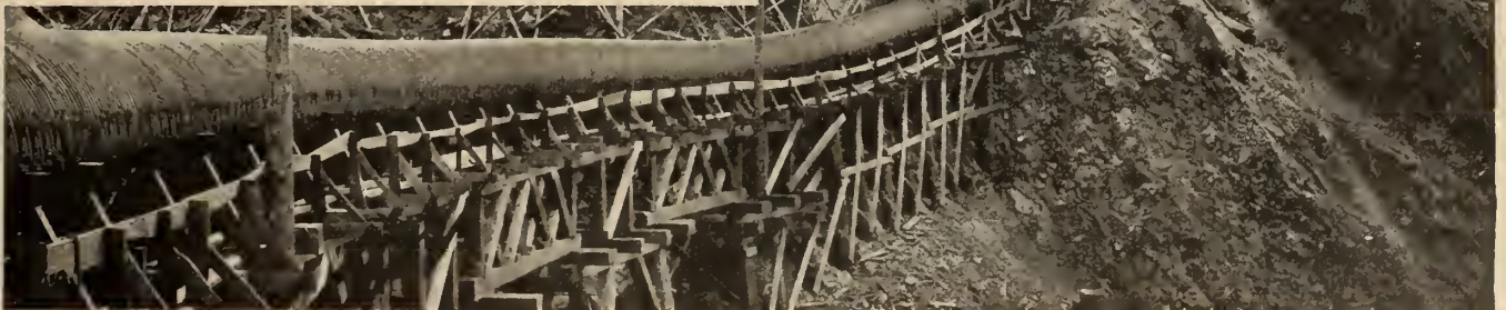
6-Foot Continuous Wood Stave Pipe Line at Anyox, B.C. 20 to 310-Foot Head.
