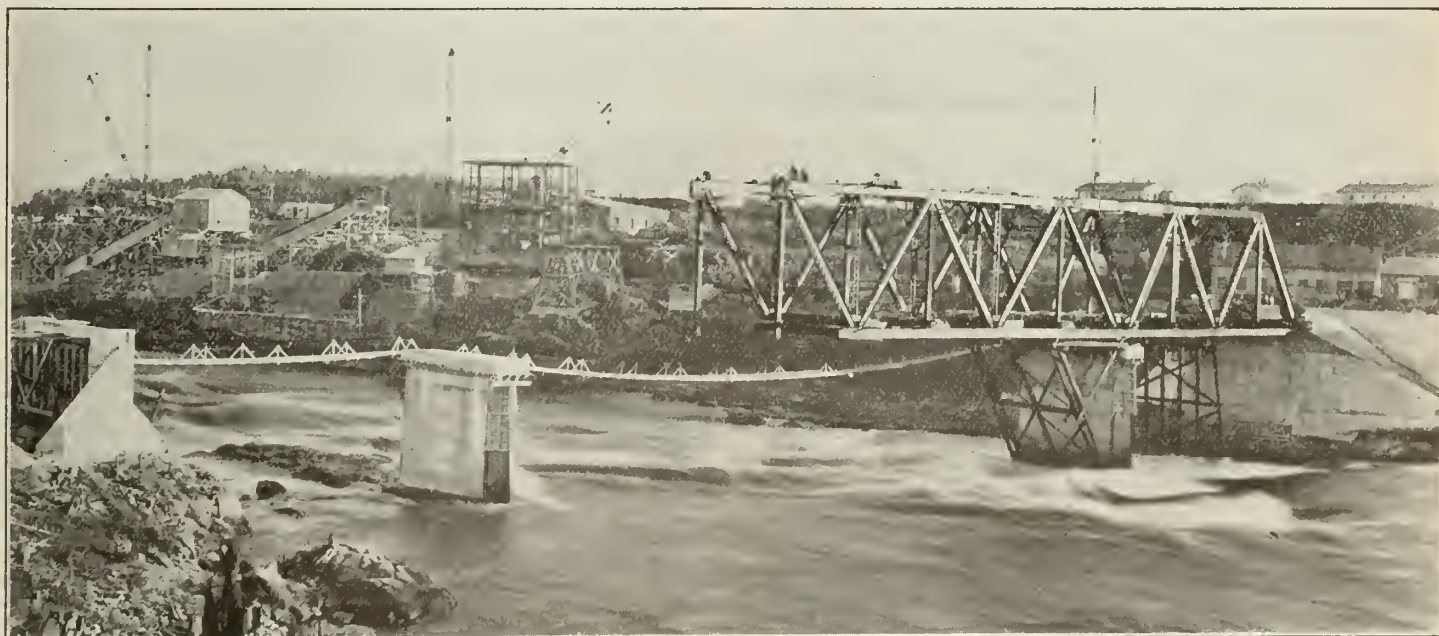
Figure No. 1. Grande Decharge Power Development. Erecting fifth panel of cantilevered span across right channel of the Grande Decharge, Saguenay R ver.
