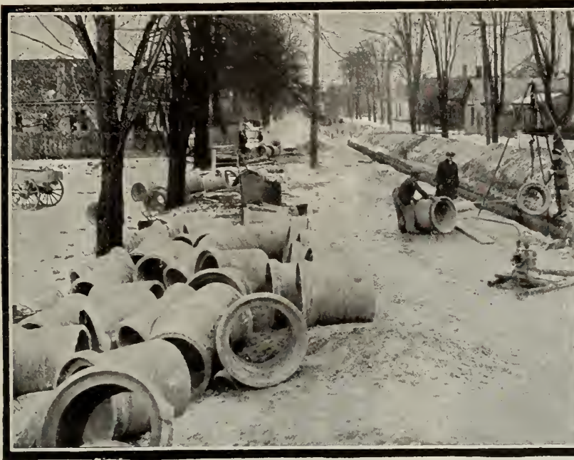
McCracken Concrete Sewer Pipe being laid in London, Ontario, for sanitary sewers.
