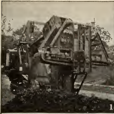
1—R. E. Sholes' Barber-Greene Ditcher cutting through hava going on a Raleigh, N. C., water main job. This photograph shows the discharge and the vertical digging boom.
