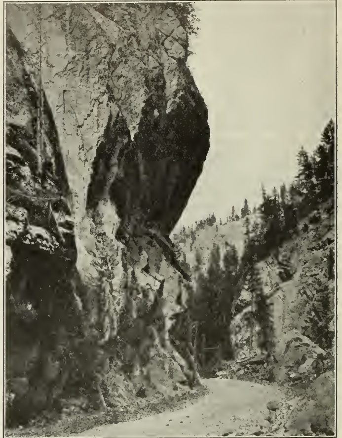
Figure No. 4.—Banff-Windermere Road, heavy rock work in Sinclair Pass. Final surfacing not done.
