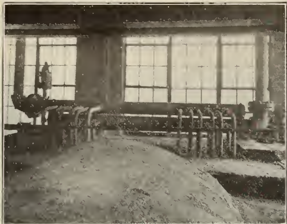
View showing ELESCO Superheater header with units at plant of Illinois Central R.R. Amboy, Ill.
