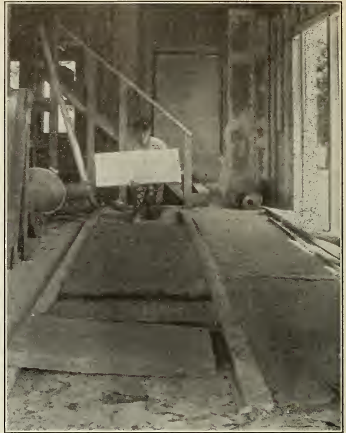
Figure No. 5.—Pre-casting Fireproof Insulex Slabs and Placing them between Furring Strips of Required Thickness for Wall Insulation.
