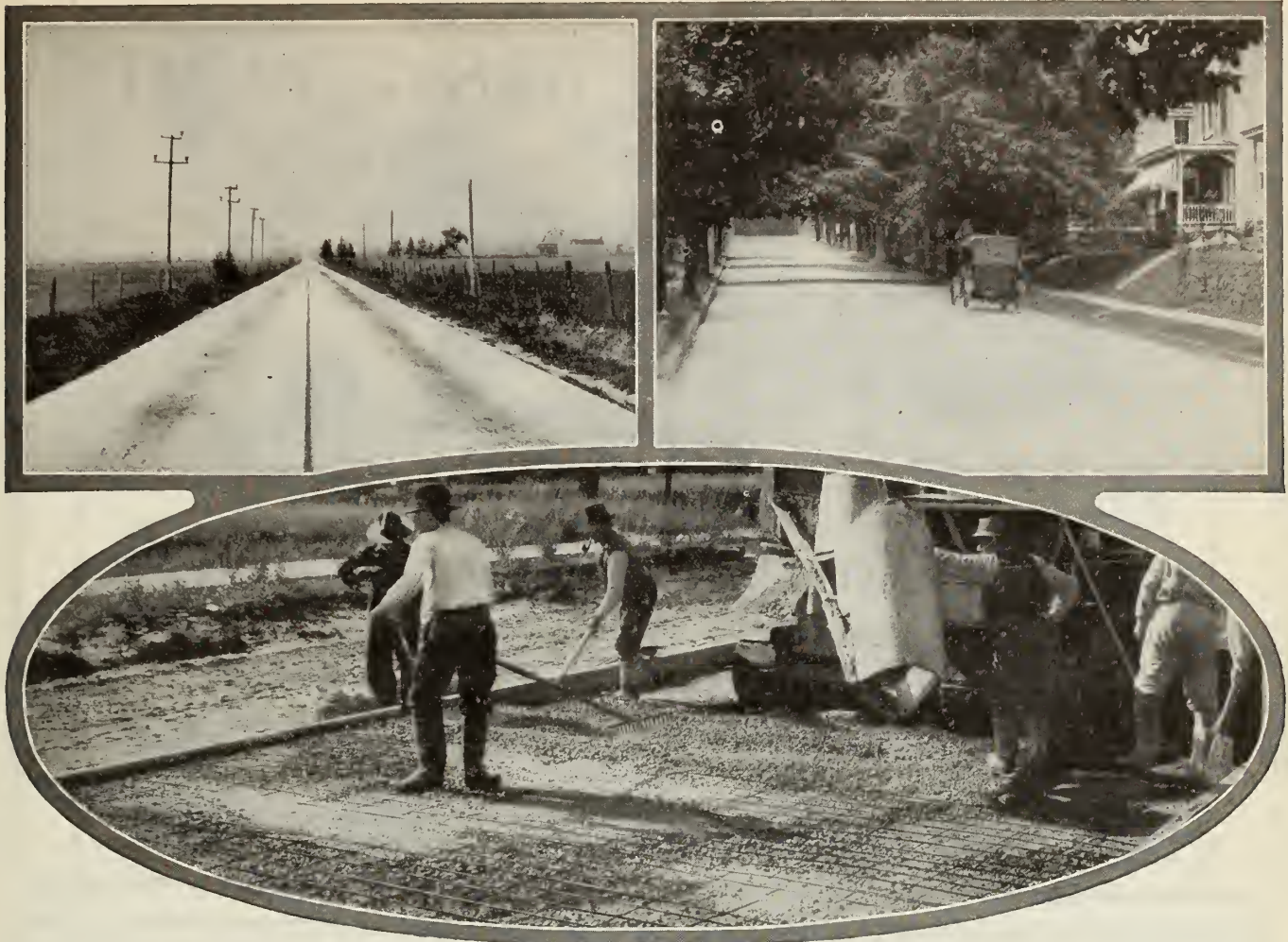
Upper left—Highway showing use of Truscon Dowel Contraction Joints and Wire Mesh. Upper right—Street view in residential section showing reinforced concrete road. Lower—Truscon Wire Mesh is the ideal reinforcement for concrete roads.
