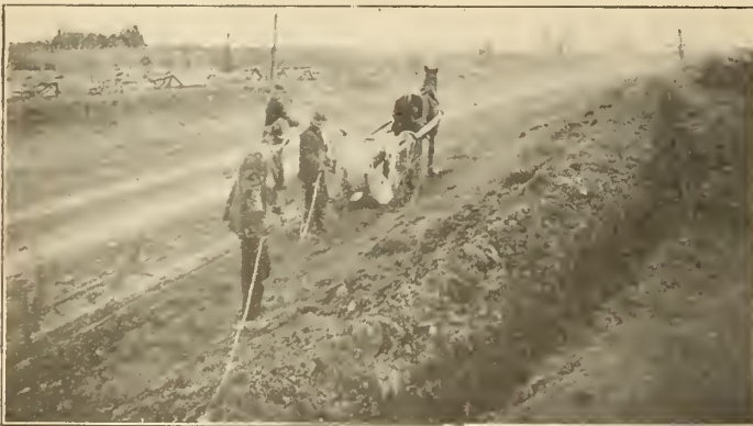
Plate No. 4b,—Underground Rural Transmission Lines. Trench excavated ready for installation of cable.
