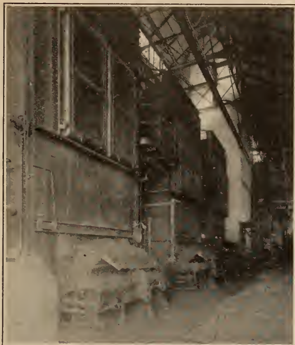
Taylor Stoker fired 400 H.P. Wickes Horizontal Water Tube Boilers. Operating at 150 lbs. pressure and 100 degrees Superheat.
