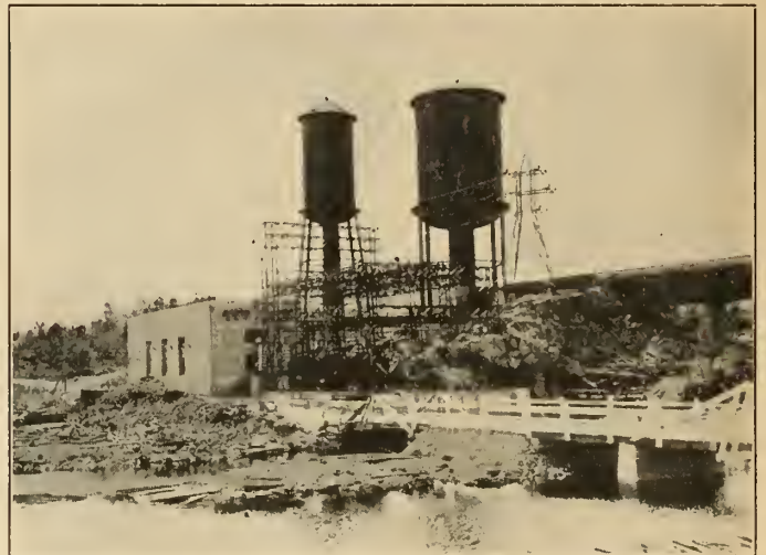
Musquash Development on the Musquash River, New Brunswick, of the New Brunswick Electric Power Commission — 11,000 h.p.
