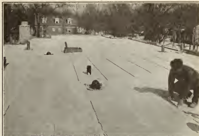
Figure No. 2.—Removing Temporary Screeds from Poured-in-Place Roof Insulex. After Filling the Screed Spaces the Roof Would Require to be finished on Top with a Commercial Waterproof Roof Covering.
