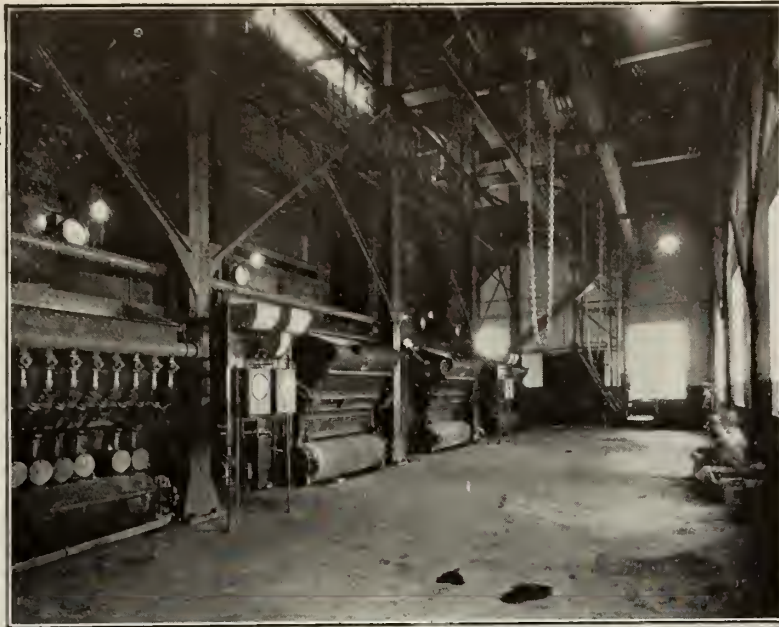
ABOVE — Four 336 H.P. KIDWELL Boilers with COXE Travelling Grate Stokers.
