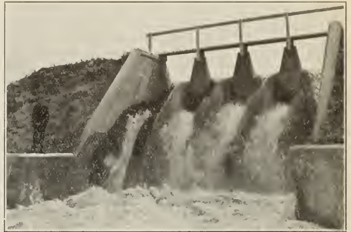
Fig. No. 6. Section A Canal near Strathmore, Alta. Drop No. 8A, Discharge 325 second-feet.
