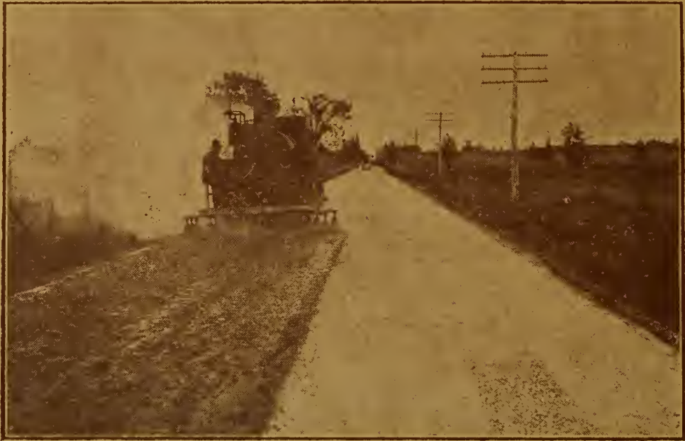
Asphalt Binder being applied by Bituminous Spraying & Contracting Co. Limited on Hamilton-Guelph Highway on Contract No. 619.
