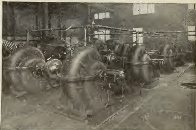
Four De Laval motor driven pumps at Toronto. In the official tests one of these pumps developed 87.2% efficiency when delivering 22,240,000 Imperial gal. per day against 267.6 ft. head.
