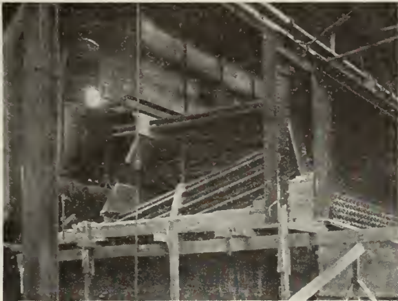
Superheater arrangement at The Farr Alpaca Company, Holyoke, Mass., where three 1046 h.p., Wickes Cross Drum Boilers equipped with Elesco Superheaters are carrying 125 degrees of Superheat at 150 per cent rating.
