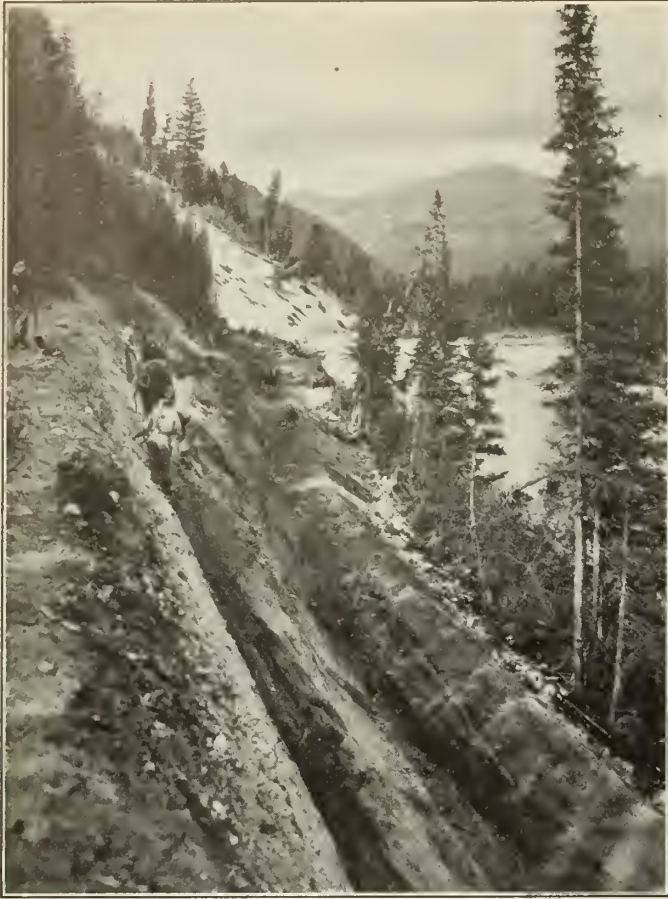
Figure No. 3.—Heavy grading along the Vermilion River, four miles east of the Kootenay Valley.
