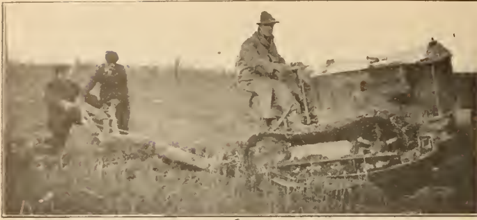
Plate No. 4a,—Underground Rural Transmission Lines. Tractor excavation trench for underground cable.
