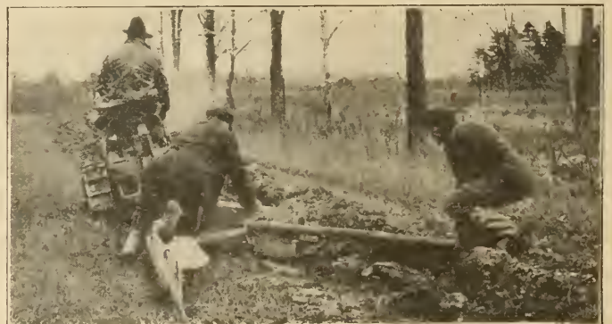
Plate No. 4c,—Underground Rural Transmission Lines. One method of re-filling trench after installing underground cable.
