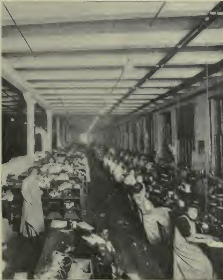
Fig. 3.—General illumination of a factory obtained from a double row of one-hundred-watt tungsten lamps, provided with special distributing reflectors and hung on short drops from the ceiling, as illustrated. Special steel reflectors, each provided with an eight-candle-power carbon lamp, direct the light at the machines.
