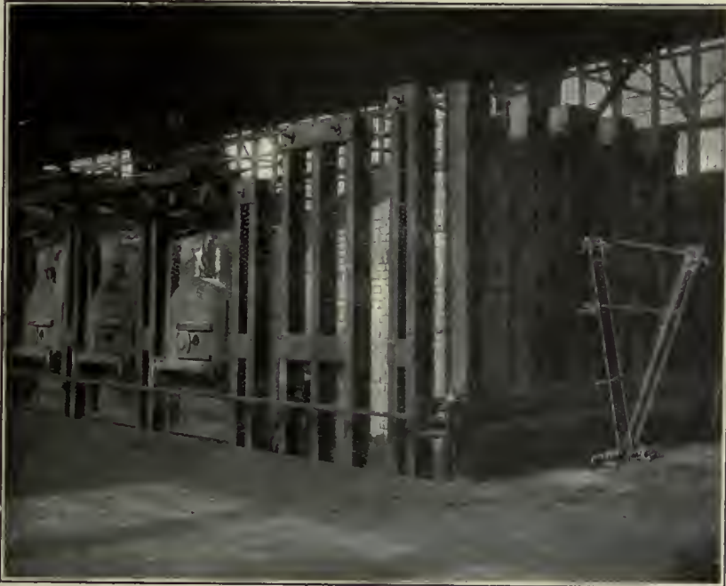
The Kirkwood Oil Fuel System as Applied to Open Hearth Furnaces.
