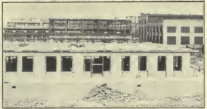
Fig. 2.—No. 2 of a Panoramic View Showing East End Stores with Pattern and Car Shops in Background.
