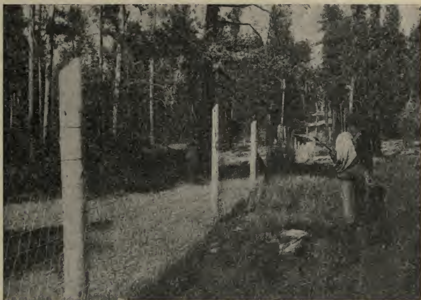
Coyote-proof fence erected by the United States Forest Service. Hunter and hound patrolling.
