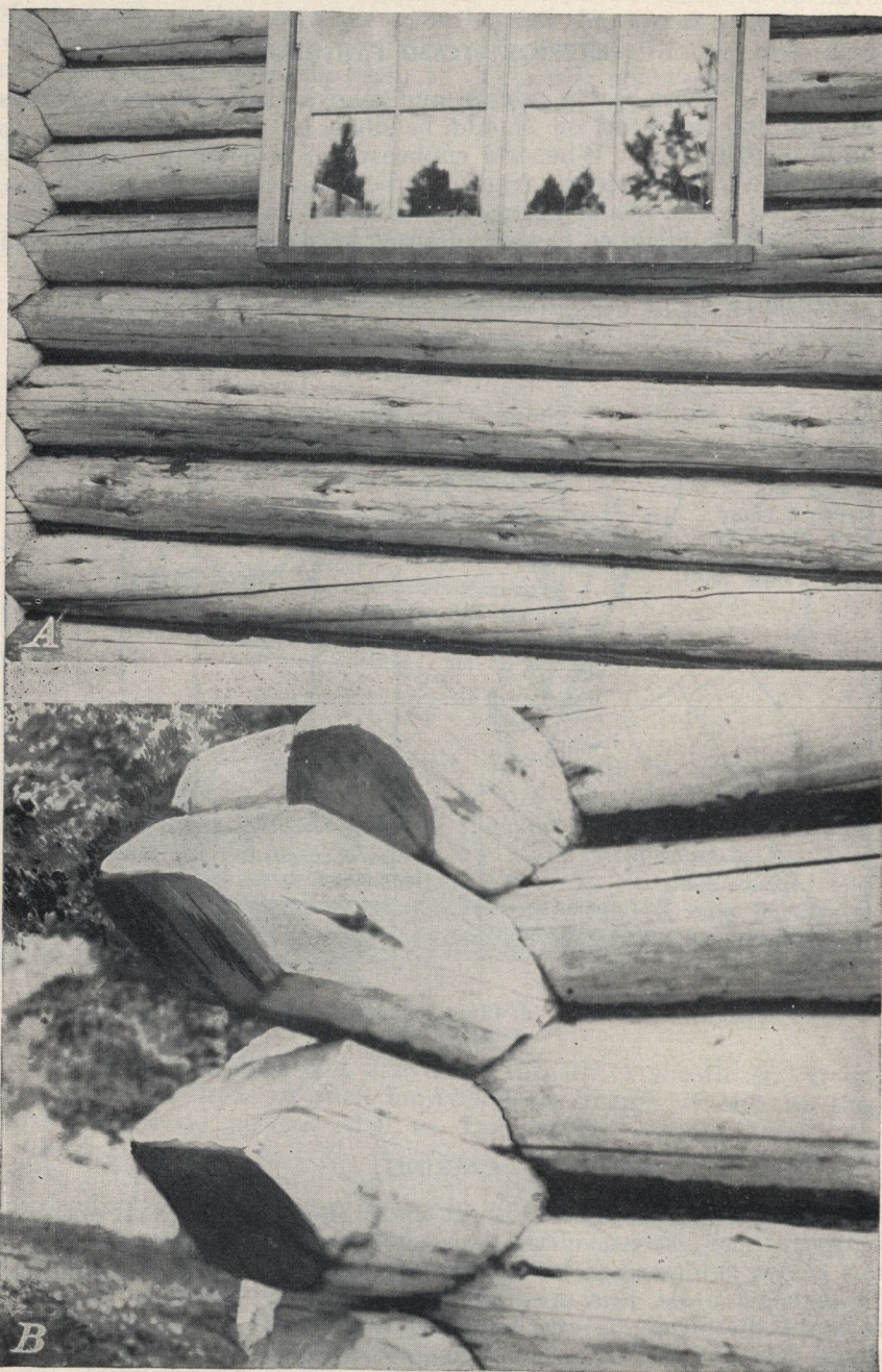
FIGURE 24.—Examples of tight joints well calked. A, Interior calking; B, exterior calking.
