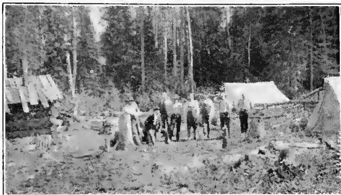
A Road-gang in the Clay Belt—Good bush roads are a prime necessity in early settlement.
