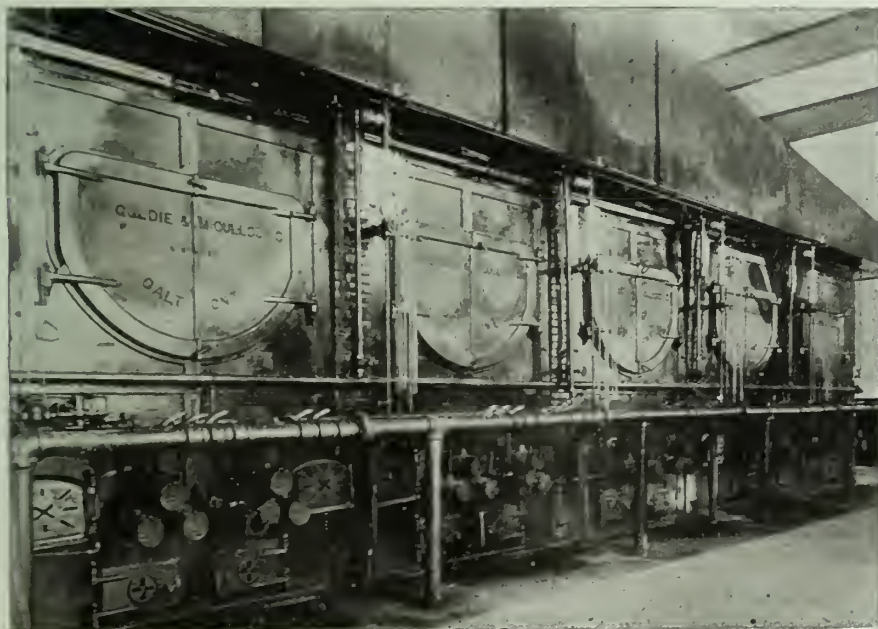
INSTALLATION OF GAS-FIRED BOILERS FOR SUPPLYING STEAM TO THE HAMMERS IN THE FORGE DEPARTMENT.
