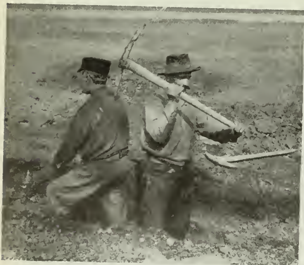
FIG. 27. EXCAVATION OR DITCHING, SHOWING LIABILITY TO SERIOUS ACCIDENT IF MEN WORK TOO CLOSE TOGETHER.
