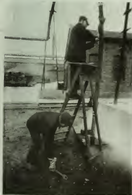
FIG. 33. WORKMAN PLACES WRENCH CARELESSLY ON LADDER PLATFORM.
