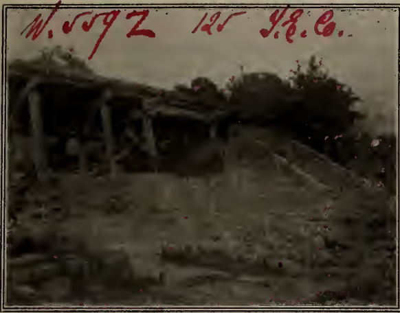
SIDE VIEW OF CULVERT AND WINGWALLS, L. E. AND D. R. RY.
