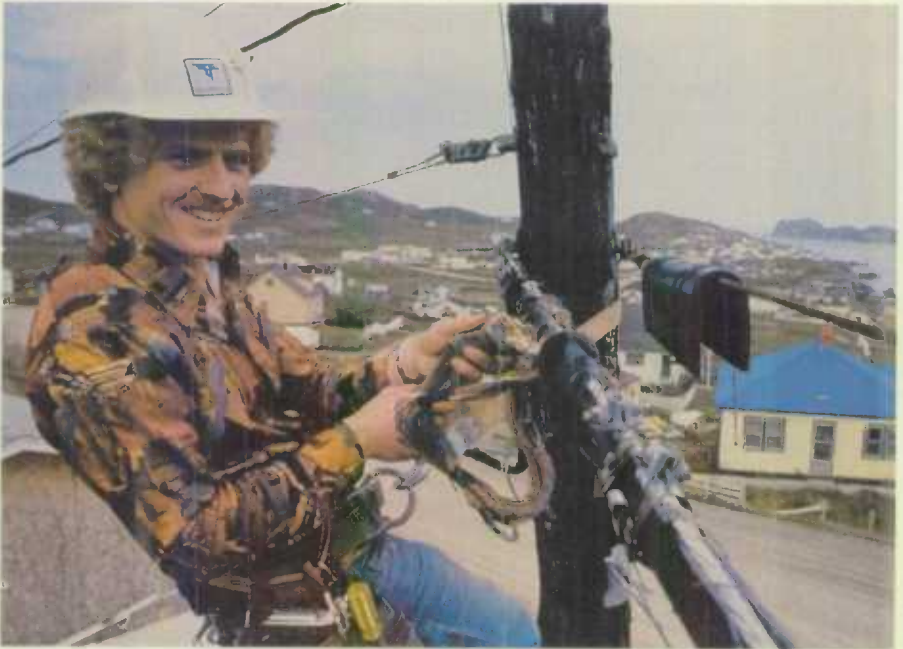
Maintenance of Newfoundland's Tanna Tel - a telephone system which is very important to people scattered widely and separated by rugged terrain.
