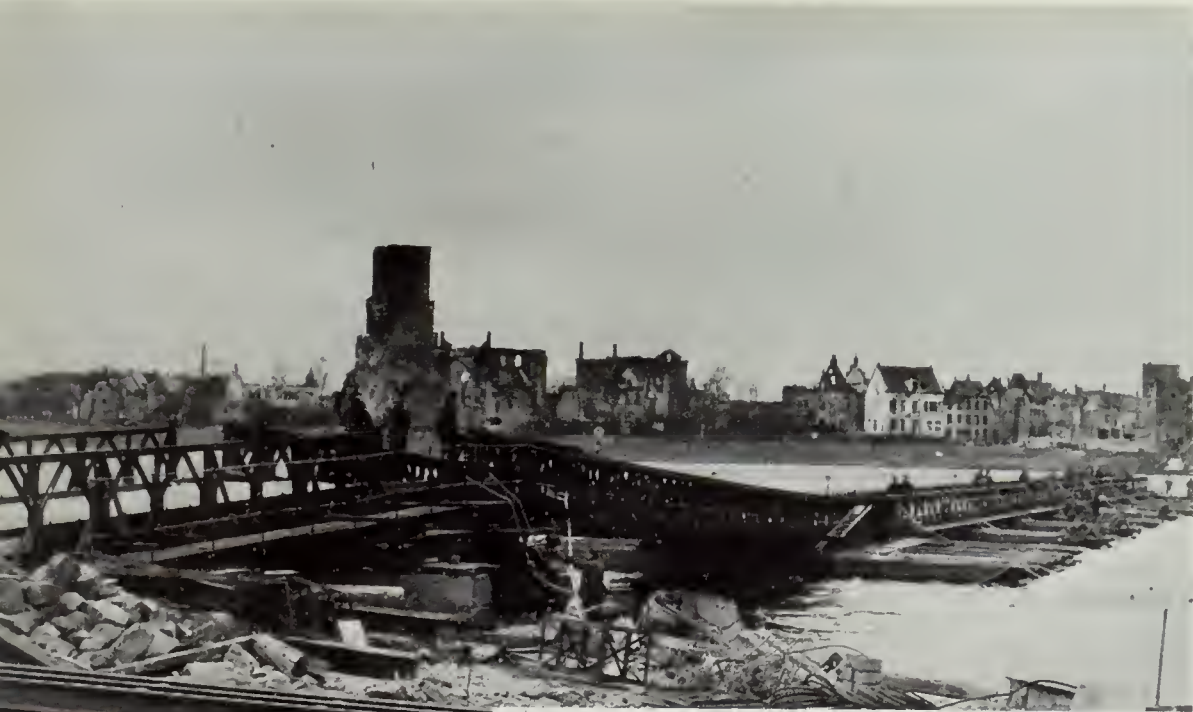
Left: "Melville" Bridge. This bridge across the Rhine at Emmerich, completed by the 2nd Canadian Army Troops Engineers on 1 April 1945, is shown under construction.
